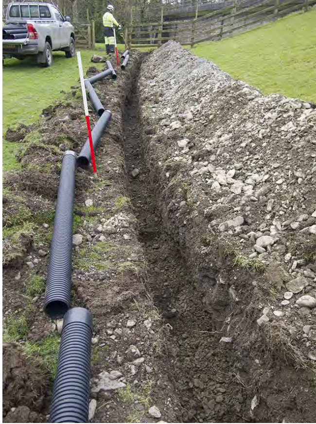
Photo 3: Looking west along the cable trench excavations on the approach to the westernmost field. 1m scale.
