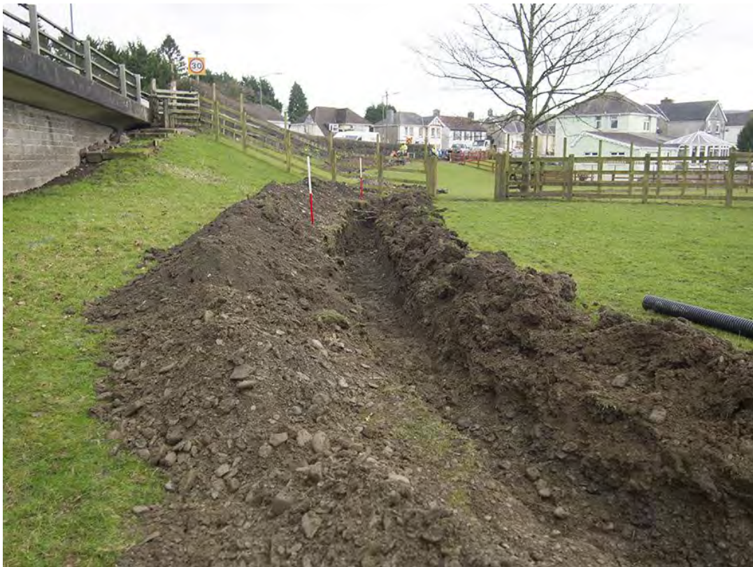
Photo 4: Looking east along the cable trench excavations in the westernmost field. 1m scale.
