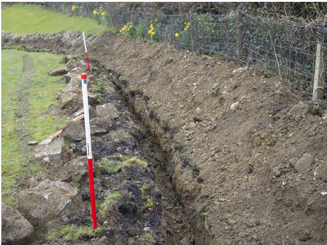
Photo 2: Looking northwest along the cable trench excavations in the easternmost field. Large stones from deposit 103 visible. 1m scale.
