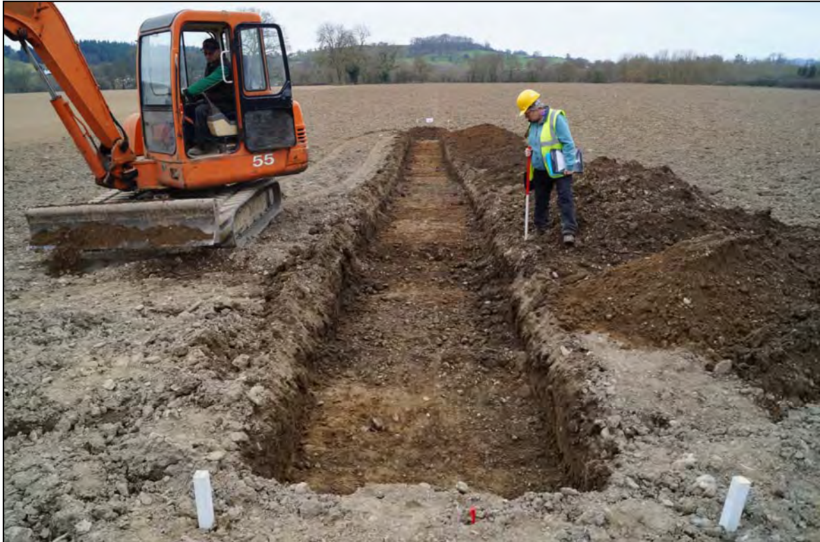
Plate 5: CCH2016_105. The excavated Trench 1, looking southwest. In the trench in the foreground is a waterworn cobble layer with clay beneath, different to the subsoil in other areas. This appears to be a natural band within the glacial subsoil.
