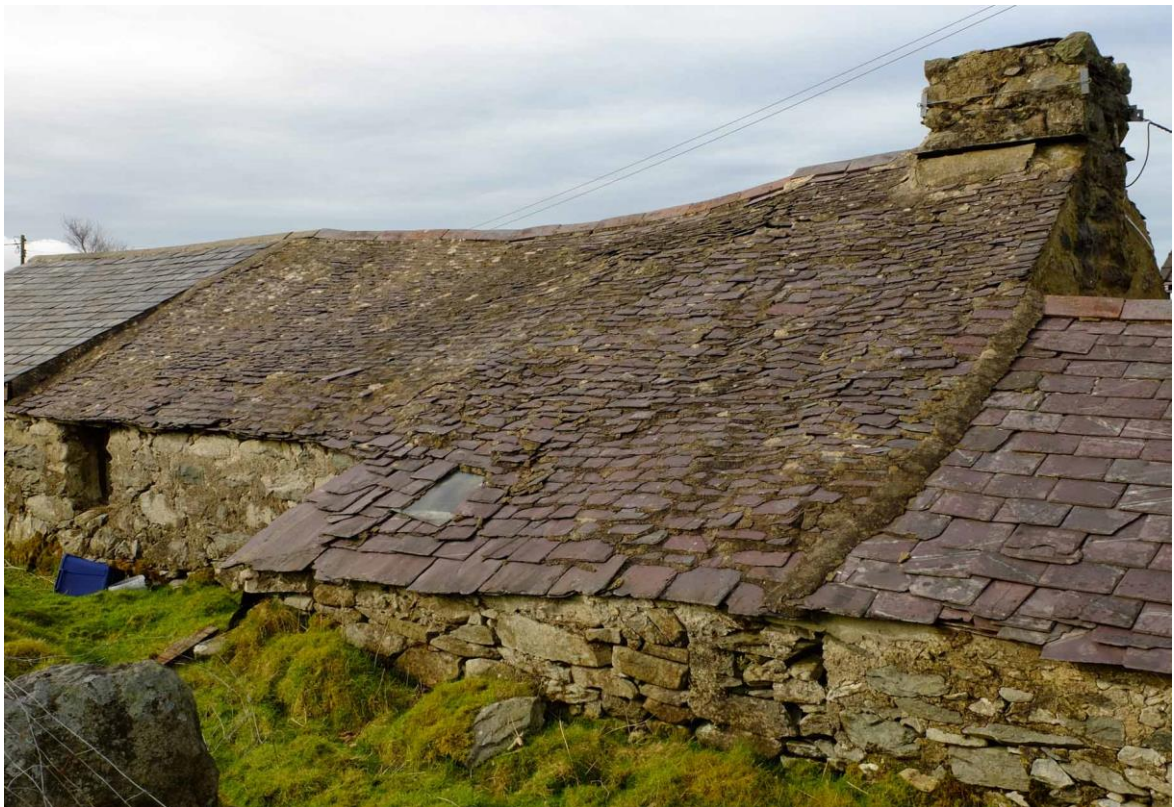
Fig 17 The old cottage at Bryn Tirion in Cilgwyn has a roof of generally poor-quality small slates, maintained by grouting.
