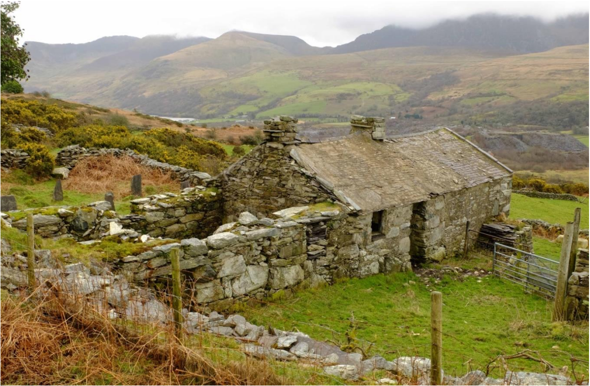
Fig 10 Pen-hafod-las in Cilgwyn. The house is roofless but has an additional heated unit and farm range in line with the cottage.
