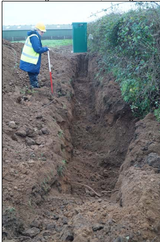
Plate10: MYW2015_110, excavating cable trench along hedgerow from cabinet in eastern field, looking south southeast
