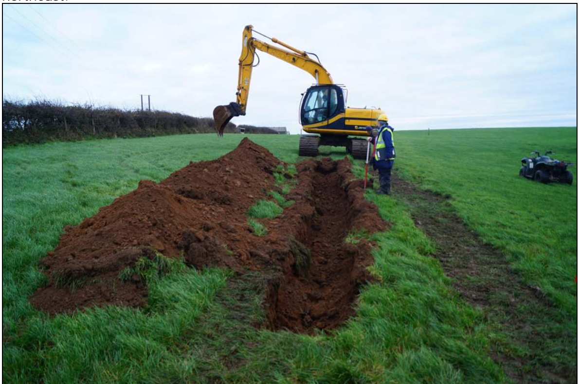
Plate 12: MYW2015_112, excavating the cable trench in the western field, looking south southeast
