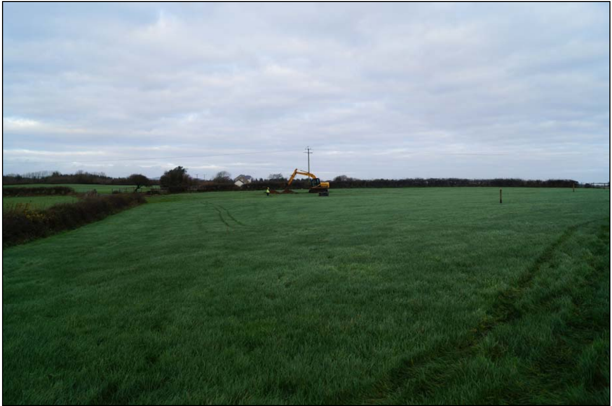
Plate 11: MYW2015_111, starting excavation of the cable trench in the western field , taken from the western side of the area of the solar array, looking northeast.
