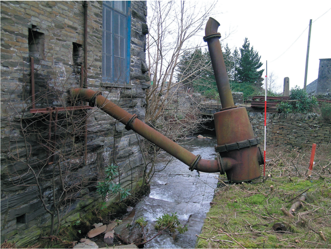
Plate 17 Site 3(1) Hydroelectric power station: Iron vessel
