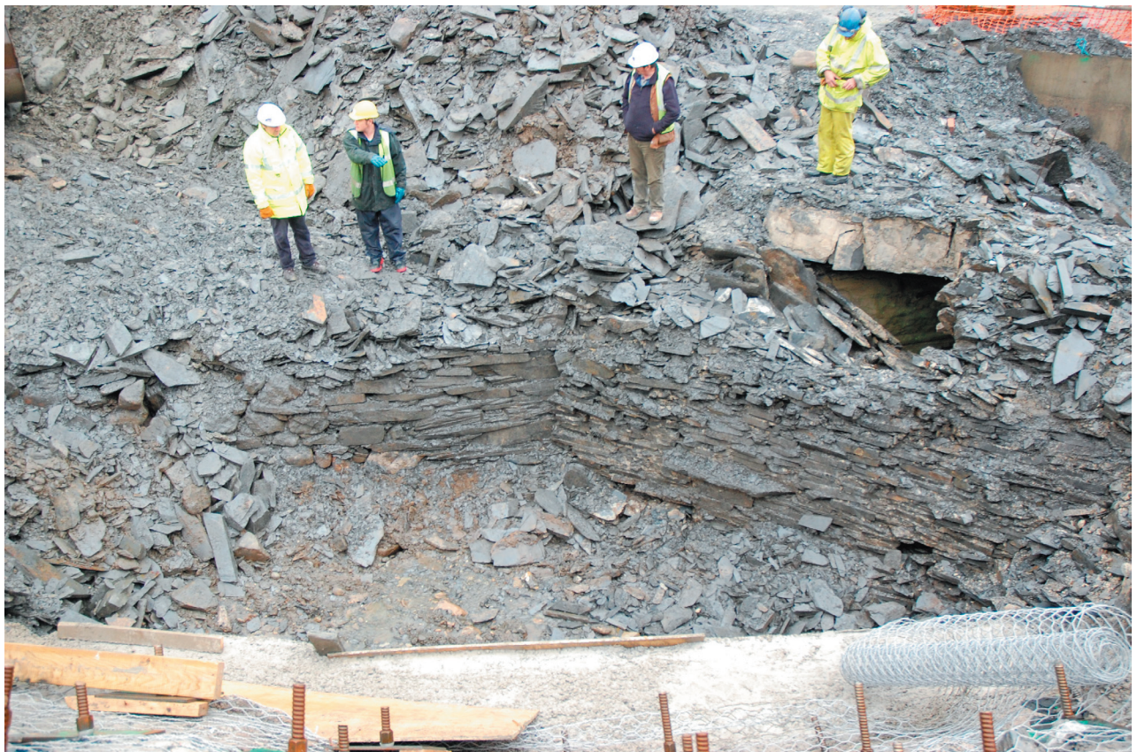
Plate 16 Site 3(3) Road causeway: Phase 1 revetment to the east of the incline tunnel
