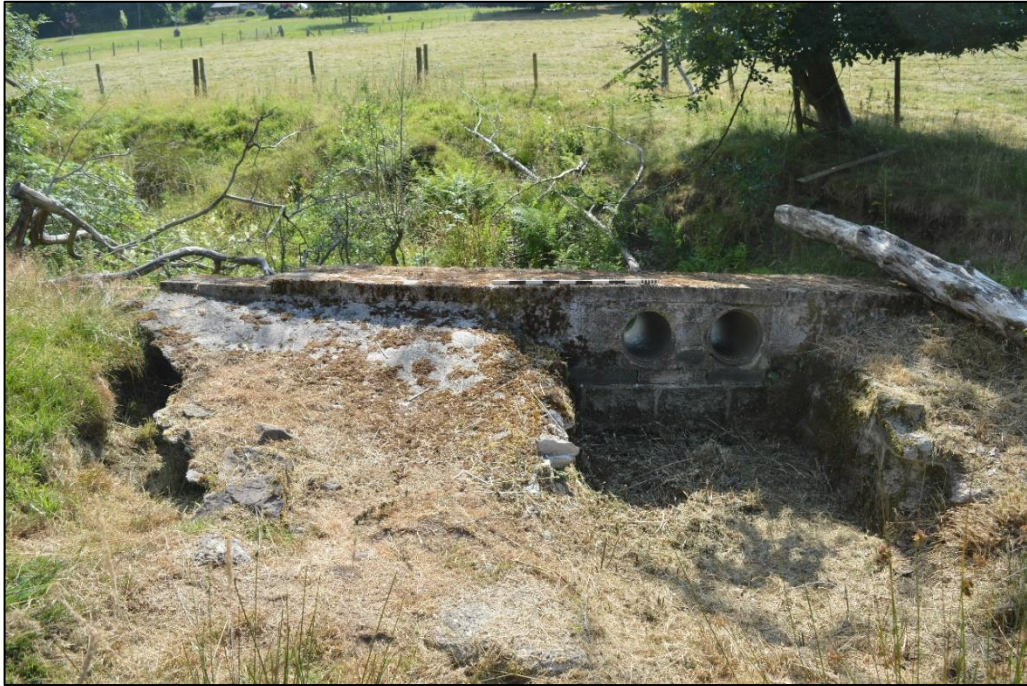
Fig. 15 View from the north-west of the southern overflow showing the erosion of the dam construction on the north-east end. Photo CPAT 4523-0015
