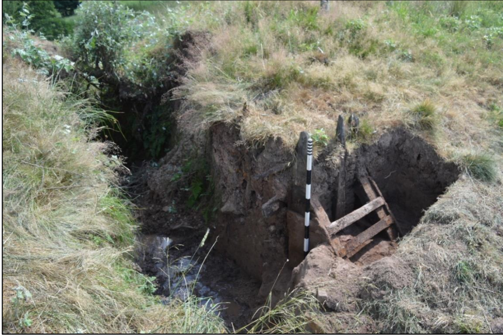
Fig. 12 View from the north-west of the breach and the wooden bank retaining structure south of the sluice. Photo CPAT 4523-0021
