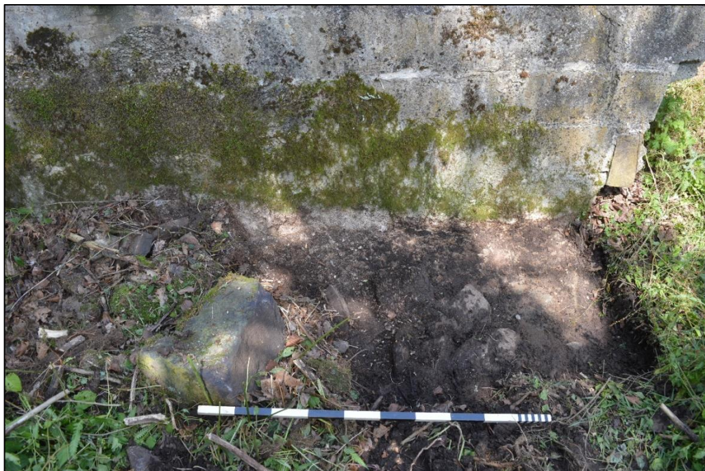
Fig. 16 Stonework in the outlet channel south of the southern channel. Photo CPAT 4523-0013
