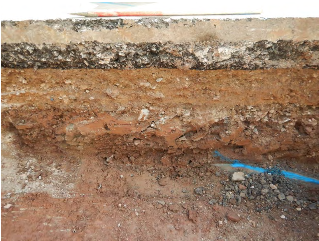
Photo 7: View south of section along Lodge Road (Phase 1), showing marked water pipe (008) and overlying modern deposits. 1m scale.
