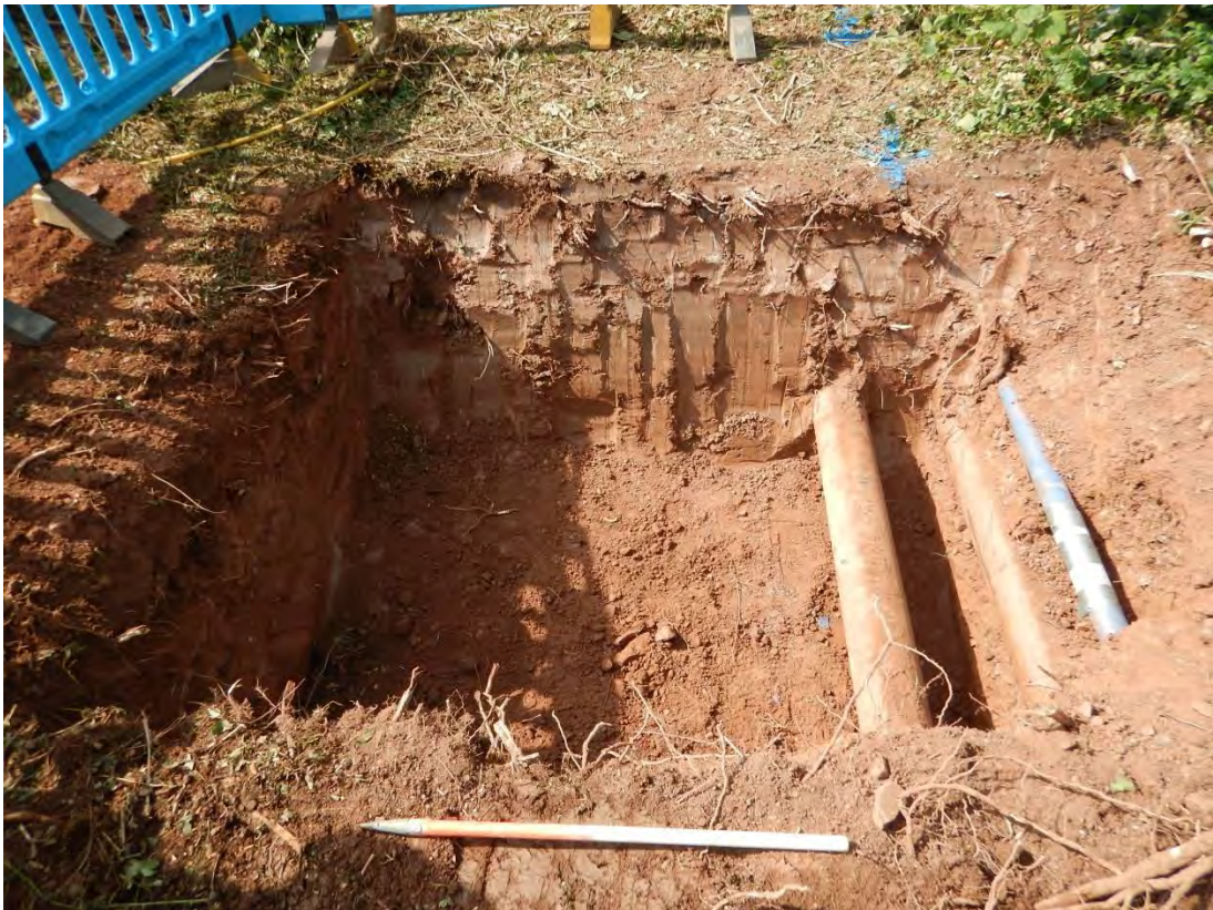
Photo 14: View southwest of the excavations adjacent to the reservoir (Phase 2), Trench 4. Showing deposits (026) and (027), cut by modern services. 1m scale.
