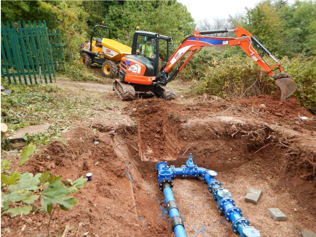
Photo 13: View northeast of the excavations adjacent to the reservoir (Phase 2), Trench 3. Showing deposits (026) and (027).
