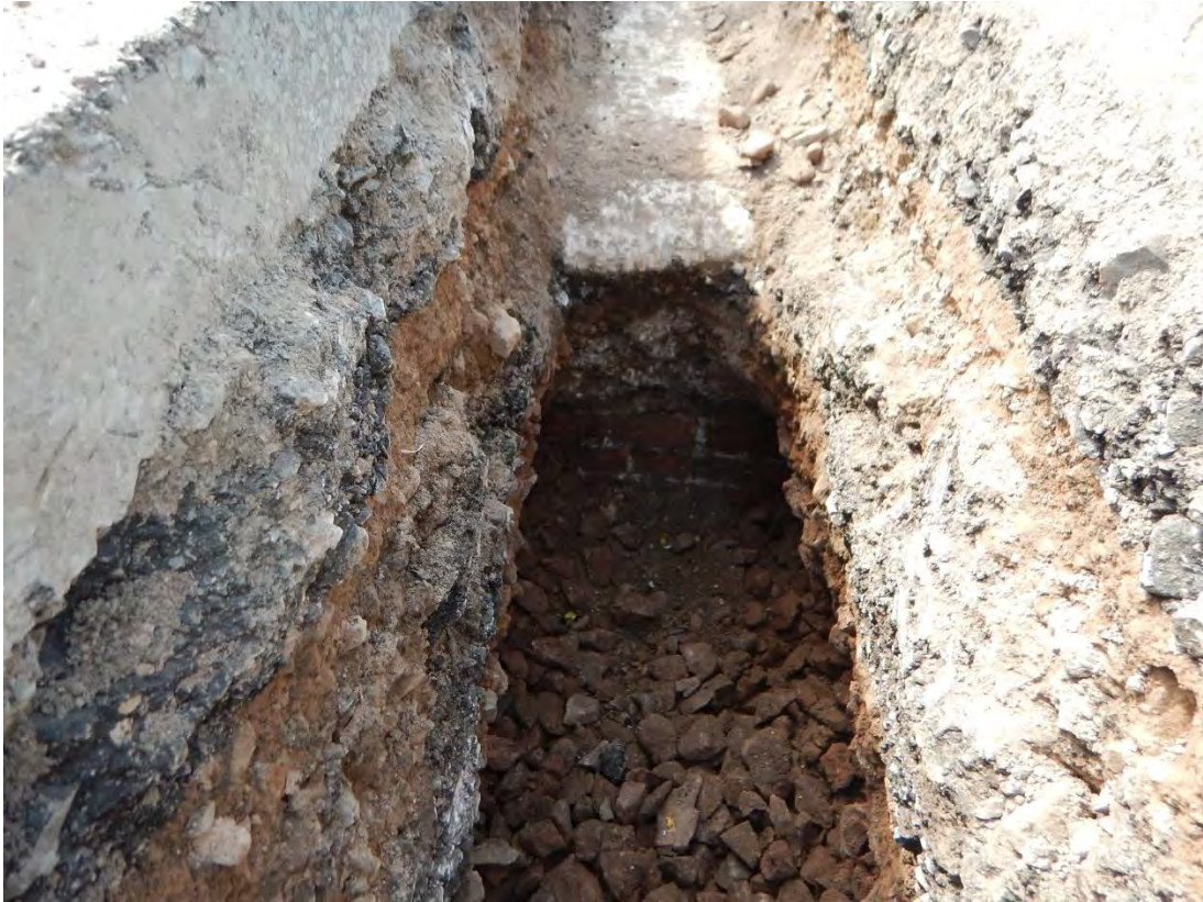
Photo 9: View west of Lodge Road (Phase 1) excavations, showing brick feature {017} and concrete capping {016}.
