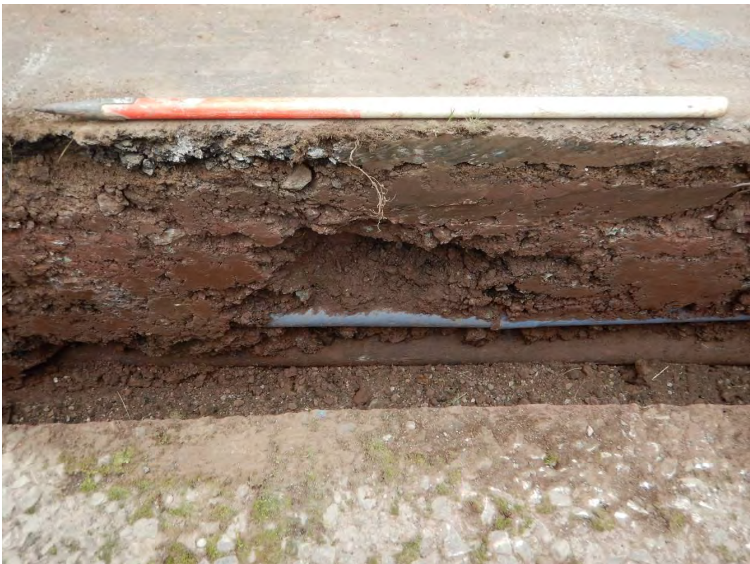
Photo 18: View west of the excavations along the reservoir access track excavations (Phase 2), Trench . Showing deposits (030) to (034). 1m scale.
