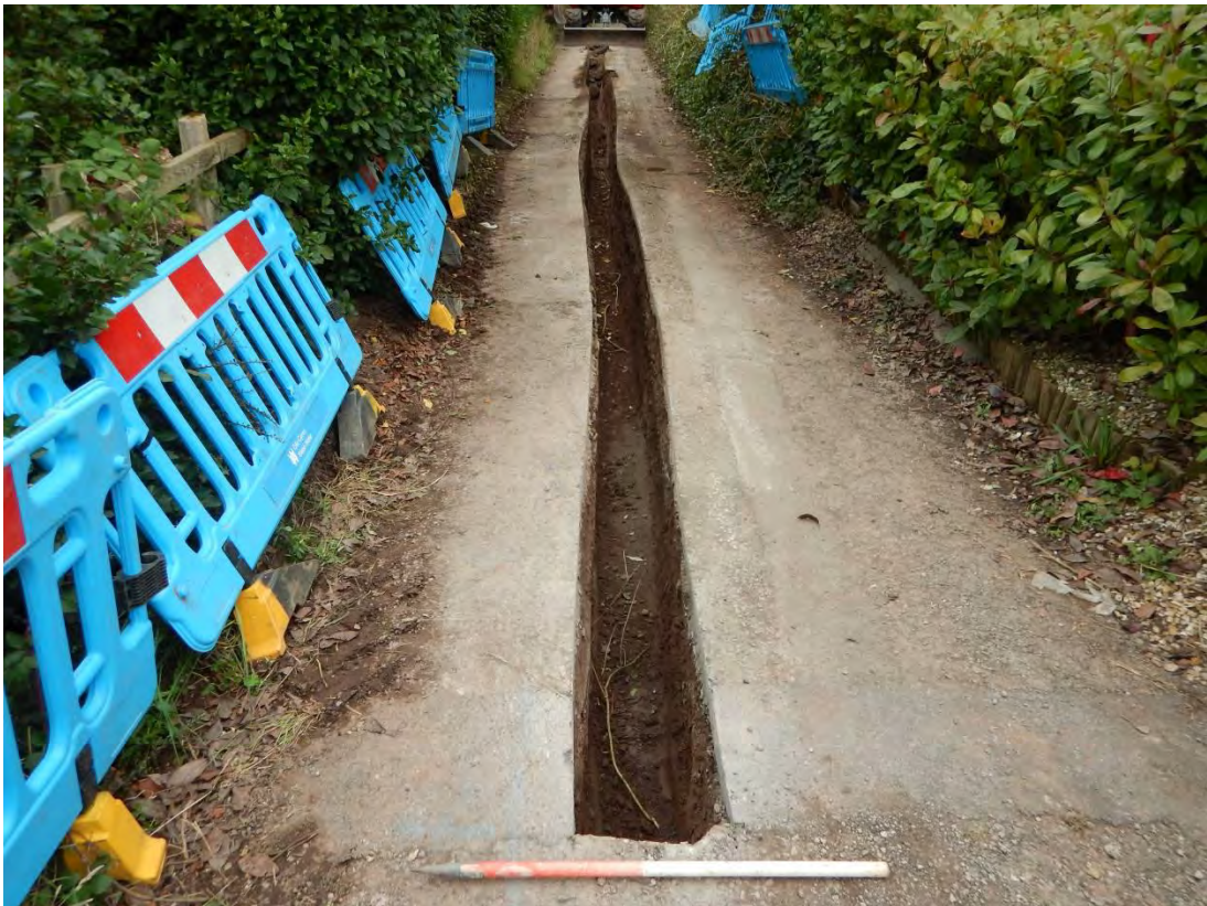
Photo 12: View northwest along the reservoir access track excavations (Phase 2), Trench 5. 1m scale.
