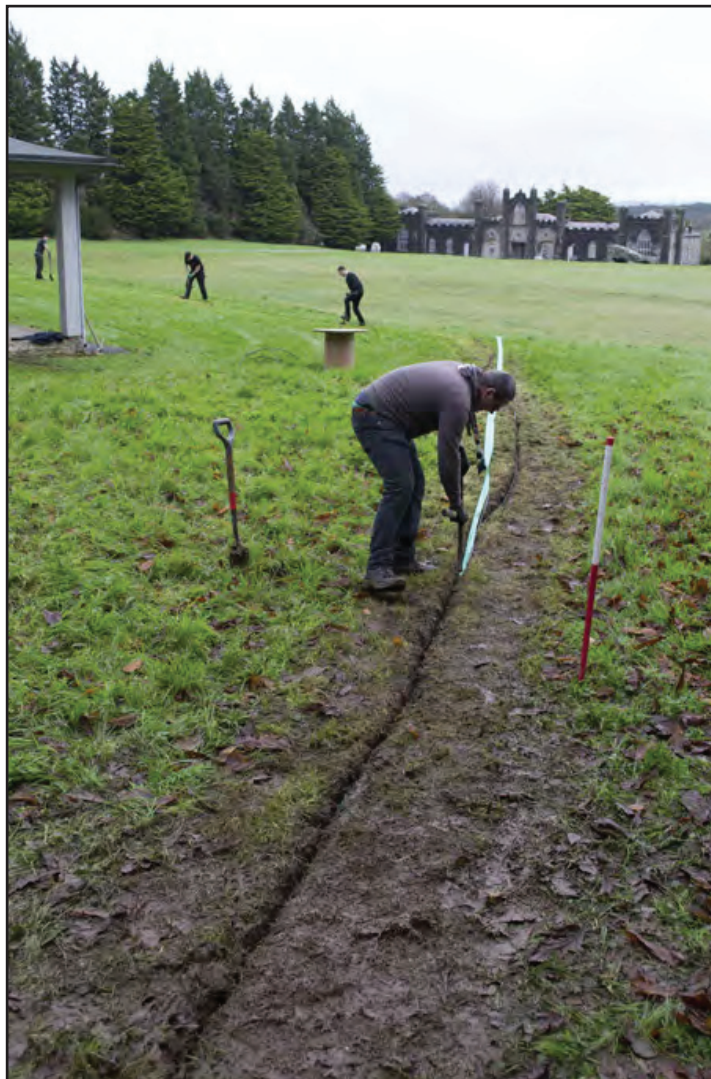
Plate 6: General shot from the east of pavilion, showing cable trench hand excavation in progress; scale: 1x1m (archive reference: G2542_016).
