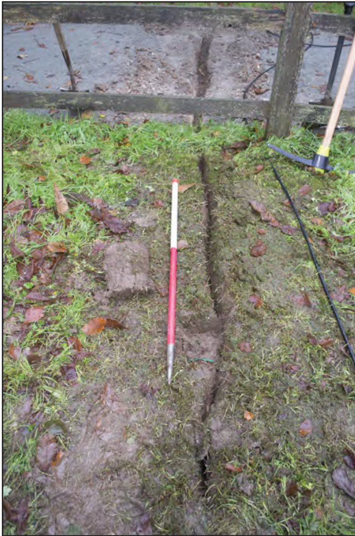
Plate 2: Detail showing cable trench near western end; scale: 1x1m (archive reference: G2542_003).
