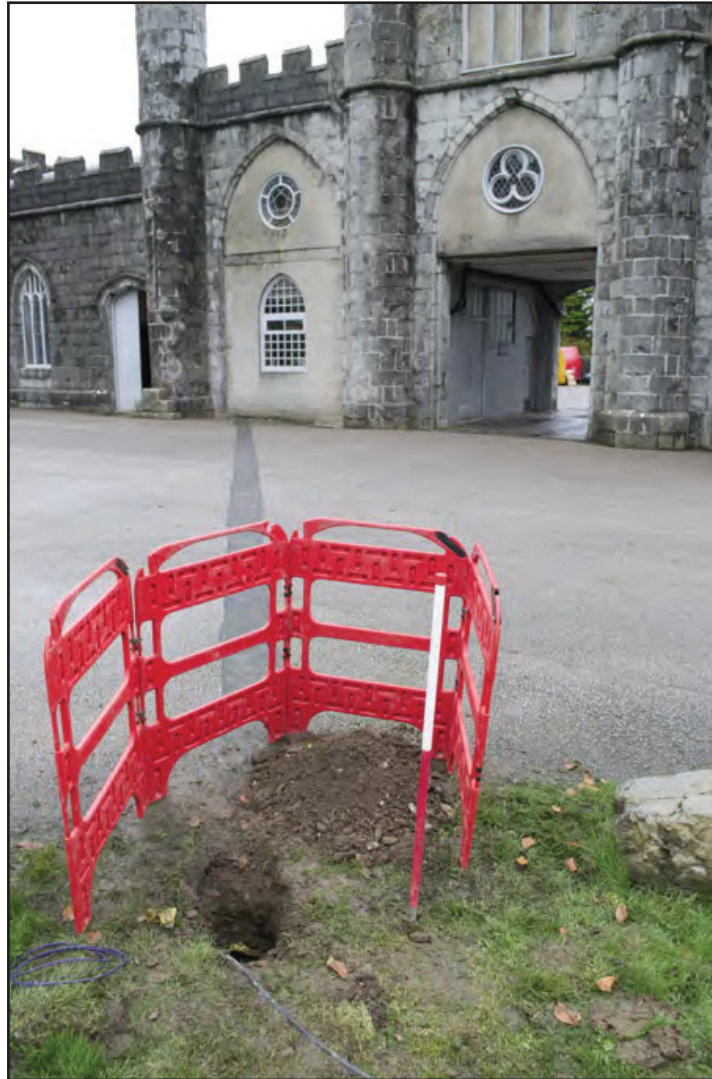
Plate 13: Service duct at eastern end of trench excavation near the stables, adjacent to macadam drive; scale: 1x1m (archive reference: G2542_031).
