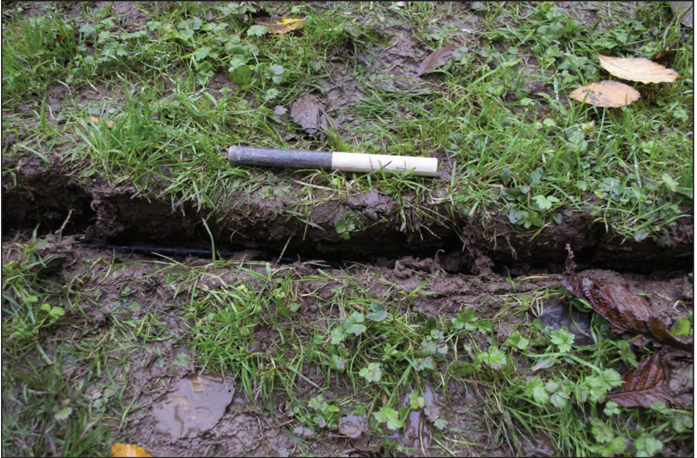
Plate 7: View of 'section' of cable trench through topsoil, with cable in place; scale: 1x0.2m (archive reference: G2542_015).
