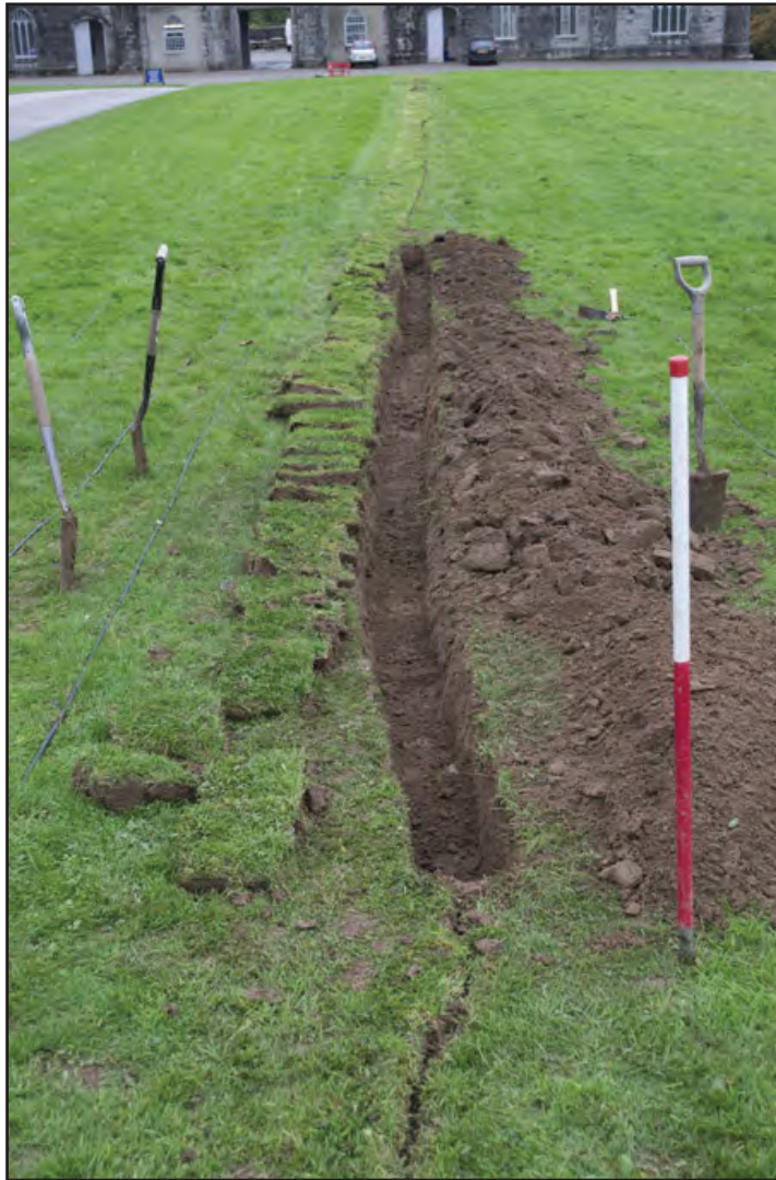
Plate 11: View of 10m long trench section after excavation; scale: 1x1m; 1x0.2m (archive reference: G2542_029).
