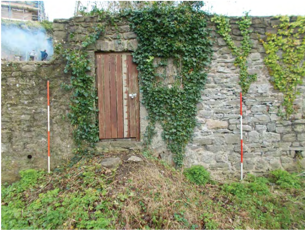
Plate 17: View north east toward south external wall, showing transition from medieval wall to the right (medieval arrow loop visible in bottom right), to 18th/19th century wall to left of ivy.
