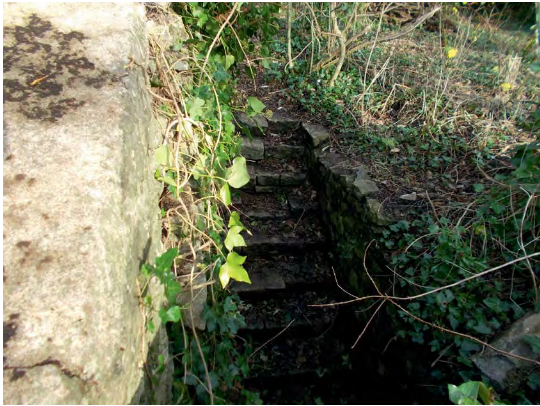
Plate 23: Stairs built in the adjacent property to the east, built against the burgage plot boundary wall, illustrated as a comparison to the stairs revealed in the north west buttress wall
