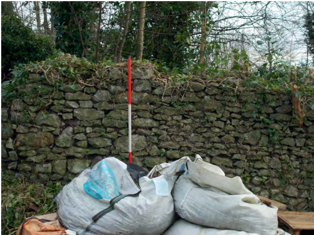
Plate 48: View south east toward east wall, showing detail of possible rebuilt section
