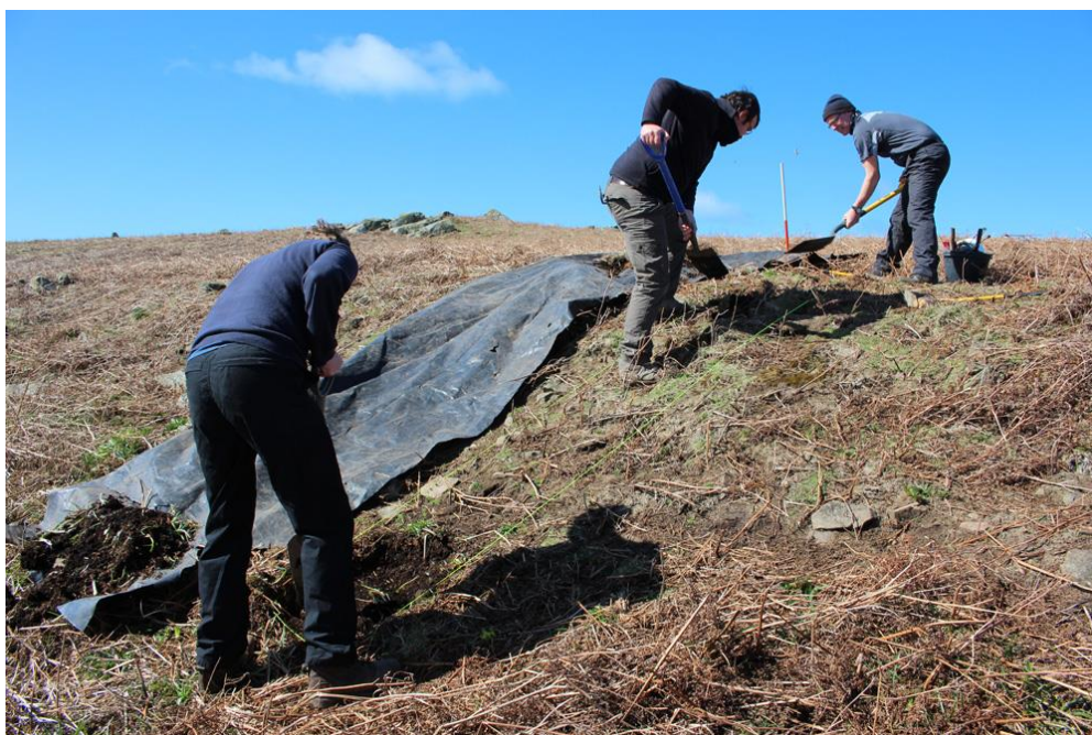
Figure 5. Initial work in progress at the trench, 30 th March 2016, with plastic laid down to contain spoil and prevent damage to surrounding ground surface. View from south-east (DS2016_078_005)
