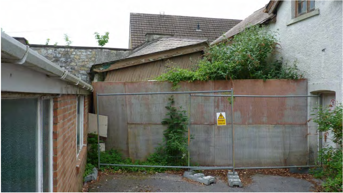
Photo 19: View west of collapsing structure adjoining the coach house.
