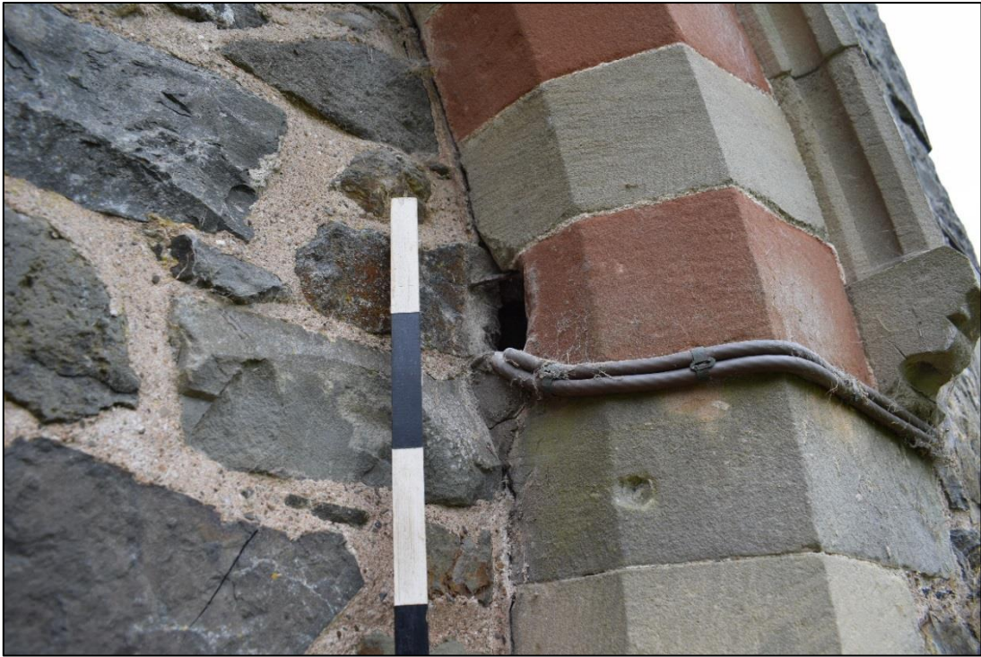
Fig. 6: The existing aperture in the blocked doorway, which was reused for the path lighting cable
