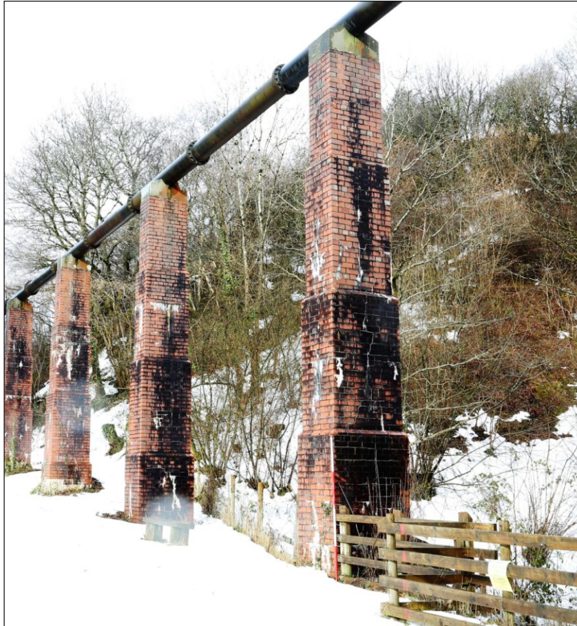
Plate 7: East end tall piers with four stage stepped profile, viewed from south-east. Scale 2m
