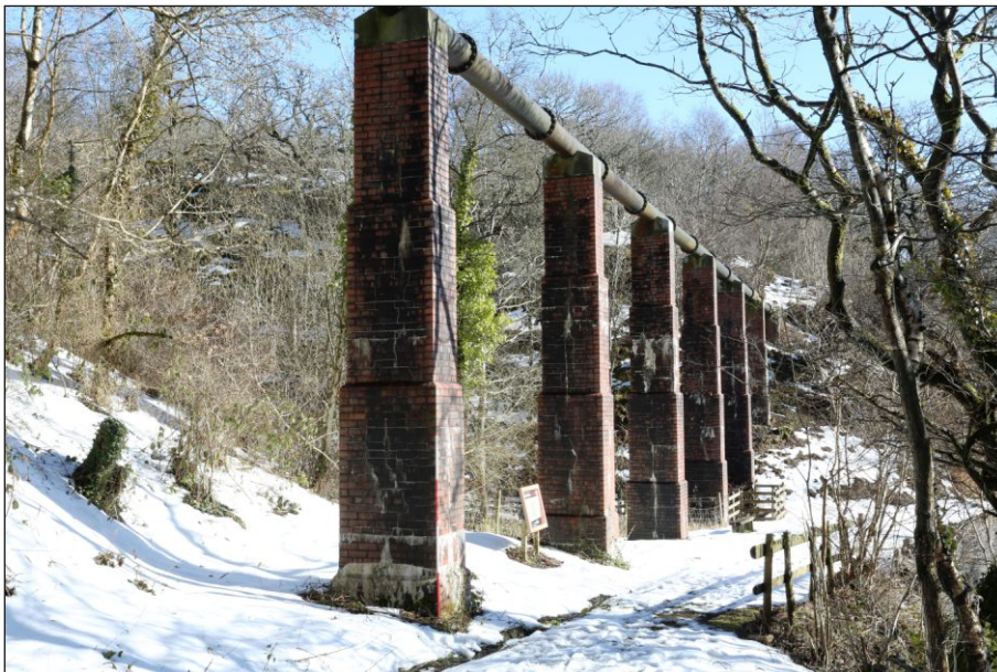
Plate 4: Pipeline on tall piers crossing Hafod Arch, viewed from west. Scale 2m
