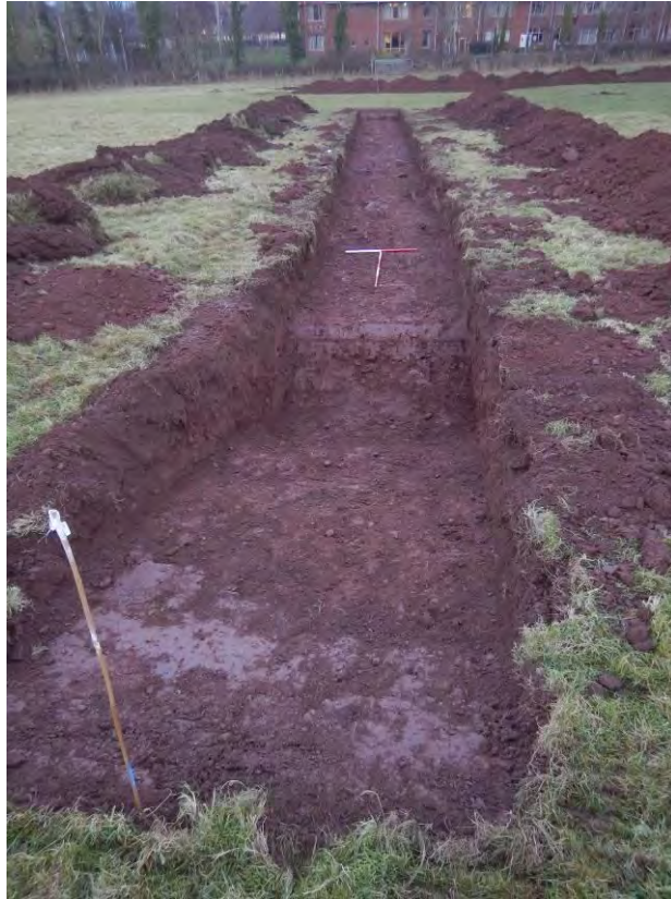
Photo 9: Trench 4, post-excavation, facing northwest. A machine excavated sondage is visible in the foreground to investigate natural deposits. 1m & 2m scale.
