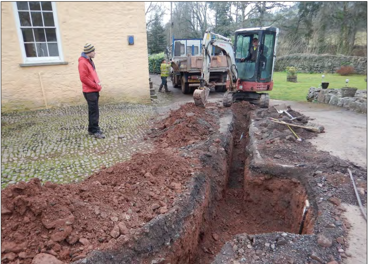
Plate 4: General shot showing excavation of the trench to the west of Abercamlais house, looking north-west.
