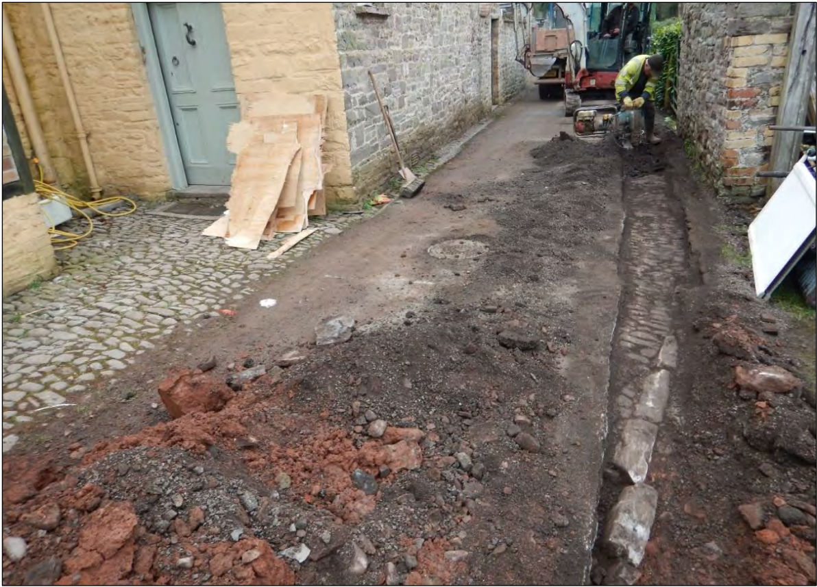
Plate 7: Working shot showing removal of tarmac road (004) to expose cobbled surface (019) to the north of Abercamlais House, looking west.
