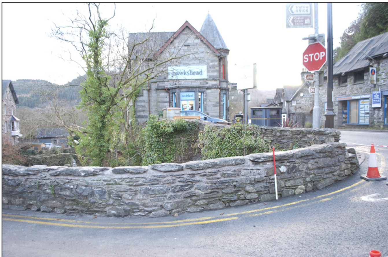
Plate 15: View of repaired southeast corner of the bridge parapet; scale: 1x1m (archive reference: G2587_033).
