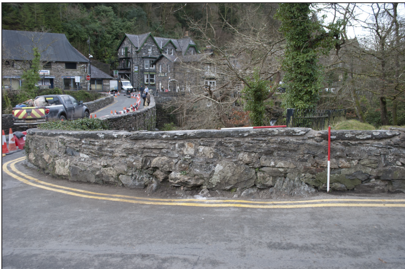
Plate 18: View of the carriageway side of the northwest parapet repair work; scale: 2x1m (archive reference: G2587_041).
