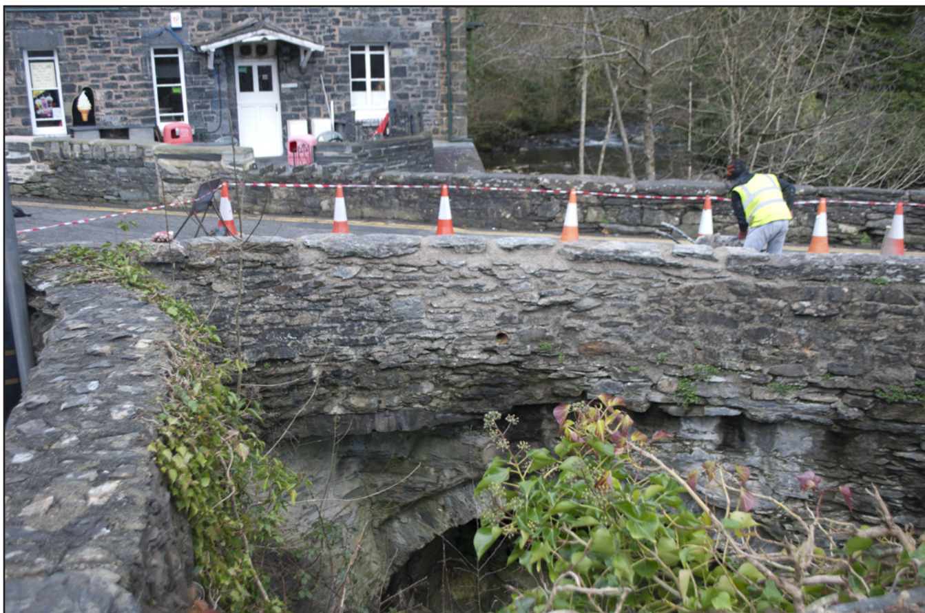
Plate 14: View of completed work to the southeast portion of the parapet from the riverside; scale: not used (archive reference: G2587_030).
