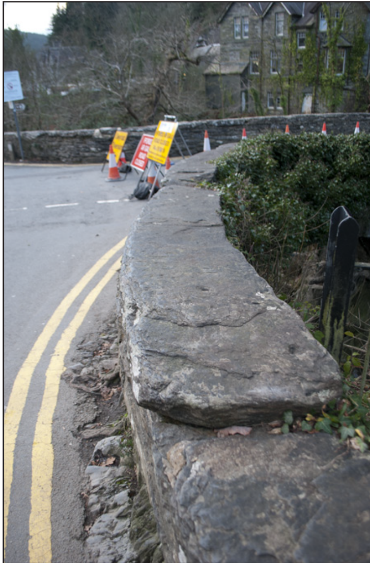
Plate 9: Detail of very large (3.2m long by 0.1m high) slipped coping stone; scale: not used (archive reference: G2587_017).
