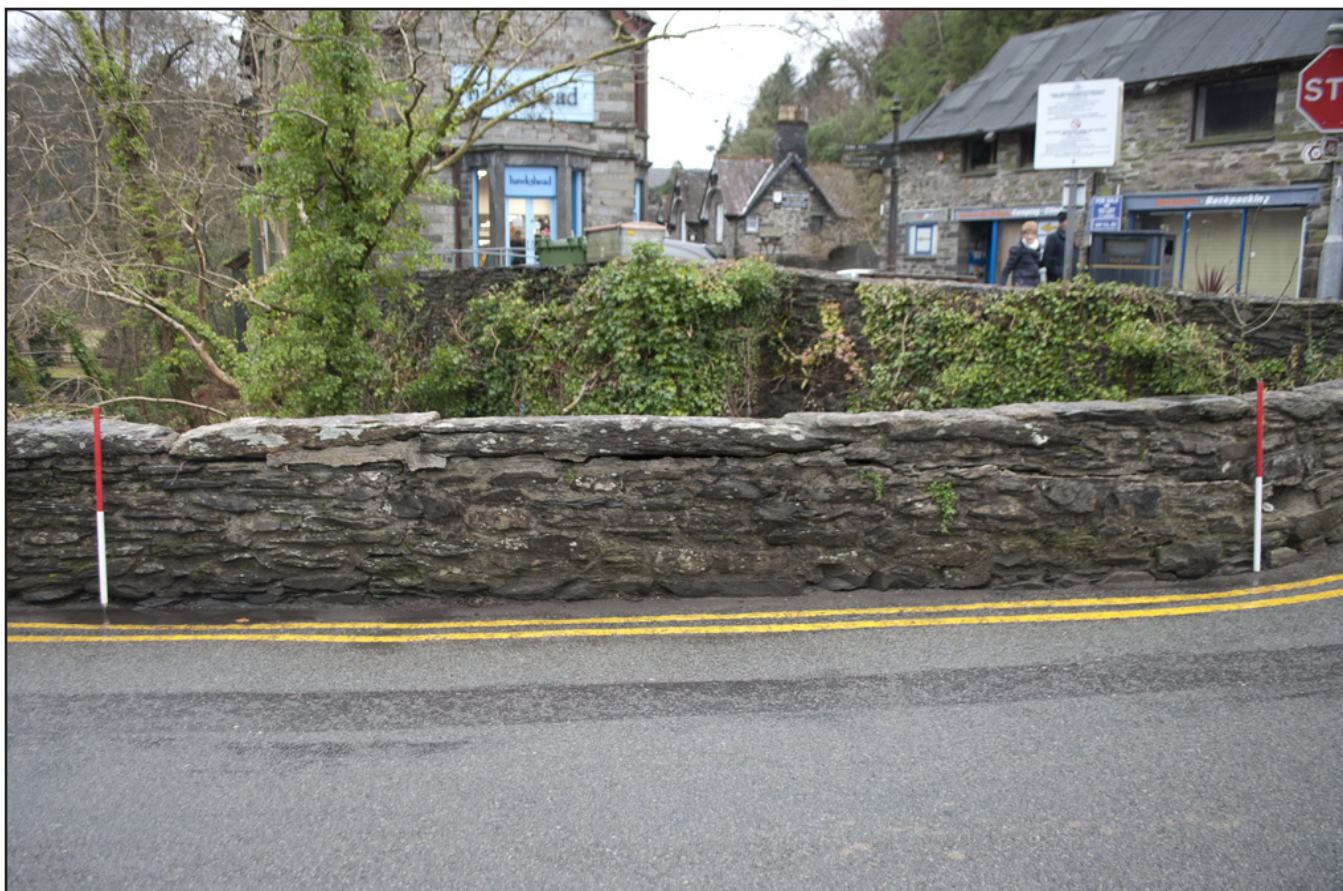
Plate 2: General view of damaged section of walling at southeast corner of Pont y Pair; scale: 2x1m (archive reference: G2587_003).
