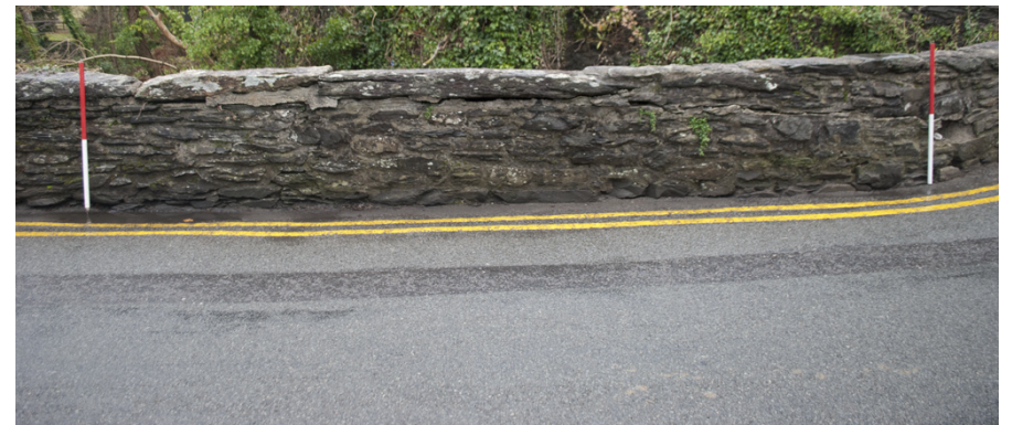
Figure 02: Southeast facing elevation of Pont-y-Pair Bridge detailing damage and existing repair. Scale as shown
