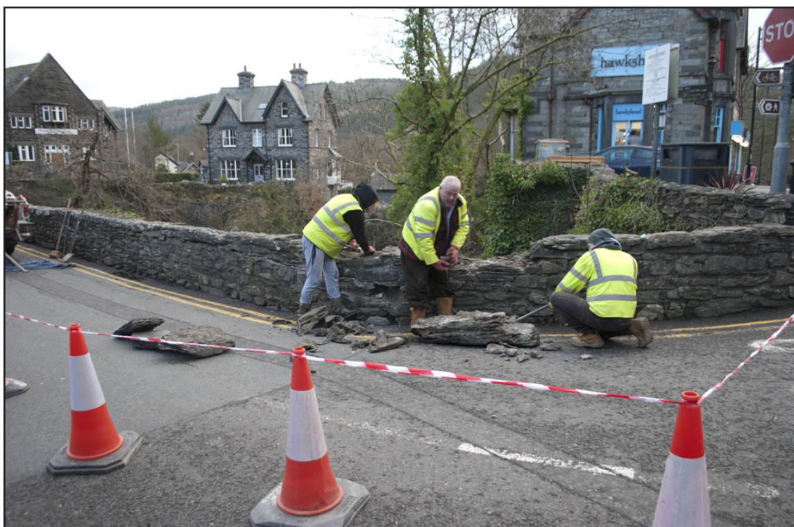
Plate 10: Action shot showing demolition work (by hand) taking place at the southeast corner of the parapet; scale: not used (archive reference: G2587_020).
