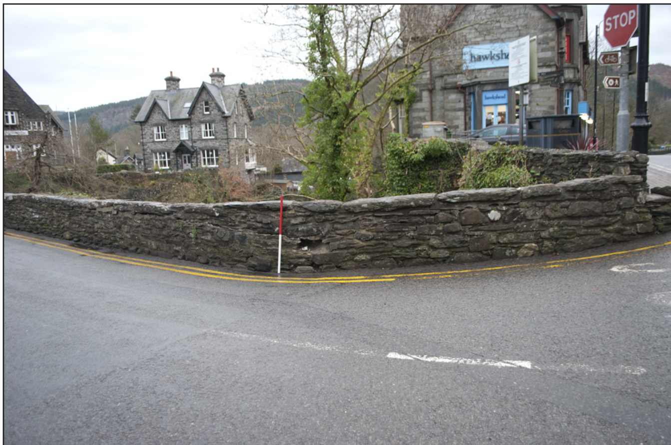
Plate 3: General view of damaged section of walling at southeast corner of Pont y Pair showing the splaying parapet from the A5 junction; scale: 2x1m (archive reference: G2587_004).
