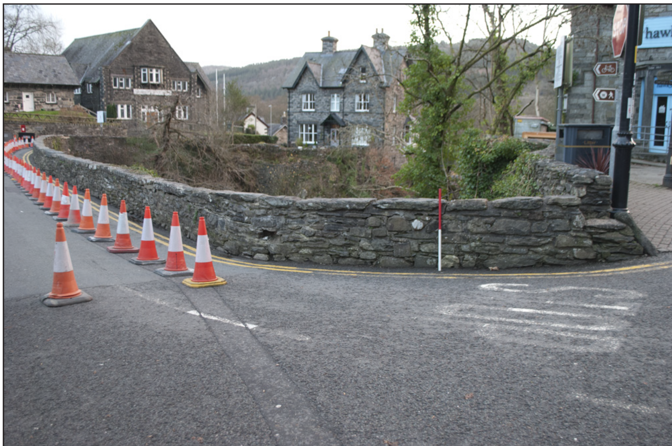
Plate 7: View of damage on splayed corner of the parapet walling to the southeast near junction with the A5 road; scale:1x1m (archive reference: G2587_012).
