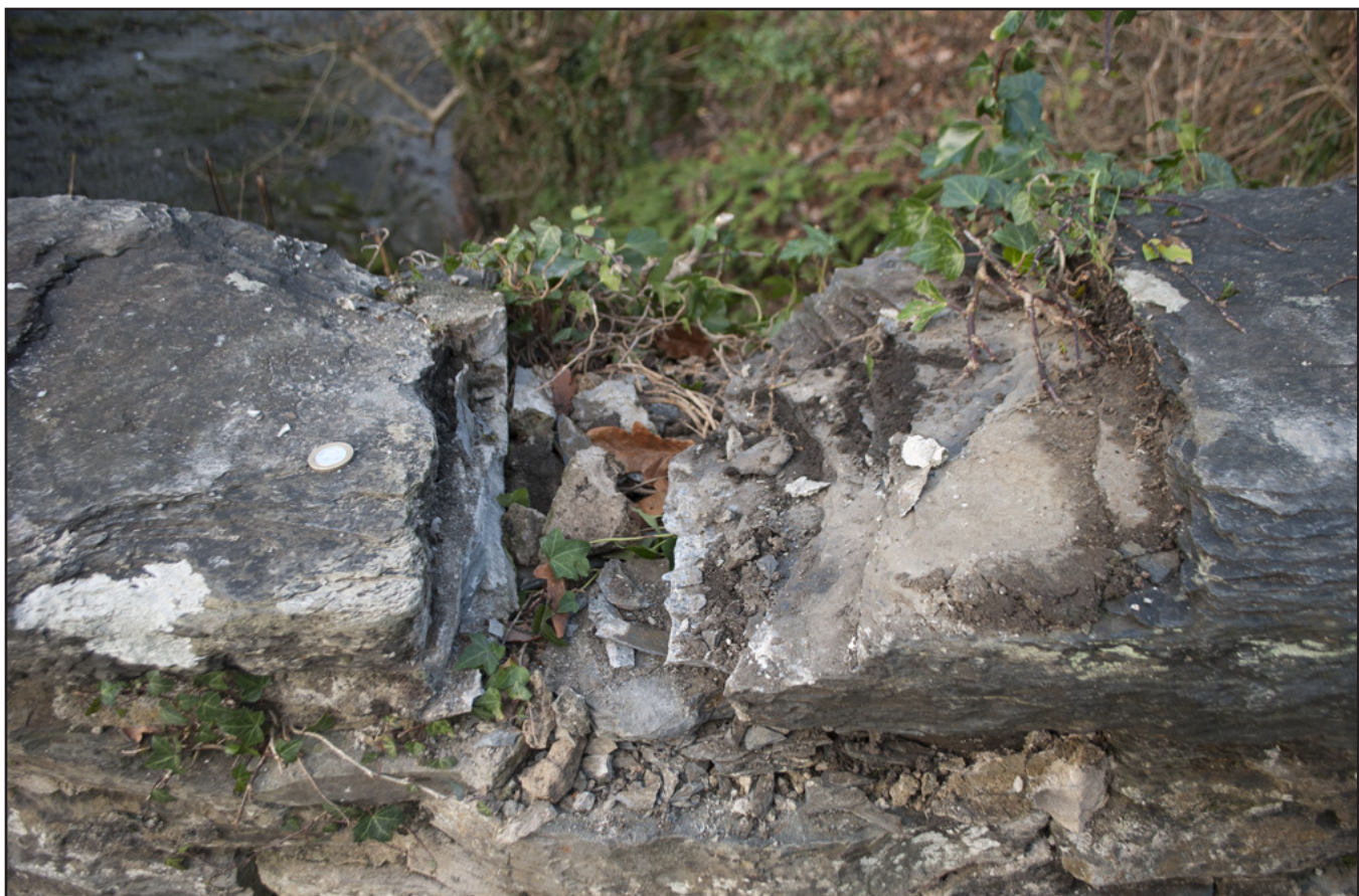
Plate 16: Area of damaged coping at the northwest end of the parapet; scale: not used (archive reference: G2587_034).
