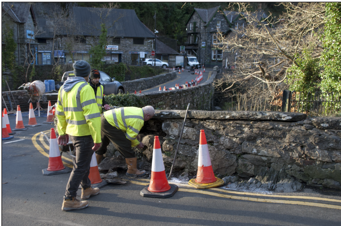
Plate 17: General shot of repair work to stones below the large coping stone at the northwestern end of the parapet; scale: not used (archive reference: G2587_037).
