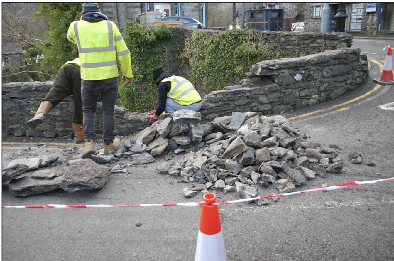
Plate 11: General view during wall demolition showing the hard mortar (in a pile); scale: not used (archive reference: G2587_023).
