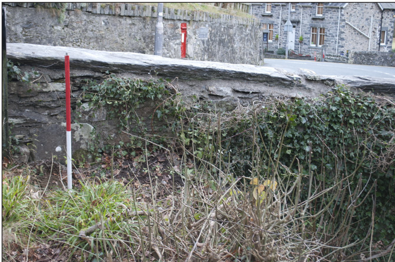
Plate 19: View of riverward side of the repaired northwest section of Pont y Pair parapet; scale: 1x1m (archive reference: G2587_039).
