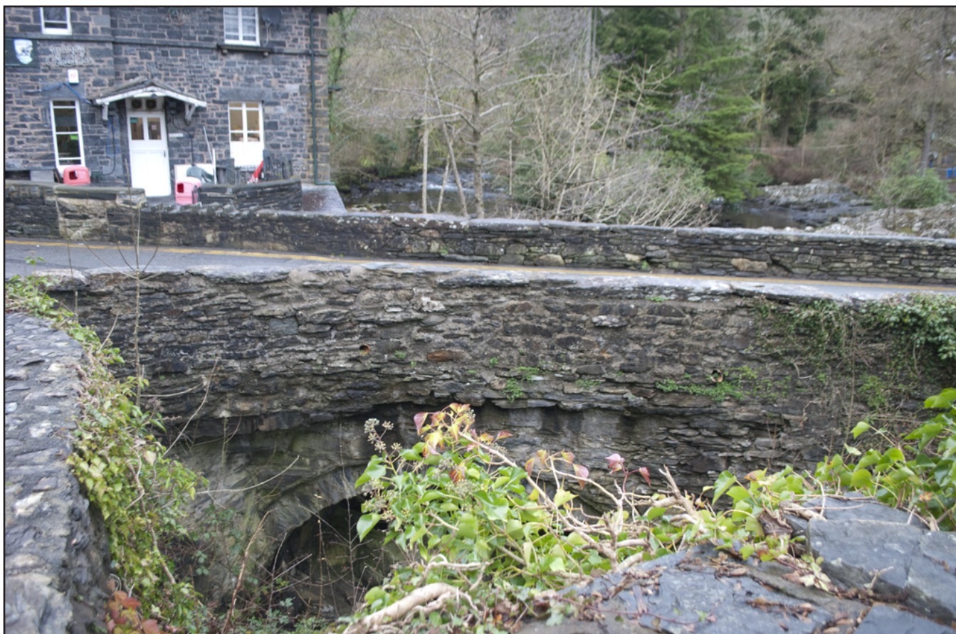
Plate 6: General view of damaged section of parapet wall; scale: not used (archive reference: G2587_005).
