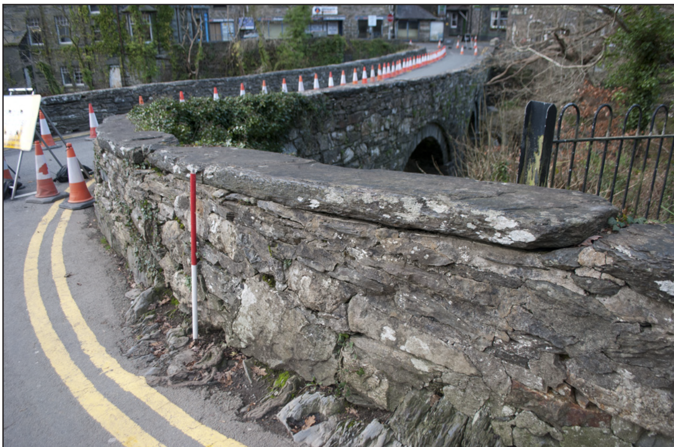
Plate 8: View of slipped coping stone at the northwest corner of the bridge parapet walling; scale: 1x1m (archive reference: G2587_016).
