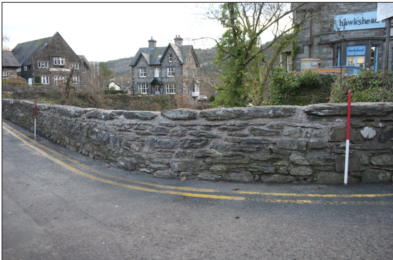
Plate 13: View of repaired southeast corner of the bridge parapet; scale: 2x1m (archive reference: G2587_031).
