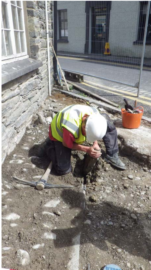
Plate 24: CHN2014_123: Removal by hand of part of 005, the edging of cobble pavement 007, prior to mechanical excavation of foundation trench, looking east northeast.
