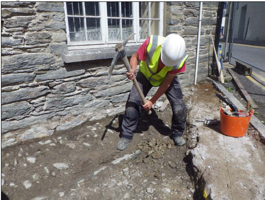
Plate 23: CHN2014_122: Removal by hand of part of 005, the edging of cobble pavement 007, prior to mechanical excavation of foundation trench, looking northeast.
