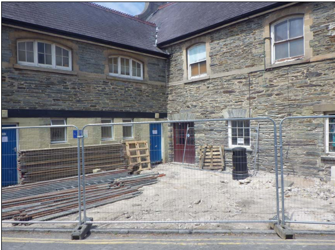
Plate 3: CHN2014_102: The rear of Cawdor Hall, after the removal of the paving slabs, context 002, looking northwest.
