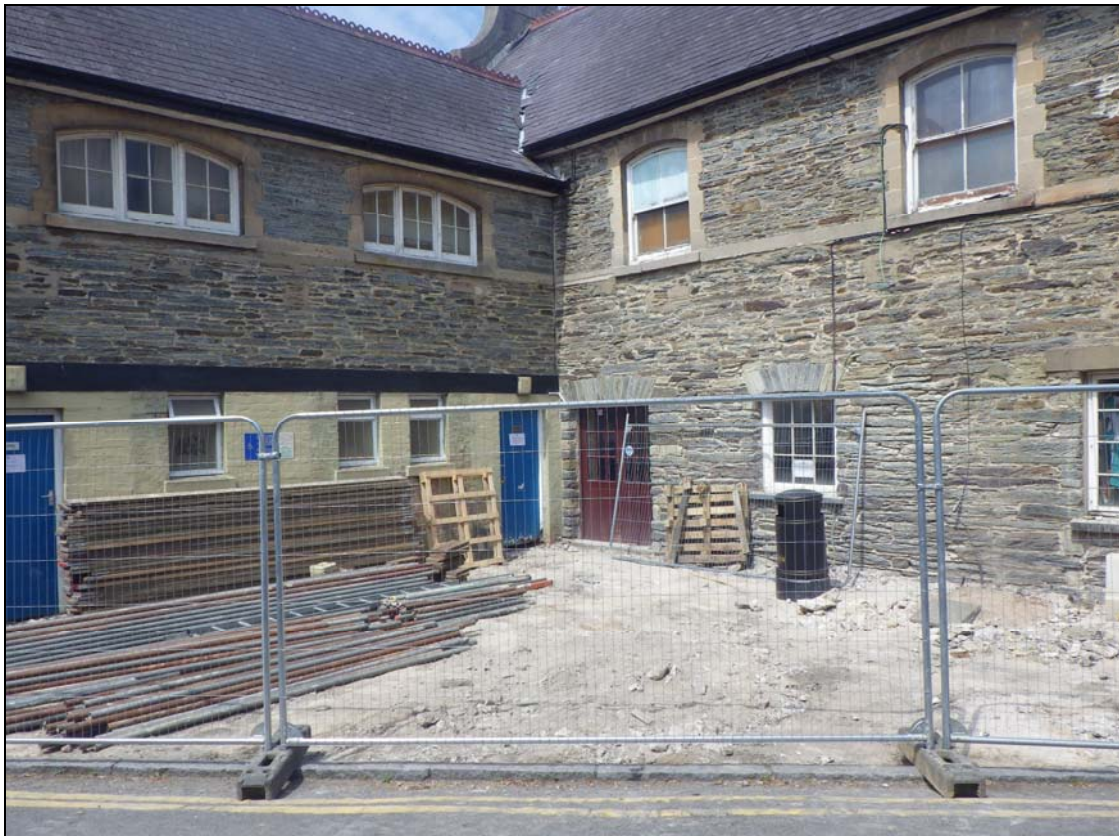
Plate 1: CHN2014_102: The rear of Cawdor Hall, looking northwest. To the left is the rear elevation of the 1892 extension, with brick reveals and voissours to its windows. To the right is the southern lateral wall of the earlier Market Hall, with original stone voissours remaining above the doorway and one window. The yellow brickwork in the upper floor shows that the roof of the original Market Hall was raised in 1892.
