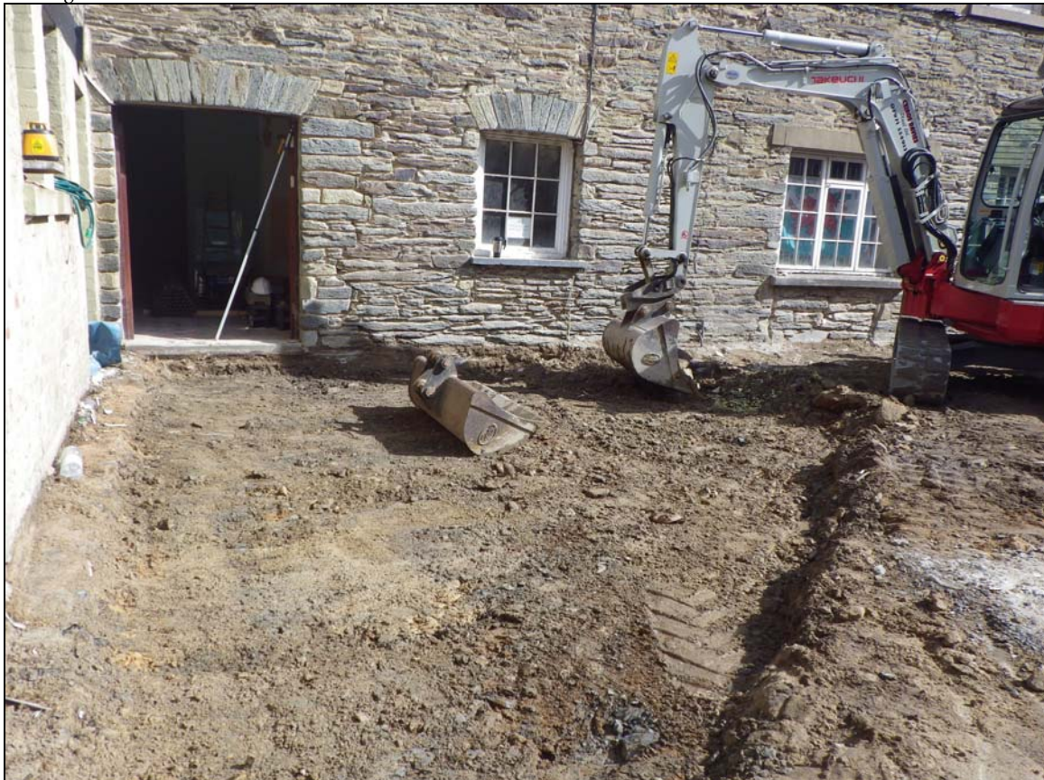
Plate 5: CHN2014_104: During removal of 003, the bedding layer below paving slabs 002, looking north.
