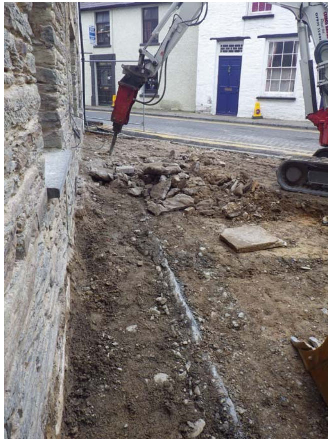
Plate 7:CHN2014_106: Removing concrete 001, the base of a former telephone box, from above cobble pavement 007, the up right edging, 005, of which is visible in the foreground, looking east southeast.
