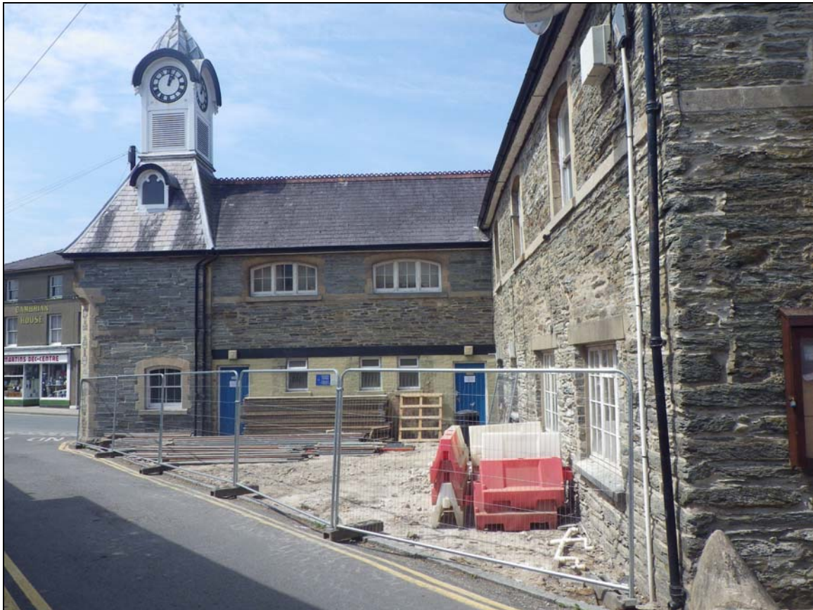
Plate 4: CHN2014_103: The rear of the Cawdor Hall, after the removal of the paving slabs, context 002, looking west.
