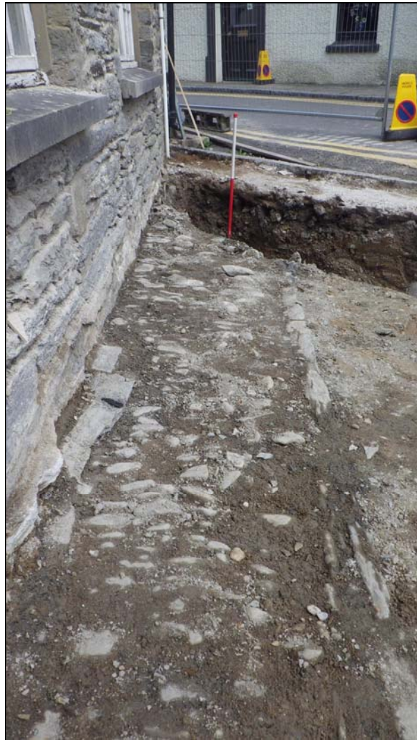
Plate 26: CHN2014_125: The cobbled pavement, 007, after the foundation trench for the new structure had been mechanically excavated, looking east southeast.
