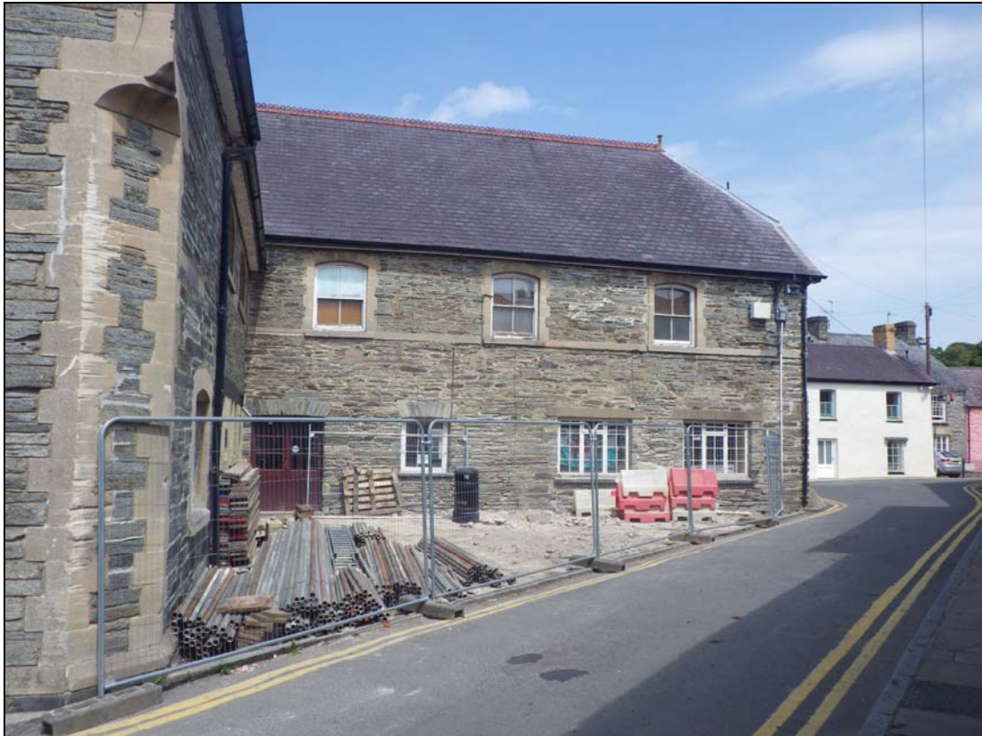
Plate 2: CHN2014_101: The rear of Cawdor Hall, after the removal of the paving slabs, context 002, looking north northeast.
