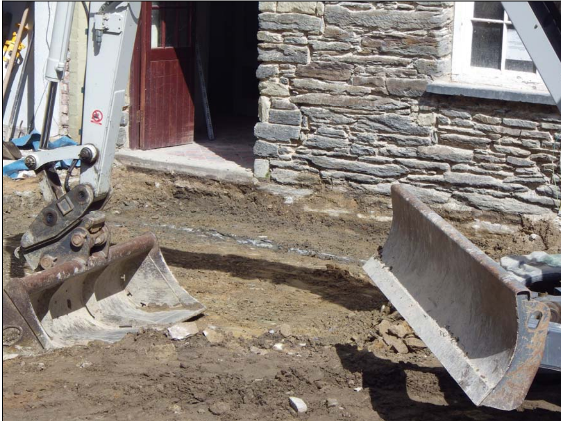
Plate 6:CHN2014_105: Cobbles 004 and upright edging slabs 005 of pavement 007 revealed after removal of 003, looking northwest.
