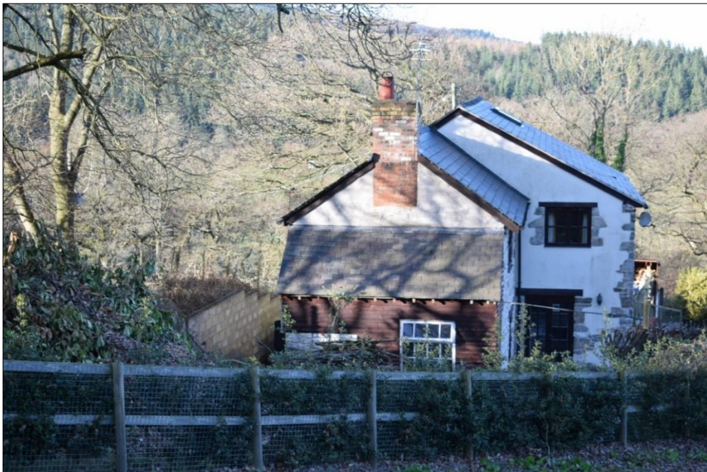
Offa's Dyke Unit 17: View from the south of the concrete block revetment at Croft Cottage (Issue 2). CPAT 4315-0023
