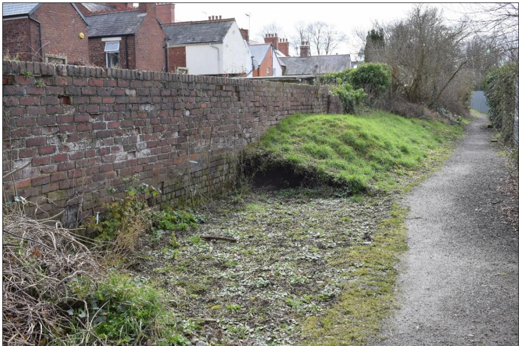
Wat's Dyke Unit 3: View from the north showing section through bank. CPAT 4317-0026
