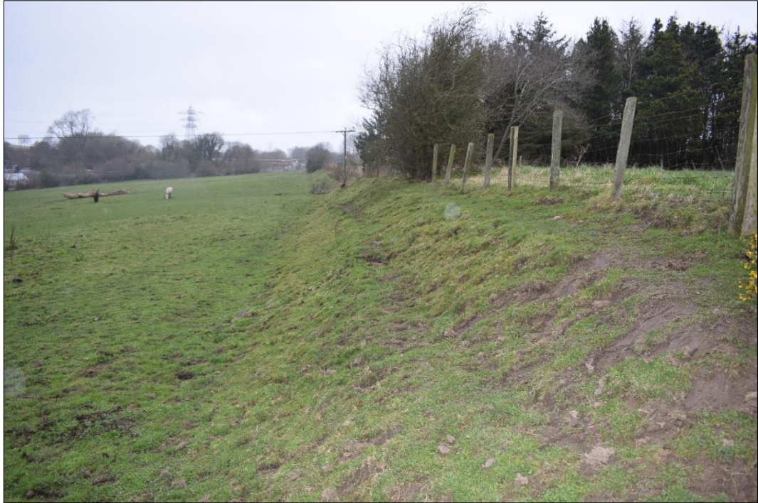
Offa's Dyke Unit 3: View to the north showing the pronounced scarp with minor stock erosion (Issue 1). CPAT 4326-0029
