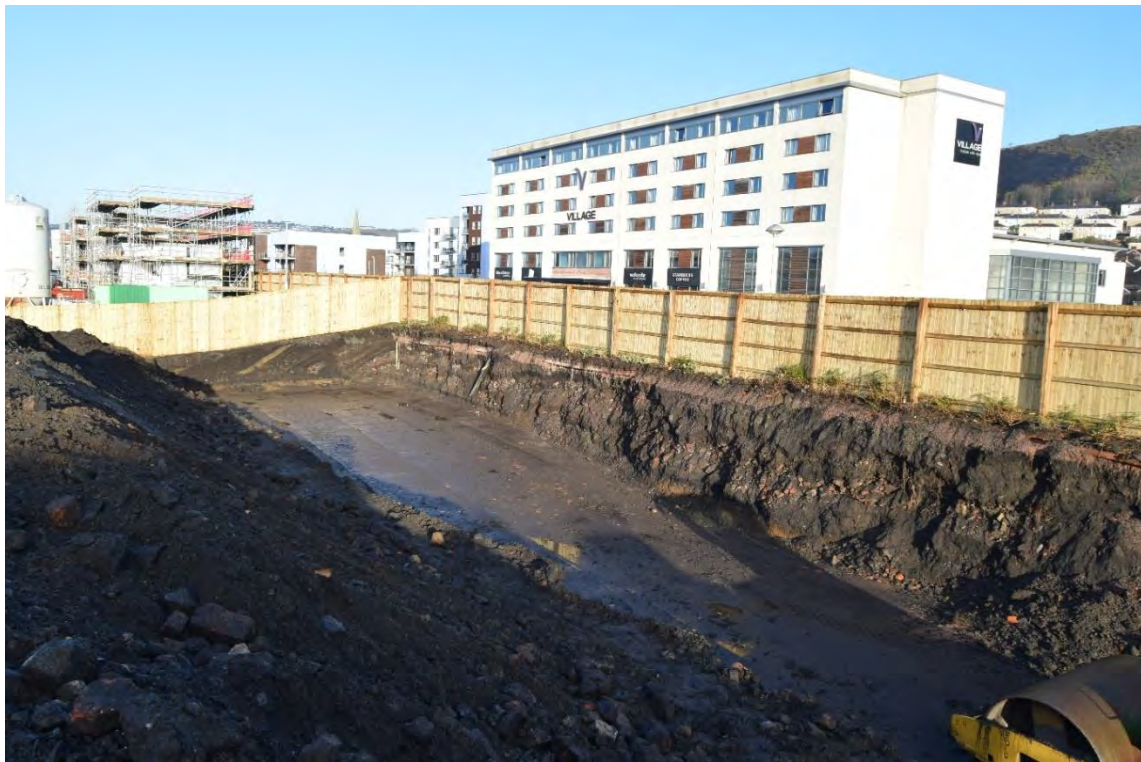
Plate 16: View northwest of plot 12-19 fully excavated and material being re-deposited and compressed.
