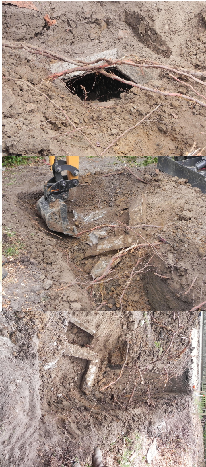
Figures 24 to 26 illustrating the modern cess pit leading from trench B to C
