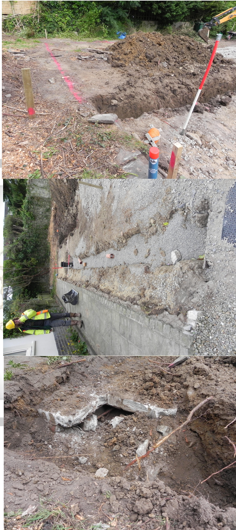
Figures 2 to 4, trench A under excavation, with spoil heap present. Length of utility trench north to south. Cess pit looking north in trench B/C
