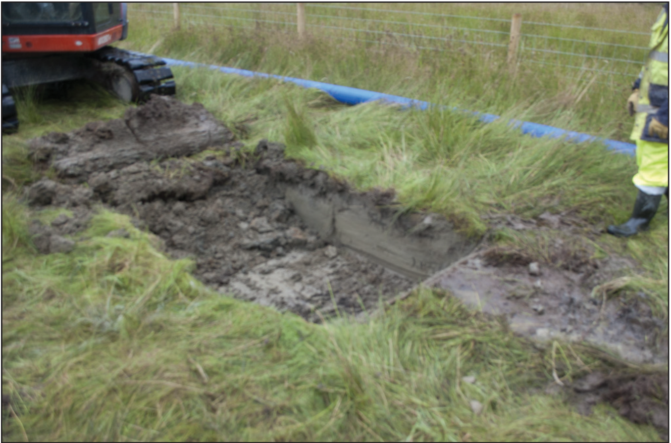
Plate 03: launch pit 1 - view from northwest with topsoil removed in early stages of excavation (archive image: G2528_002).
