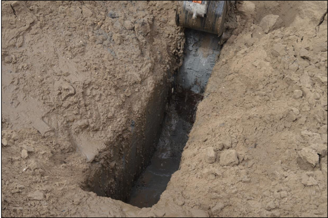
Fig. 4. Trial Pit 102, viewed from the south-east, organic peat deposits visible in section. Photo CPAT 4490-0004
