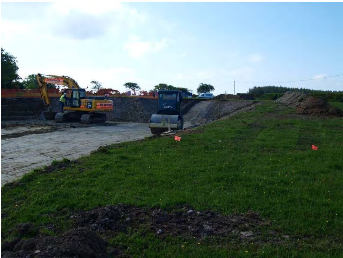
Photo 4: View south across the deeper excavations at the northern end of the access track as it enters the crane pad area.
