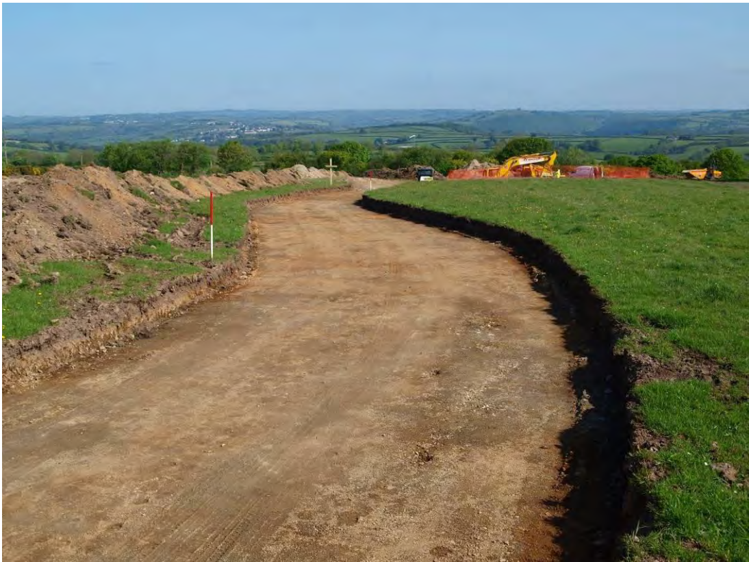
Photo 2: View north along the access track from the site compound, established close to the roadside. 1m scales.
