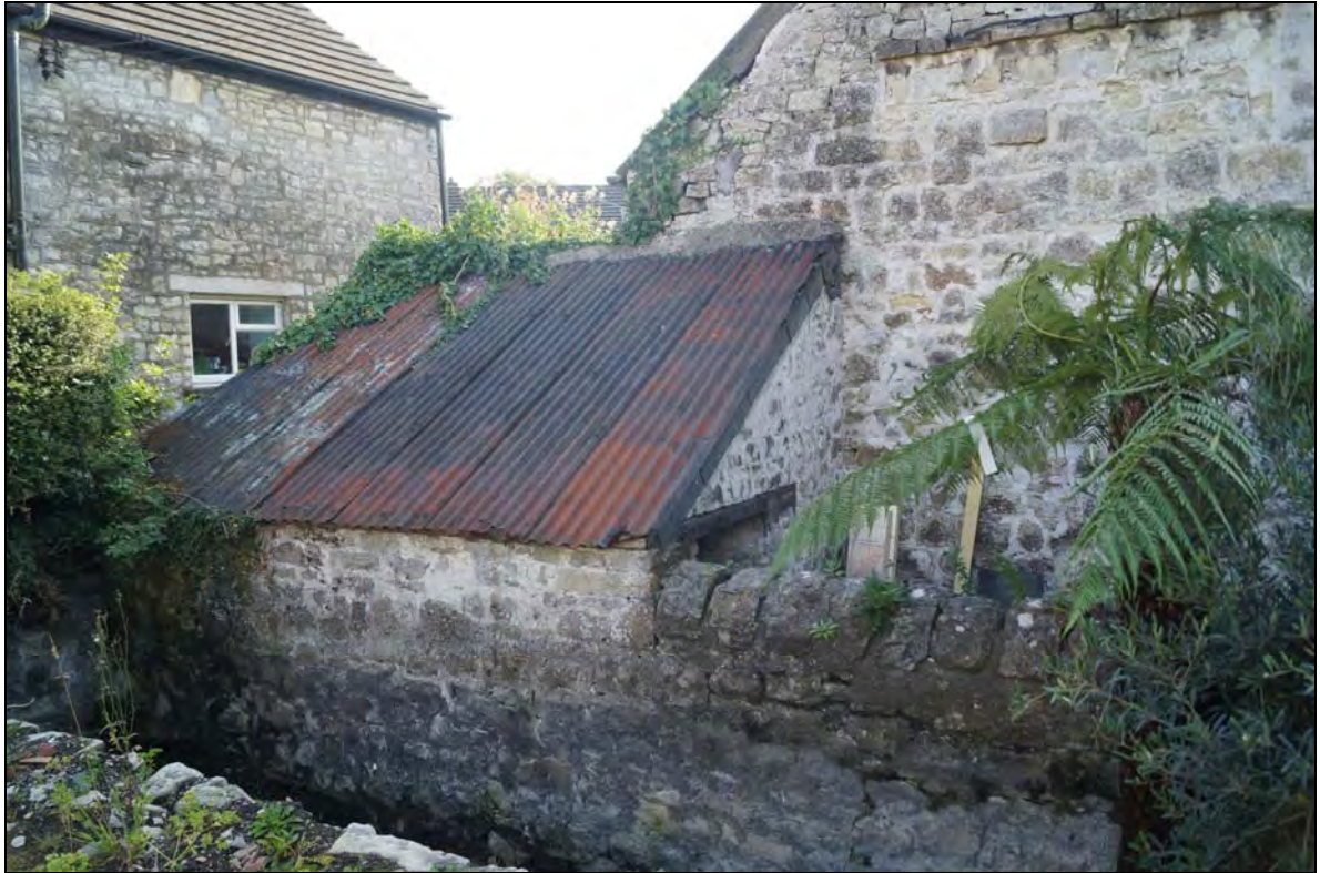
Plate 13: RCT2017_113, Former pigsty (F) and its yard wall (G) with the eastern gable wall of barn (A), looking south southwest.
