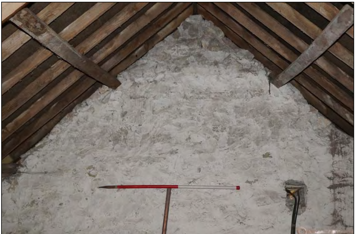
Plate 16: RCT2017_116, Internal view of eastern gable of barn (A), looking east northeast.
