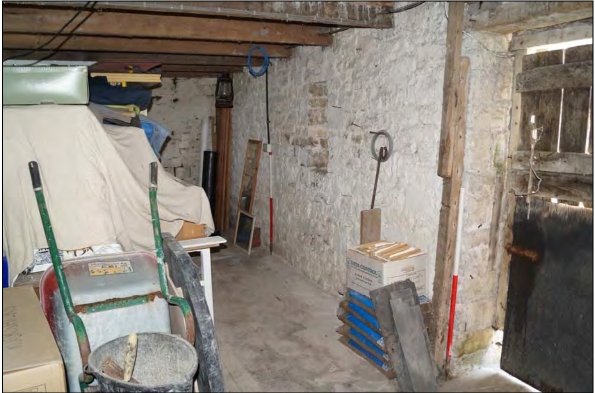
Plate 19: RCT2017_119, Internal view of eastern end of southern wall of barn (A), looking east-southeast.
