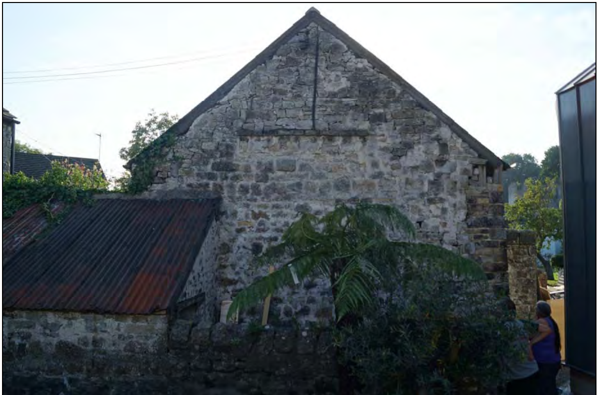
Plate 12: RCT2017_112, The eastern gable of the barn (A) with former pigsty and yard (F & G) in the foreground, looking west southwest.
