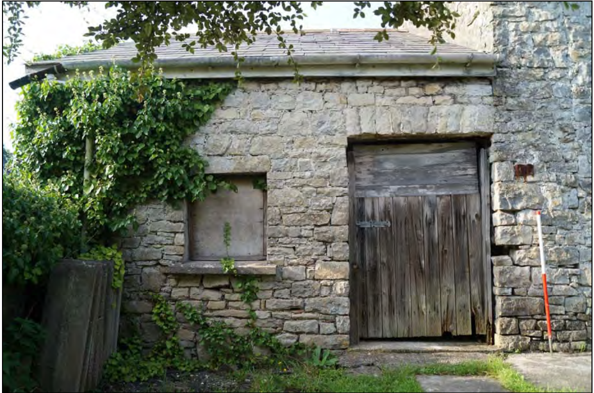
Plate 3: RCT2017_103, The low extension (B) to the west of the main barn (A) showing doorway and window, looking north northwest.
