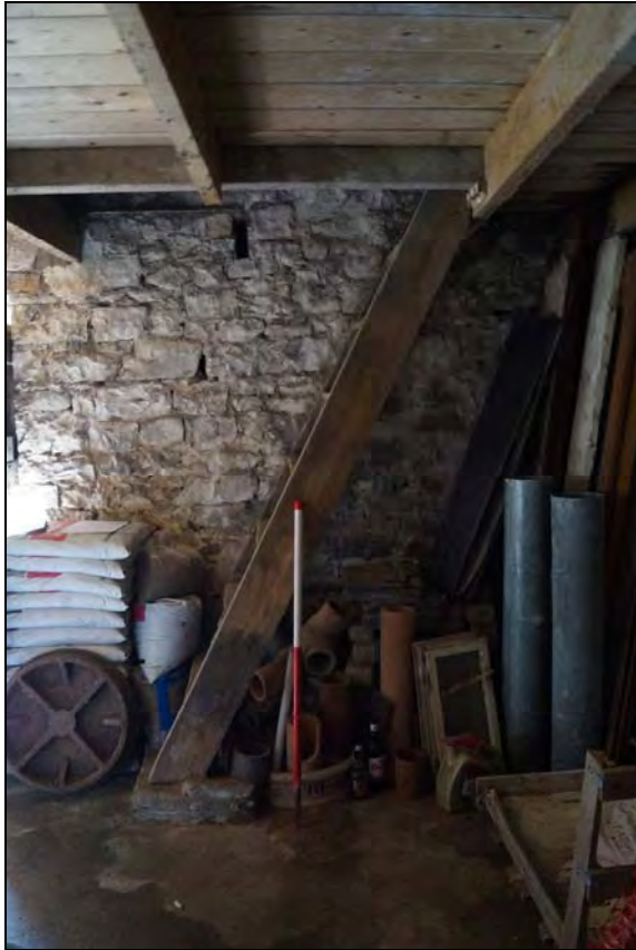
Plate 17: RCT2017_117, Internal view of western end of southern wall of barn (A), looking south southeast.
