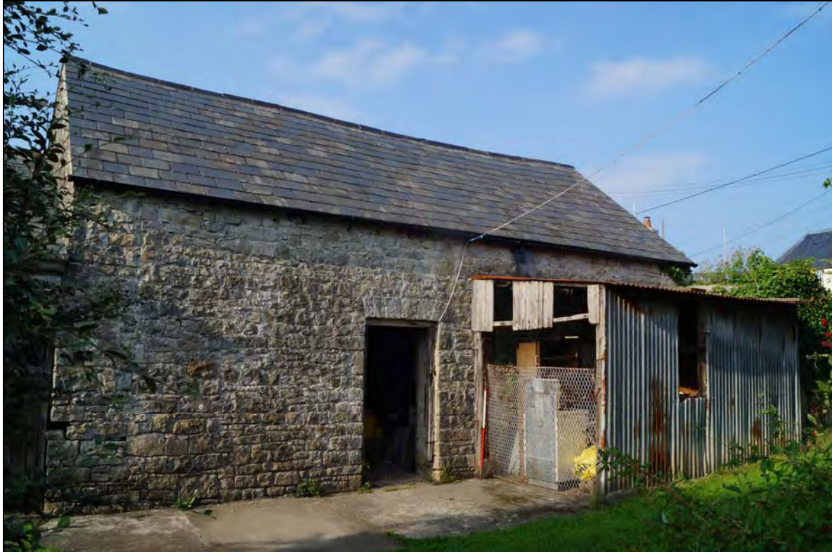
Plate 1: RCT2017_101, The main part of the barn (A) with the lean-to (H) visible to the right of the photograph, looking northeast.
