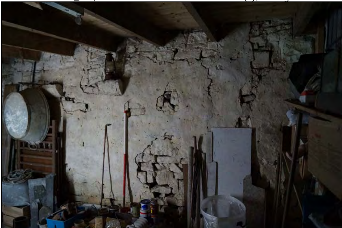
Plate 22: RCT2017_122, Internal view of eastern end of northern wall of barn (A), looking northwest.
