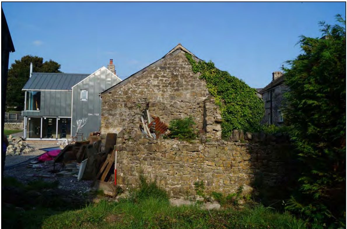
Plate 6: RCT2017_106, The western end of the building looking at the ruined western pigsty (C) and the gable end of the western extension (B). The gable of the main barn (A) is just visible above the extension gable, looking east northeast.
