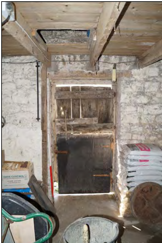
Plate 18: RCT2017_018, Internal view of doorway in southern wall of barn (A), looking south southeast.
