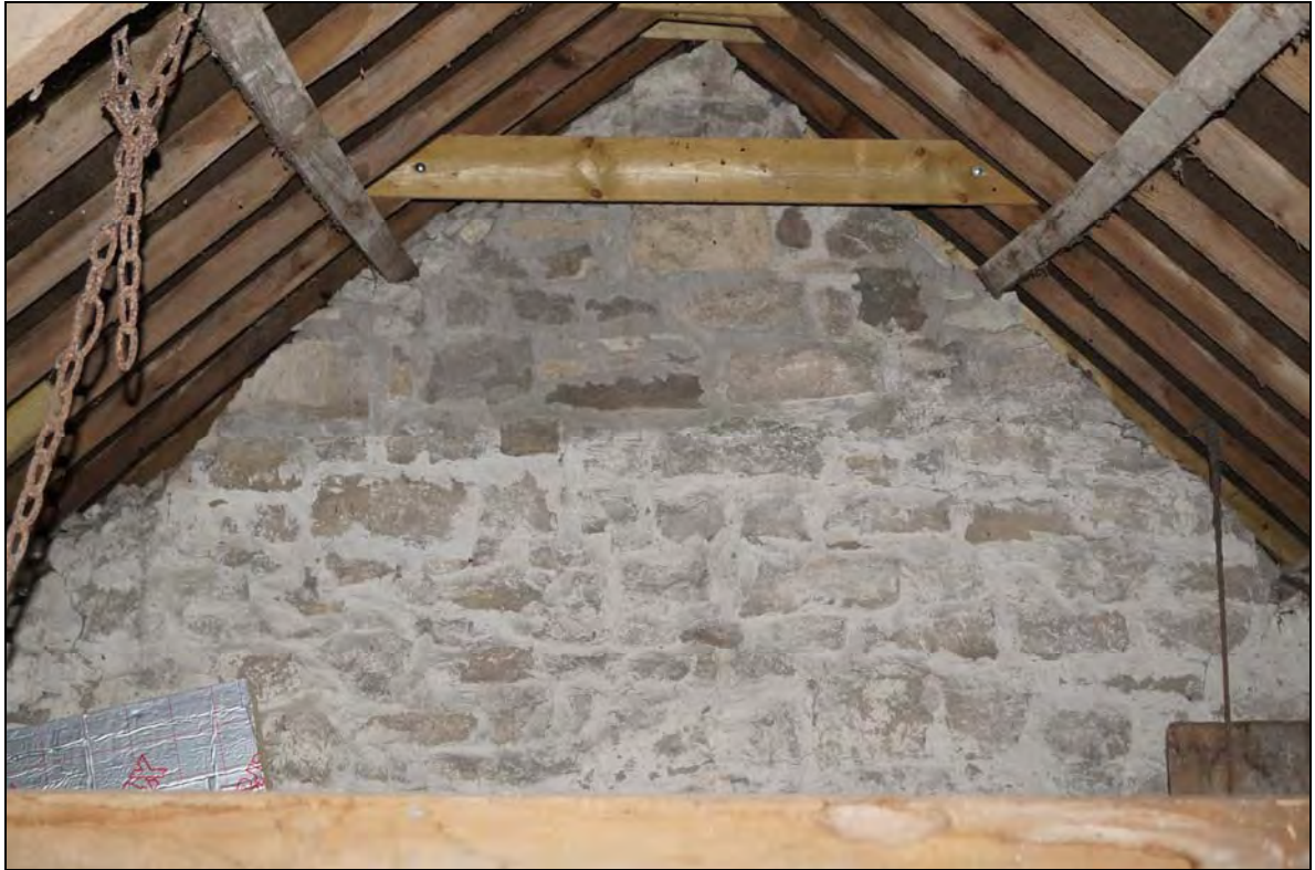
Plate 15: RCT2017_115, Internal view of western gable of barn (A), looking west southwest.
