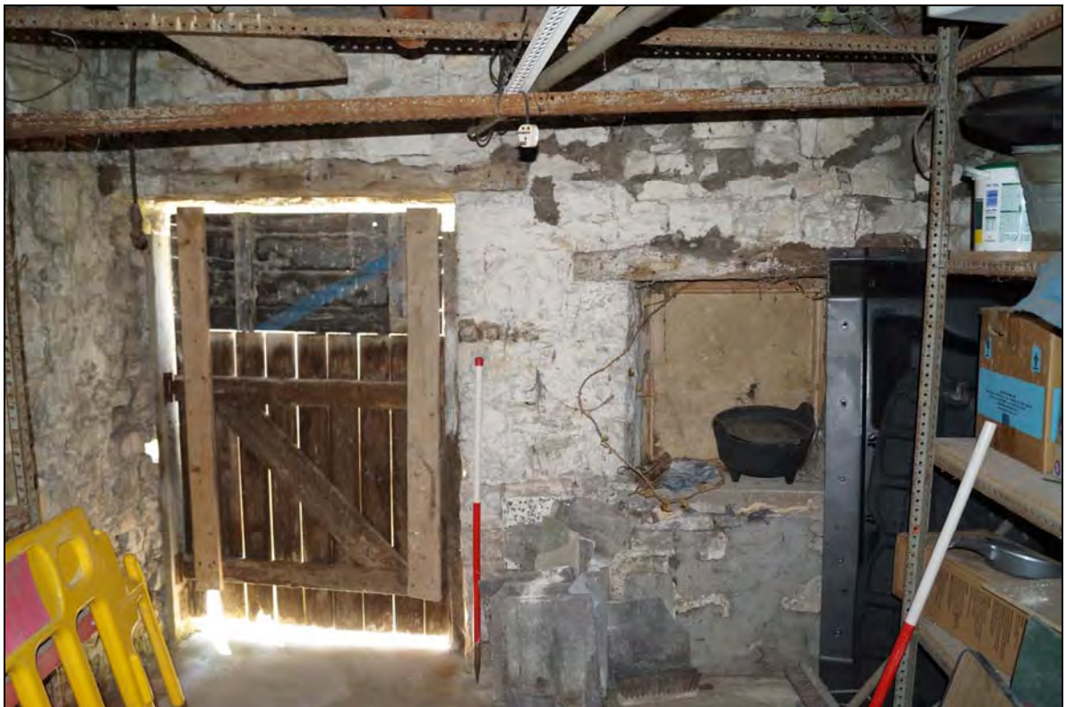
Plate 26: RCT2017_126, Internal view of southern wall of extension (B) showing doorway and window, looking south southeast.
