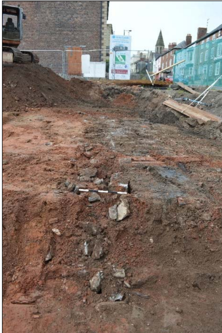
Fig. 14. The limestone wall (65) running parallel with the street frontage, truncated by modern services, with the front of the Old Police Station on the background. CPAT Photo 4030-0093
