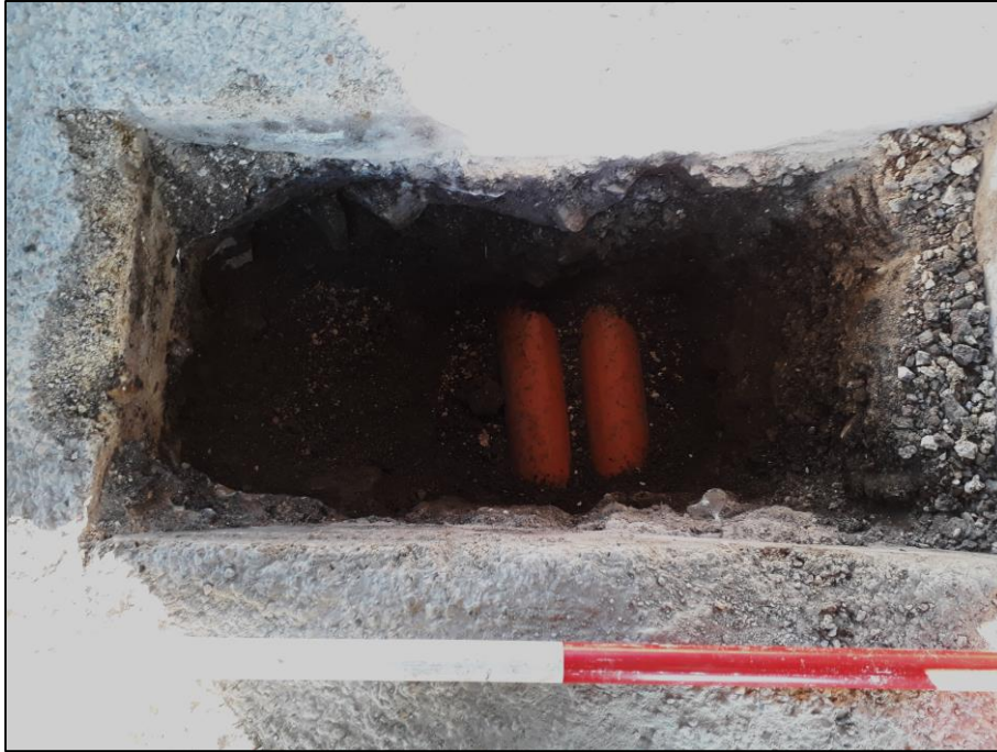
Plate 1. Plan view of Trial pit 1 showing the twin service ducts (104) underlying deposit 103. Scale divisions 0.5m
