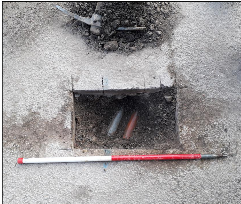
Plate 2. Plan view of Trial Pit 2 showing twin service ducts (204). Scale divisions are 0.5m.
