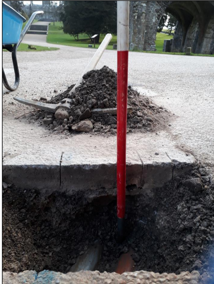
Plate 3. Oblique view of a section through Trial Pit 2 showing service pipes (204) and deposits 201-203. View to south, scale division 0.5m.
