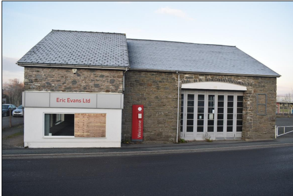
Fig. 4 South-east elevation showing the modern office extension (left of shot) and the large road access doorway Photo CPAT 4574-0006
