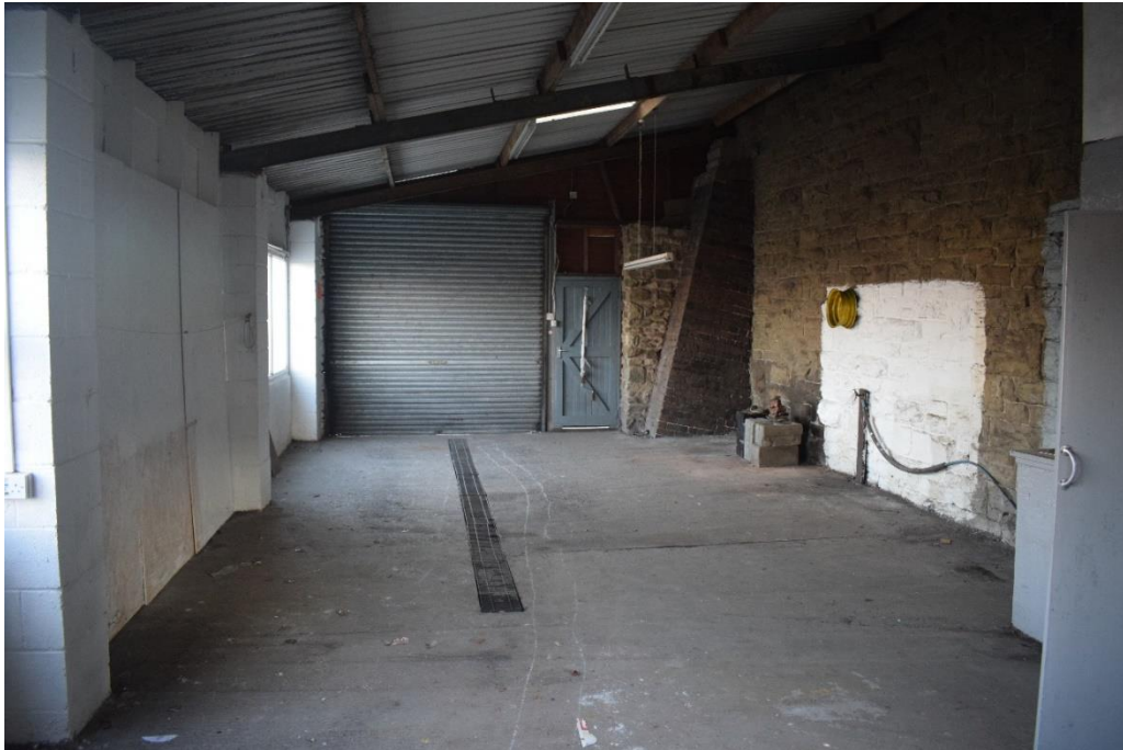
Fig. 9 View from the south-west of the garage extension showing one of the brick buttresses retaining the north-west wall of the goods shed Photo CPAT 4574-0029
