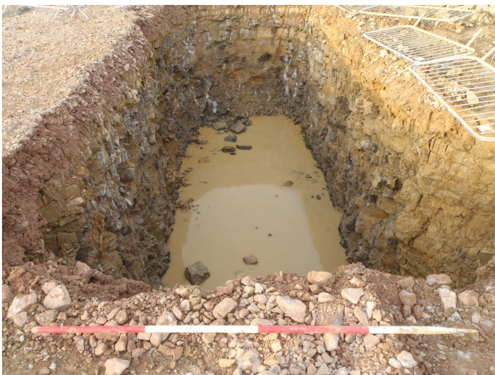
Plate 4, General view of excavated Stanchion Pad stratigraphy (Section 4), facing east (Scale 2m)
