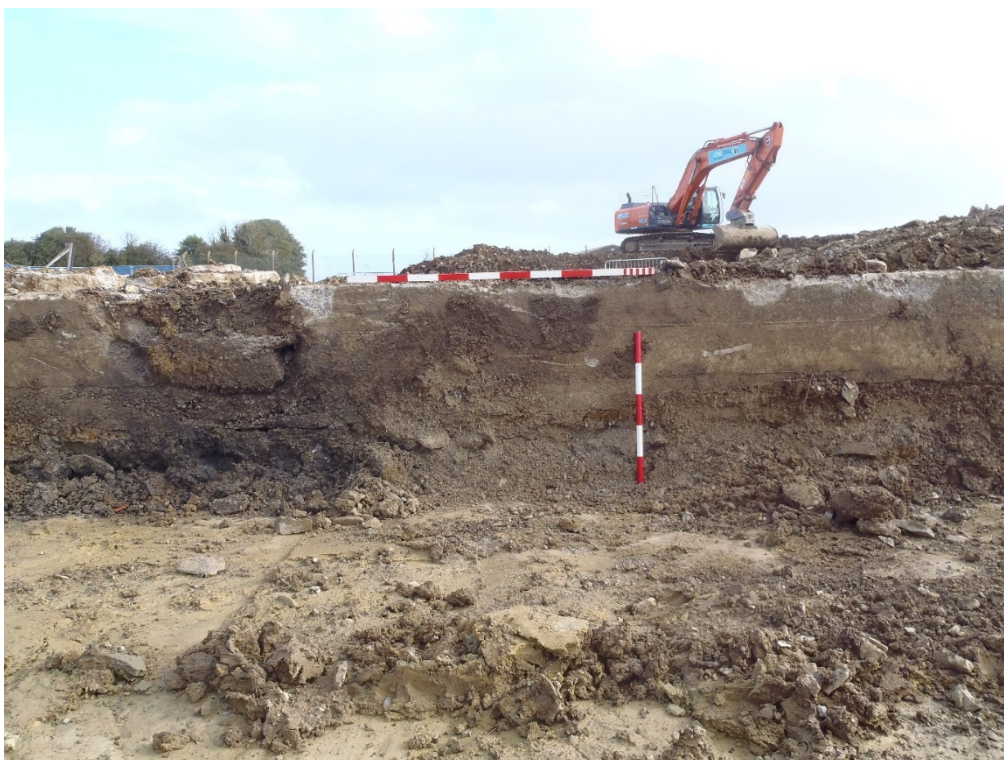
Plate 3, General view of excavated stratigraphy (Section 2) under former E3-Type building, facing east (Scales 1 & 0.50m)
