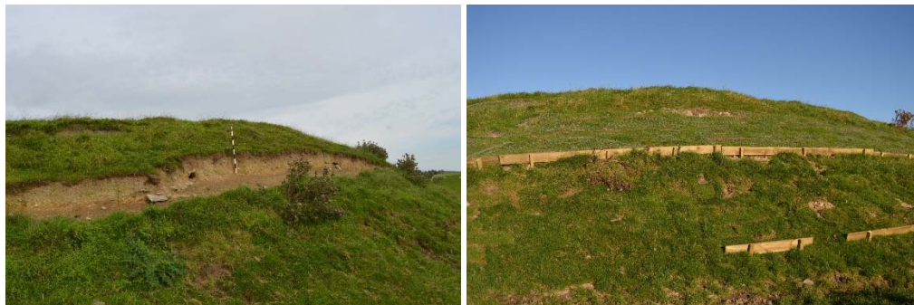
Figs 6 and 7. Extensive livestock and burrowing damage along south-east extent of monument before and after repair work. CPAT 4224-0028 and CPAT 4224-0133
