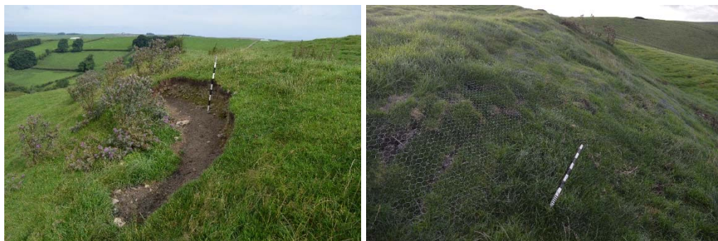
Figs 4 and 5. Large sheep scrape on south-west extent of monument before and after repair work. CPAT 4224-0008 and CPAT 4224-0093
