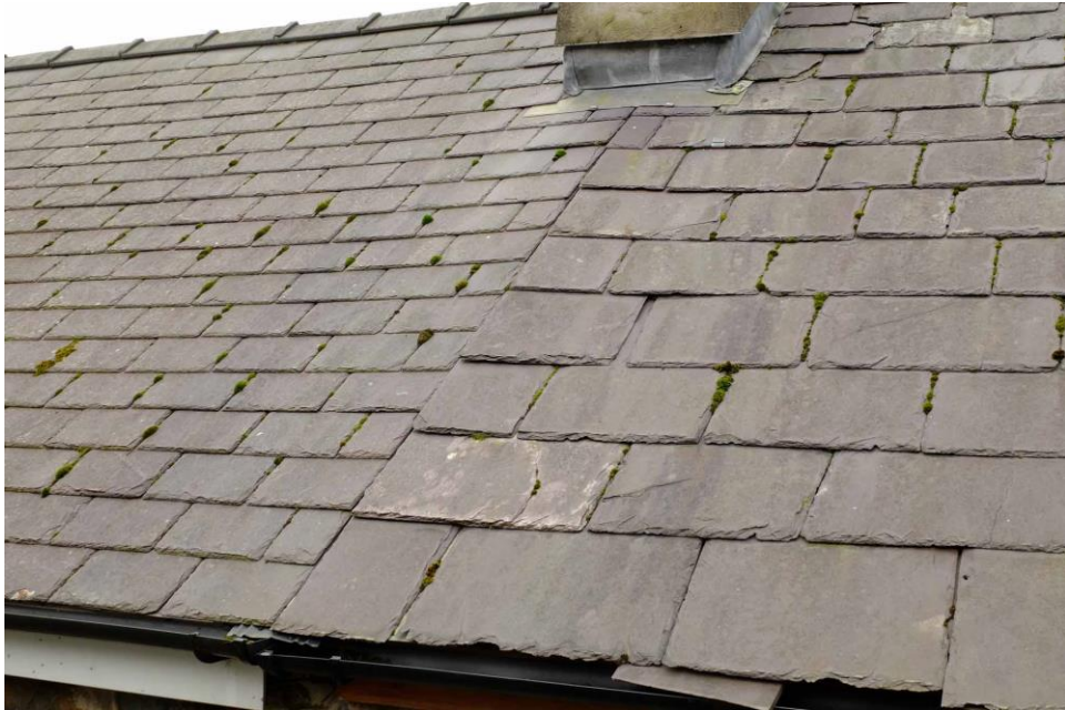
Fig 22 Roofs on Penybryn Terrace have slates of different sizes, the left side having been re-roofed.
