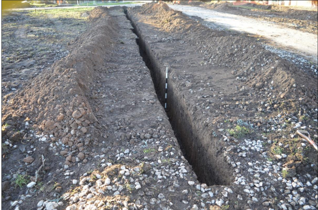
Fig. 3 Drainage trench in the central part of the car park Photo CPAT 4596-0011
