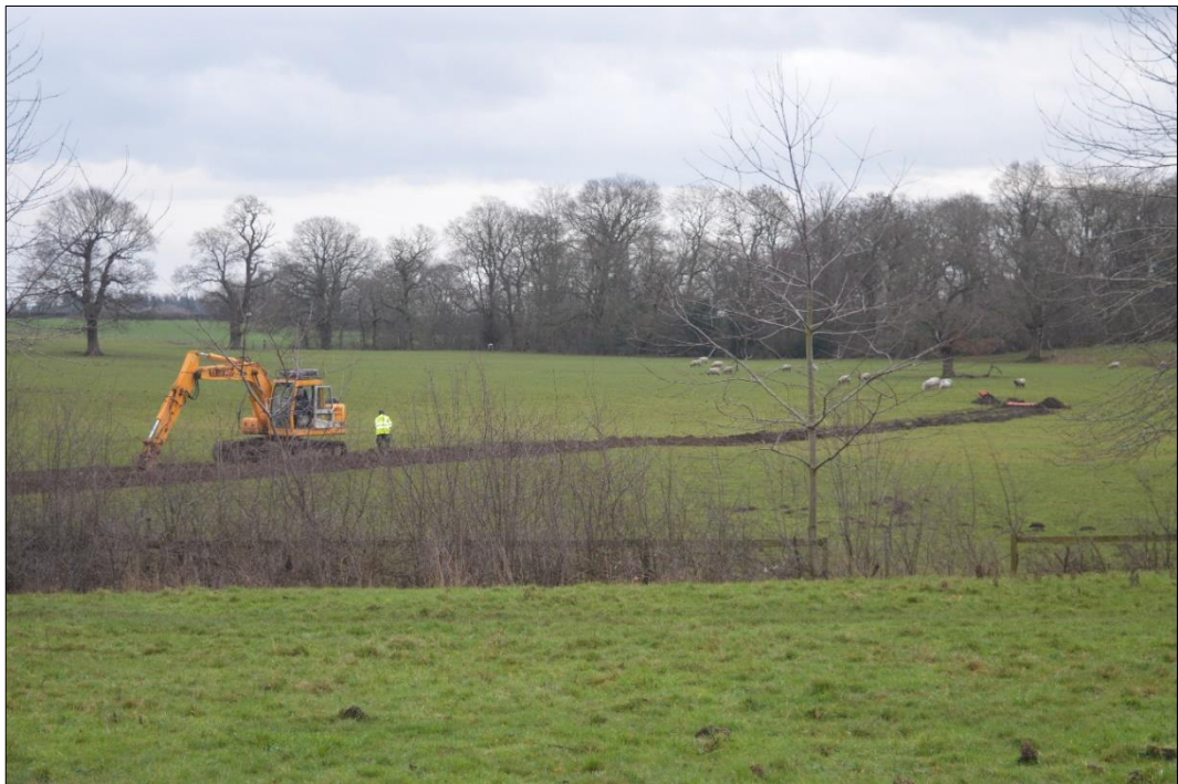
Fig. 6 The excavation of the new drainage connection across the park land. Photo CPAT 4596-0009
