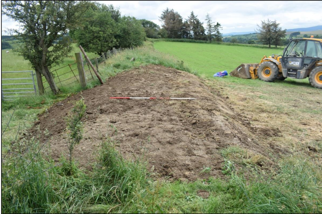
Fig. 8 The reinstated section of the Dyke viewed from the north. Photo CPAT 4663-019
