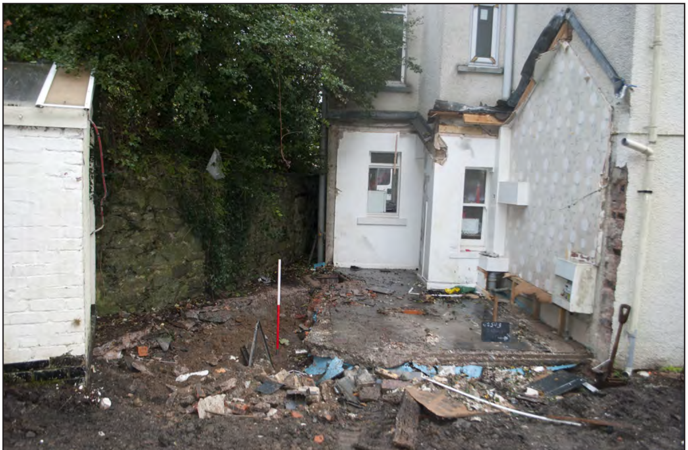
Plate 4: View of conservatory area subsequent to wall footing removal; slate floor in place; scale: 1x1m (archive reference: G2573_011).
