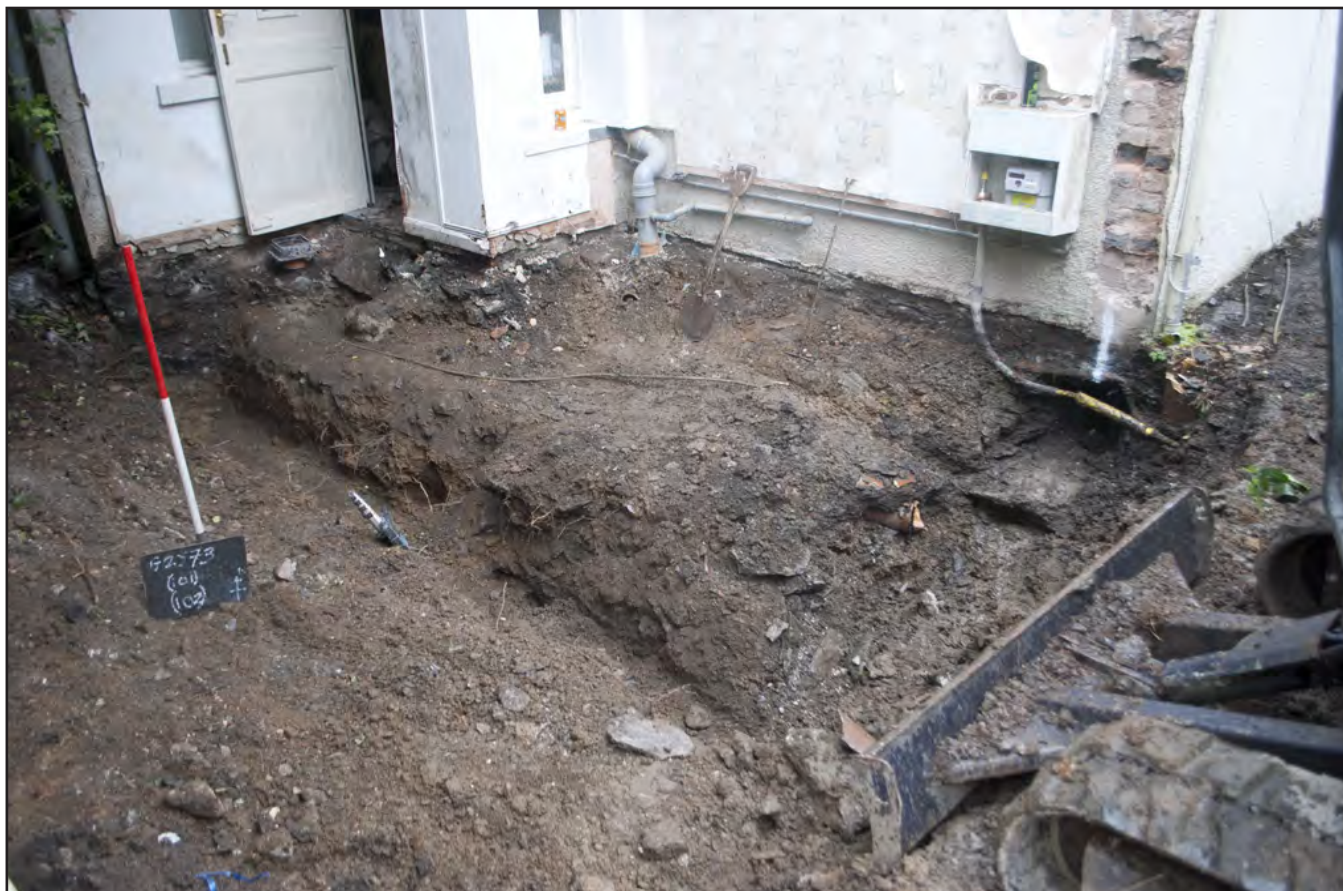
Plate 5: Angled view of new foundation trenches post-excitation; scale: 1x1m (archive reference: G2573_019).
