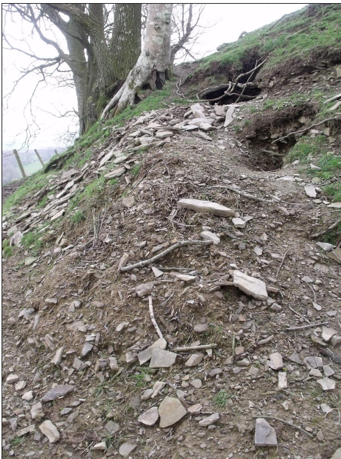
Fig.7 Damage caused by badger setts on the western side of Tomen Madoc – Photo CPAT 3808-0057
