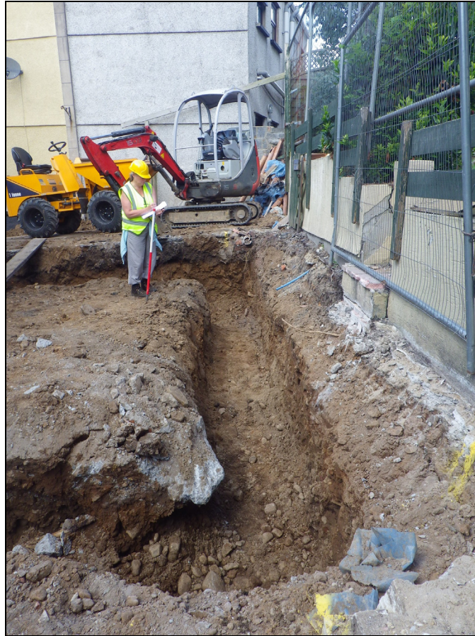
Plate 11: SRL2014_111, Looking along foundation trench from E to D, looking north northwest.
