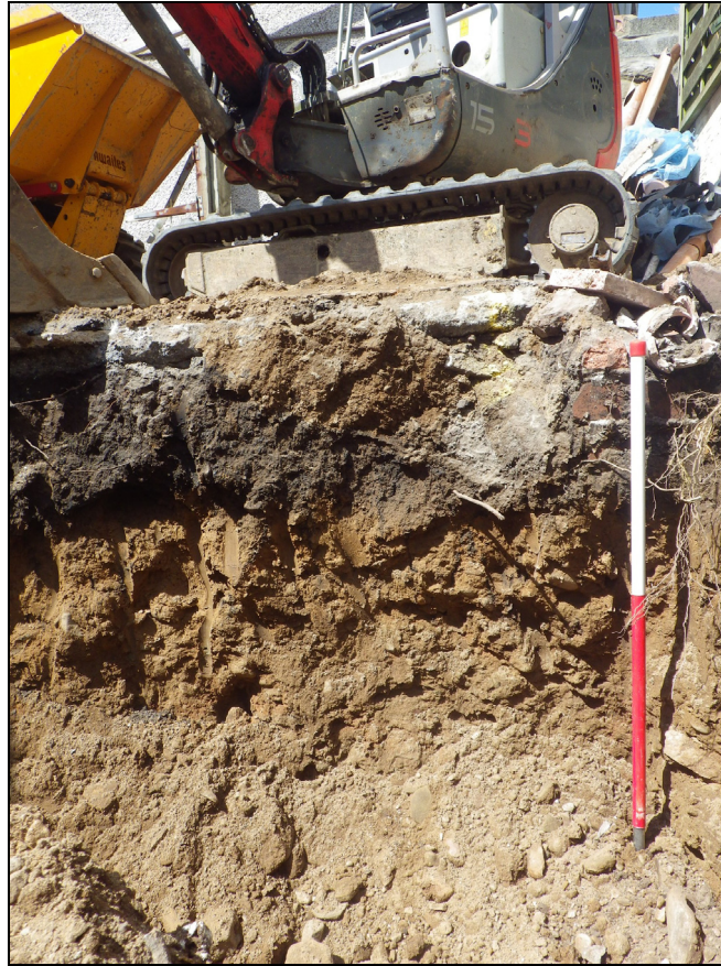
Plate 7: SRL2014_107, Foundation trench at the eastern end of C to D, looking north northwest.
