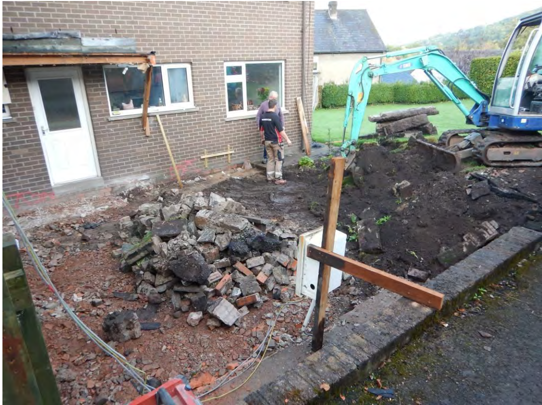
Photo 1: View northwest, general shot of site area after demolition, and during initial excavation works.
