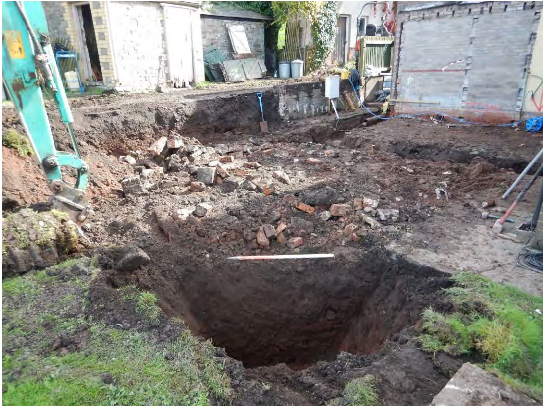
Photo 7: General view southeast across the development site after excavation works. The soakaway lies in the foreground, with the foundation trenches to the rear. 1m scale.
