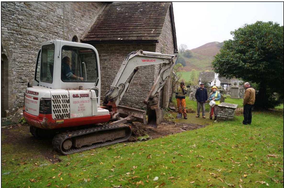
Plate 4: SMG2017_104, the eastern part of the path from the porch to just beyond the west end of the church. This area was only scraped, off and under most of was a metalled surface, looking northeast
