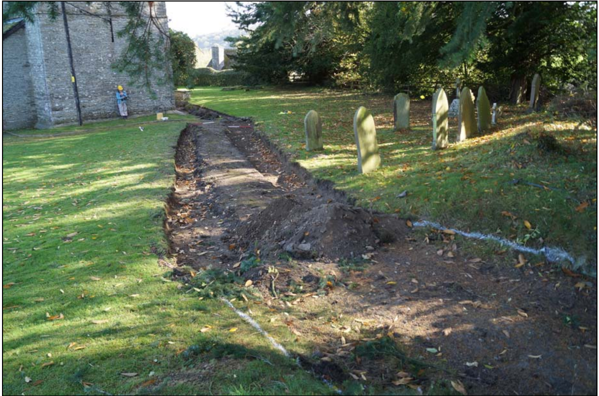
Plate 14: SMG2017_114, Excavated trenches A and B, and central area of pathway retained, looking east northeast
