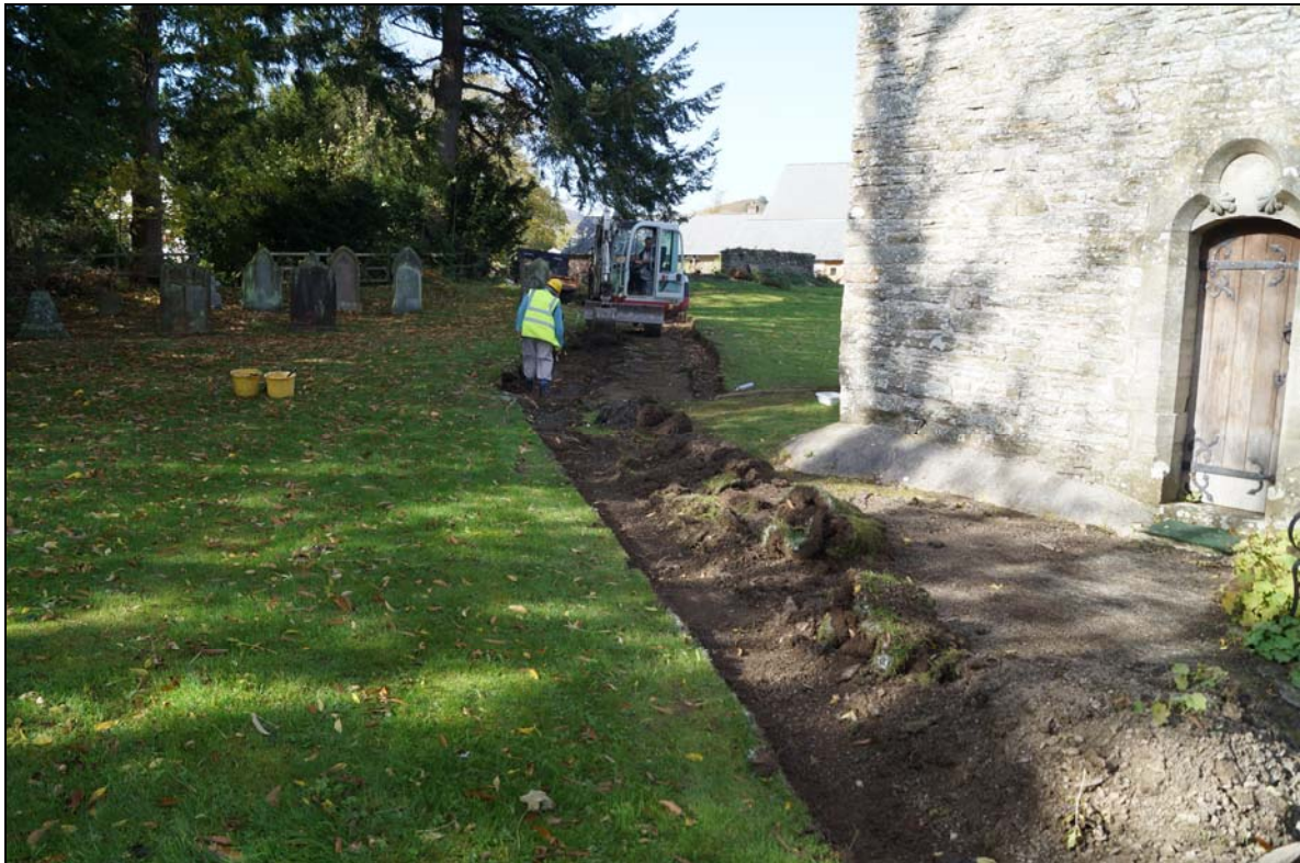
Plate 6: SMG2017_106, Turf only removed from the area of path in front of the church, no archaeologically significant contexts observed, looking west northwest.
