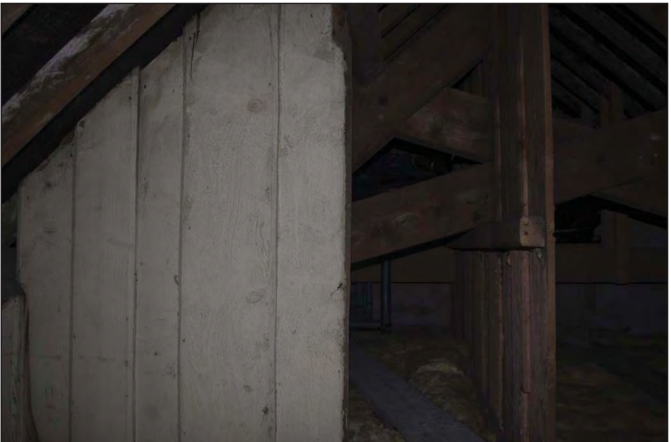
Plate 42: View of wooden storage partitioning with in roofspace of House 1, baring similar resemblance to the partiton walls in House 2 (photographic archive ref. G2520_053)
