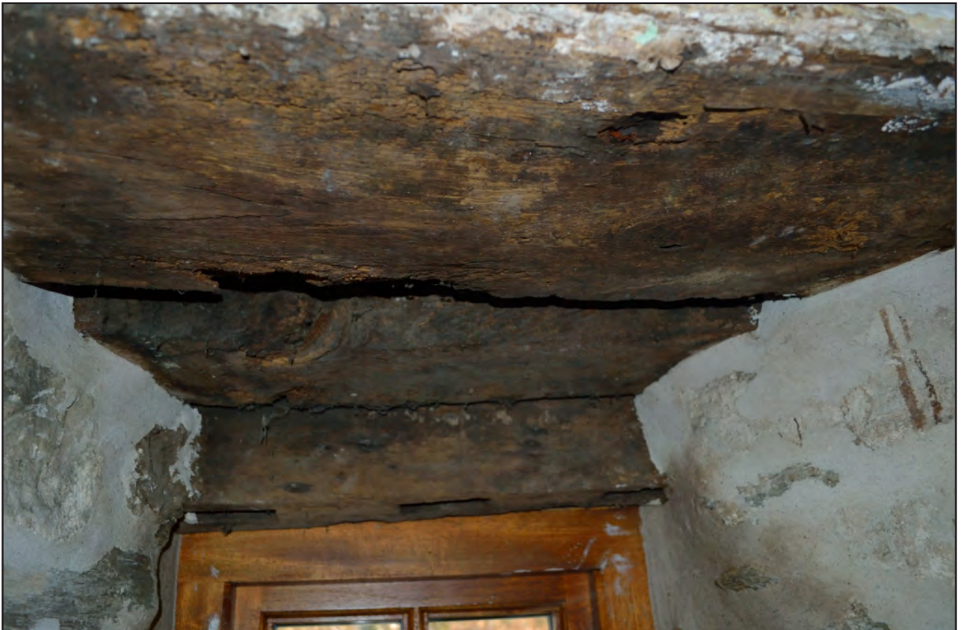
Plate 57: Detail of WB02, showing the three lintel beams, with outermost one with three mortice holes (10cm x 3cm) cut into it (archive reference: G2520_1126).
