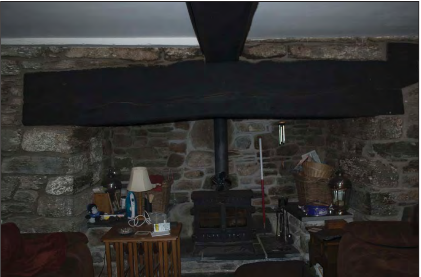
Plate 18: View of late 16th century fire range F02 within Lounge 1, with visible peg holes within the lintel (photographic archive ref. G2520_35)
