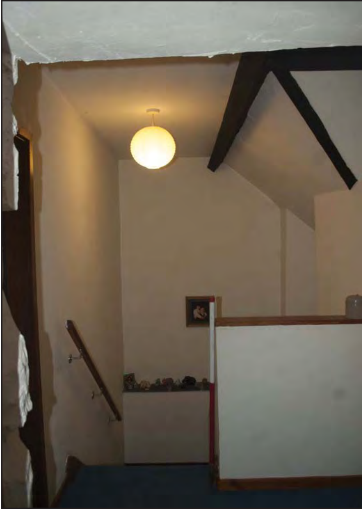
Plate 29: Modern staircase insertion on lounge 1 with internal view of blocked window WB01, staircase leads into Hall 1. (photographic archive ref. G2520_067)
