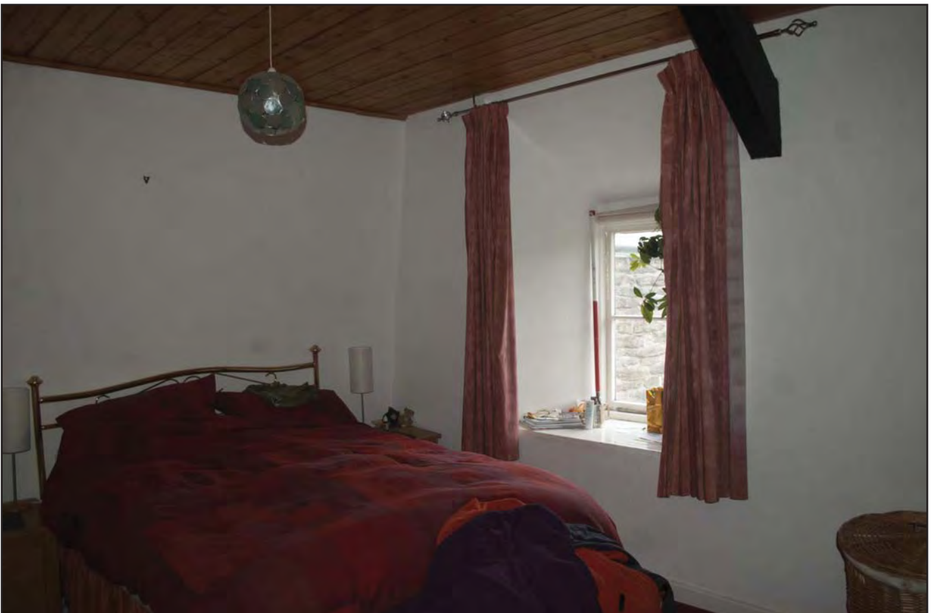
Plate 24: View of Bedroom 3 with visible painted attic truss overhang (photographic archive ref. G2520_050)
