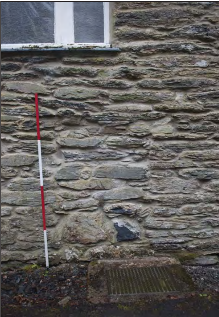
Plate 10: View of visible blocked doorway DB01 below window W13, may have possibly been part of the late 16th century cross-passage (photographic archive ref. G2520_018)
