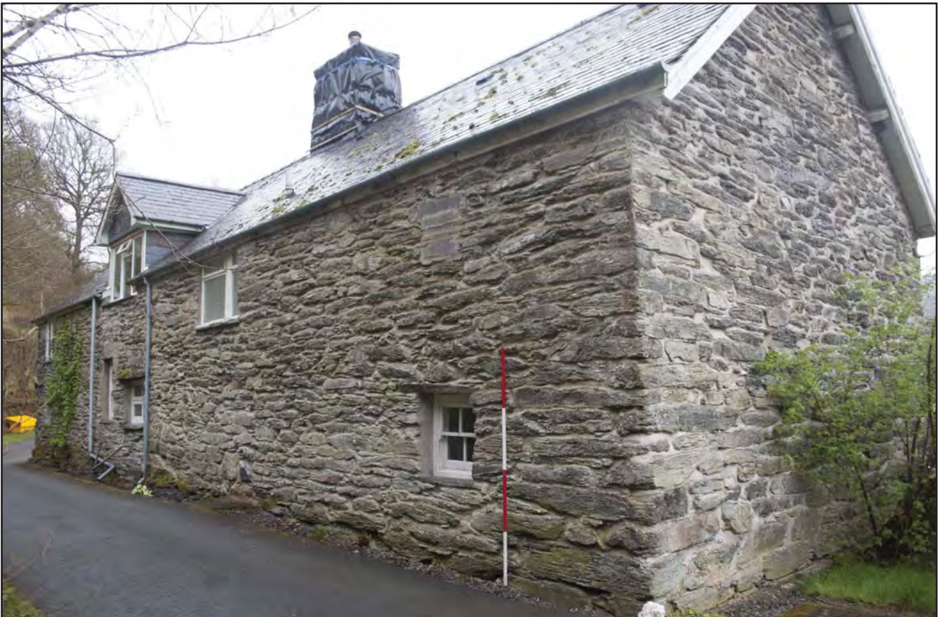
Plate 08: Oblique view of the western elevation of late 16th century section of House 1, with view of blocked window WB02 (photographic archive ref. G2520_014)
