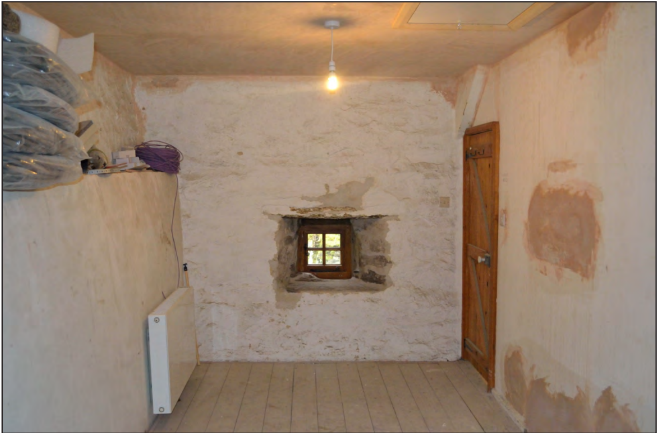
Plate 56: General view of NW wall of bedroom 4 showing location of WB02 (archive reference: G2520_1128).
