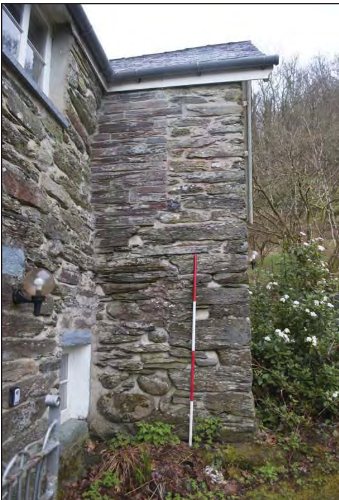
Plate 02: View of blocked window WB01 on the east facing elevation of the north gable end of House 1. (photographic archive ref. G2520_003)
