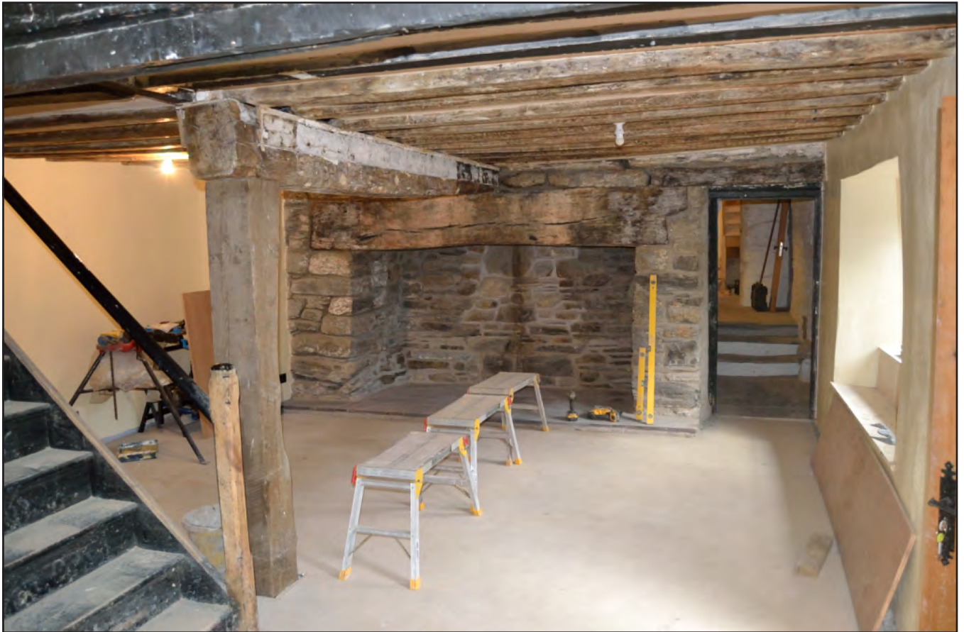
Plate 58: General view of Lounge 1 (House 1), showing its current stripped out character (archive reference: G2520_1121).
