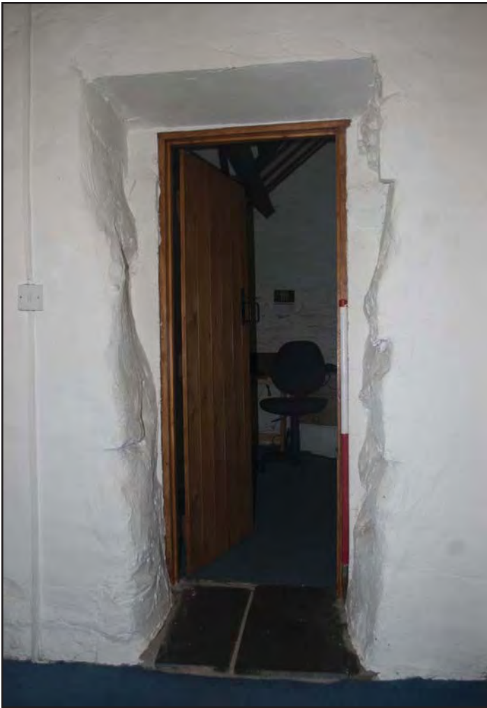
Plate 27: View of doorway D16 cut into the former northern gable end after further 18th century extension (photographic archive ref. G2520_066)
