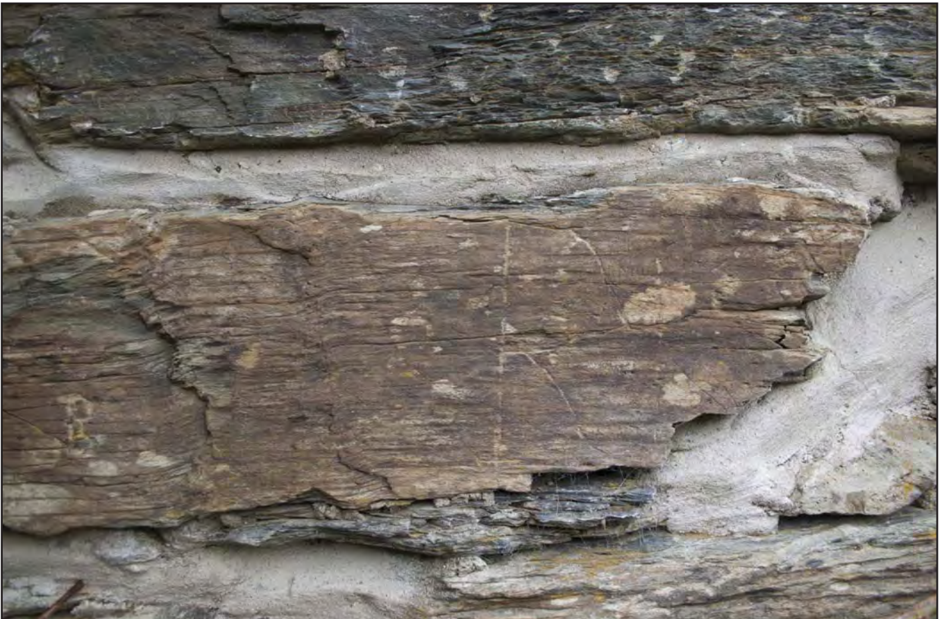
Plate 14: View of the letter 'R' and geometric criss-cross patterns scratched onto a stone in between windows W06 + W07 on the southern 17th century elevation of House 2 (photographic archive ref. G2520_011)
