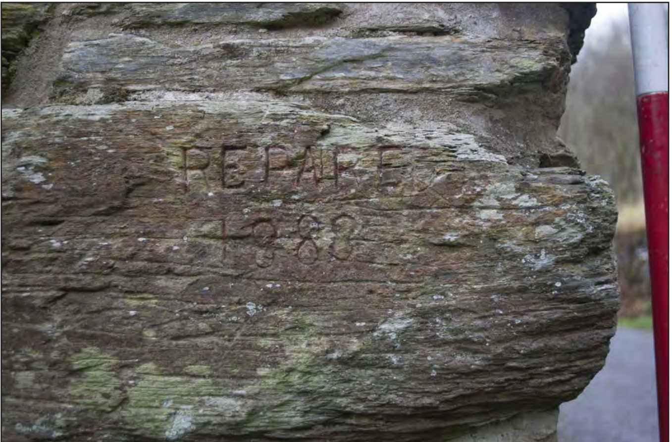
Plate 12: Close-up view of "REPAIRED 1883" engraved into the north facing quoin of House 1 north gable end (photographic archive ref. G2520_007)
