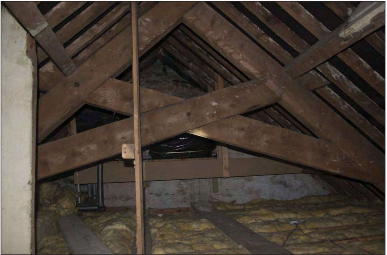
Plate 41: View of 20th century replacement timber roof truss in House 1 (photographic archive ref. G2520_052)
