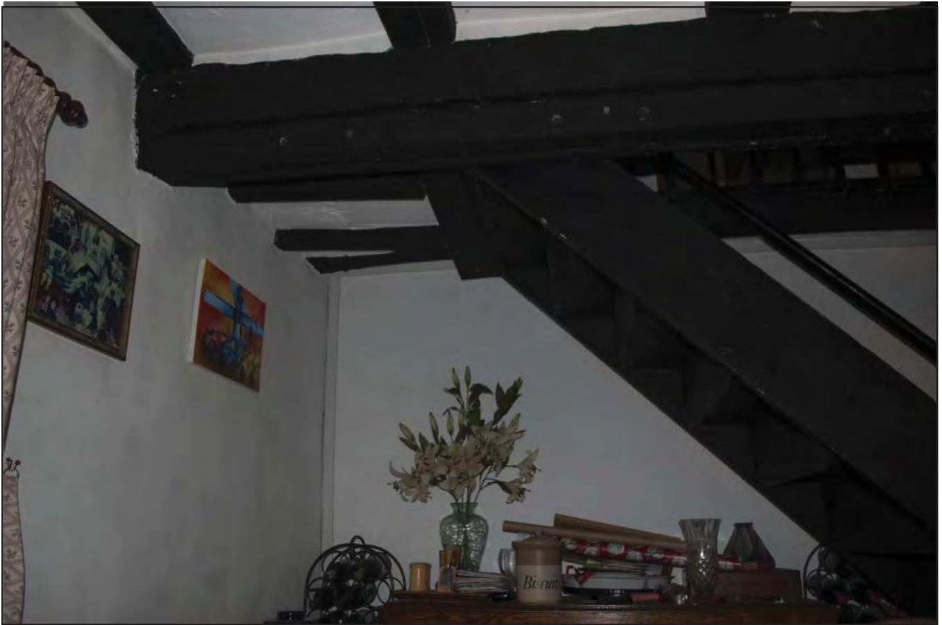
Plate 21: View of earlier narrow beams on a eastern-western beams, alongside visible peg holes within the central beam (photographic archive ref. G2520_044)
