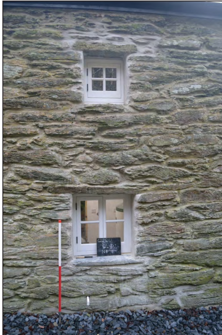
Plate 52: Detail of replacement windows WB02 and W03; scale: 1x1m (archive reference: G2520_1113).
