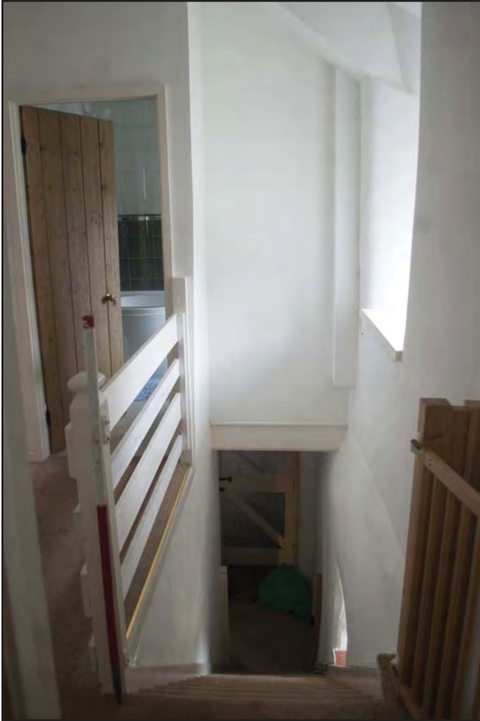
Plate 37: View of stairwell showing ground floor elevation against first floor expansion on north facing wall, with view of early 20th century staircase fittings (photographic archive ref. G2520_094)
