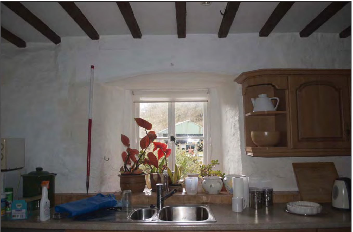
Plate 36: View of window W06 displaying arched lintel, previously belonging to the main entrance of the 17th century cross-passage (photographic archive ref G2520_080)
