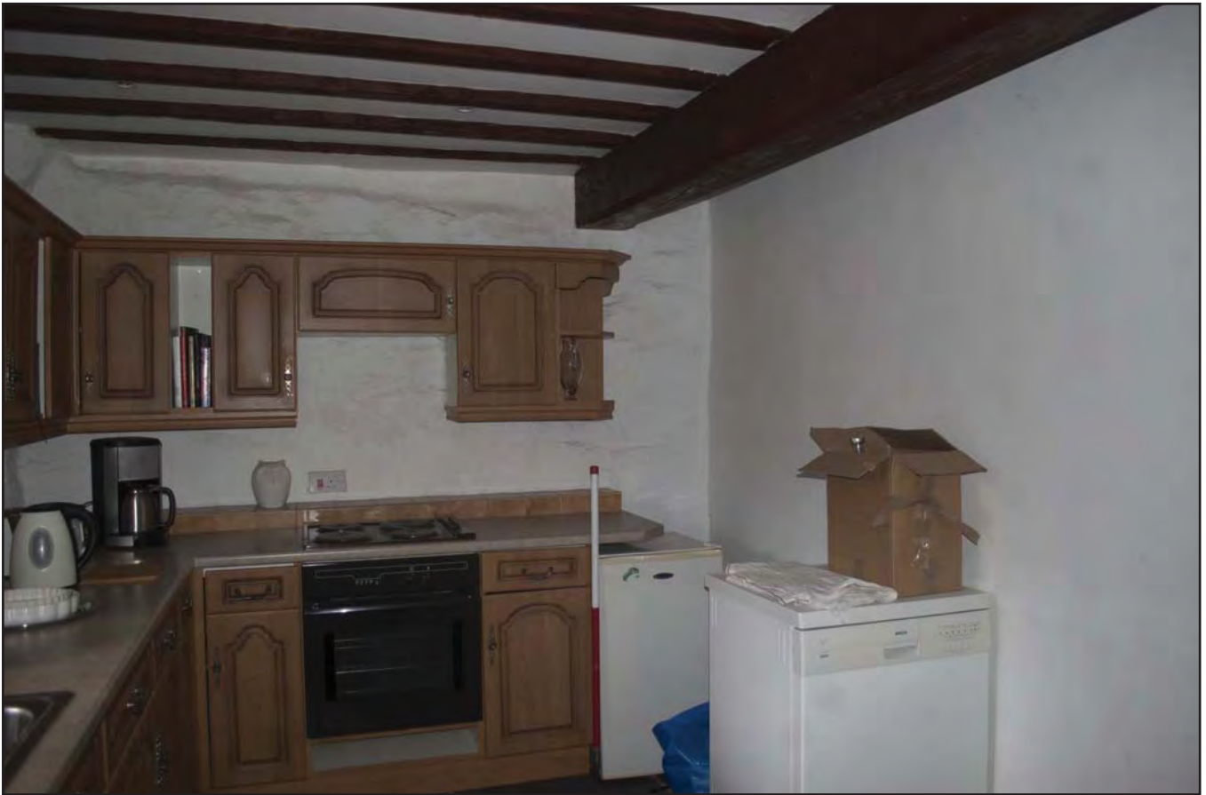
Plate 35: View of west facing wall within Kitchen 2, displaying uneven surface at ceiling edge subjected to renovations (photographic archive ref. G520_078)
