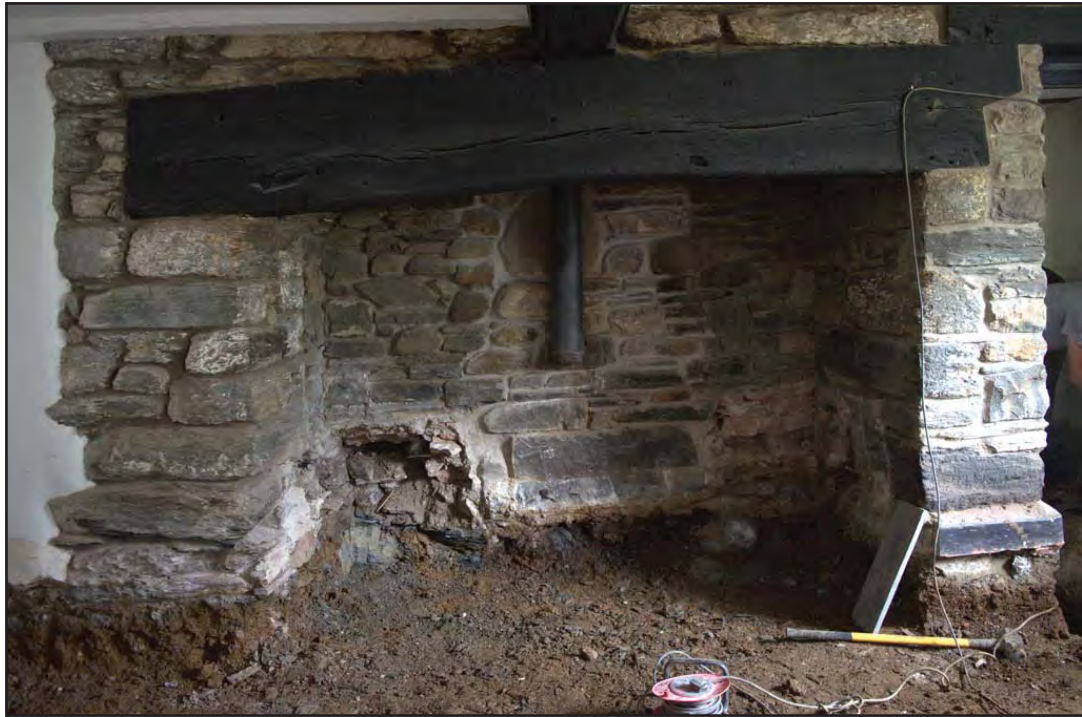
Plate 49: Shot of fireplace following removal of modern features; scale: (archive reference: G2520_1104).
