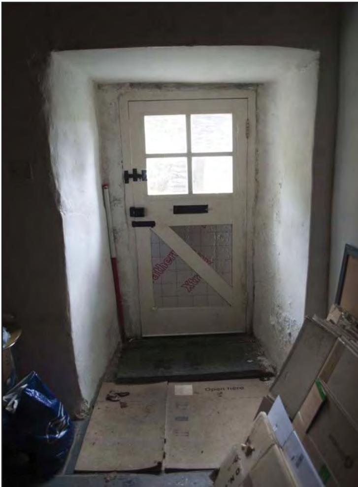
Plate 30: View of doorway D01, the northern end of the 17th century cross-passage, with 1930s half glass paneled door (photographic archive ref. G2520_068)
