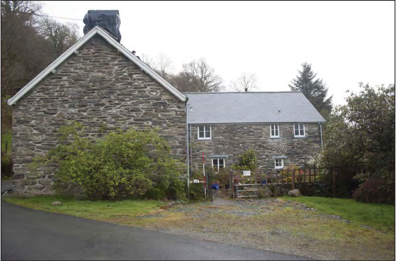
Plate 05: View of House 1 south gable end, with visible evidence of roof raising. Alongside with the view of House 2 the southern elevation (photographic archive ref. G2520_009)
