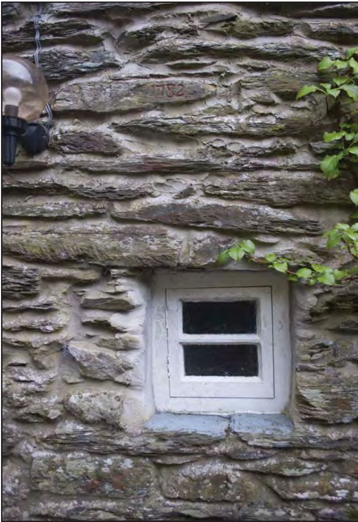
Plate 15: View of window W10 on western elevation demonstrating a later window size reduction, alongside with dates 1782 engraved into a stone above, with visible remnants of red Ox-blood paint (photographic archive ref. G2520_017)
