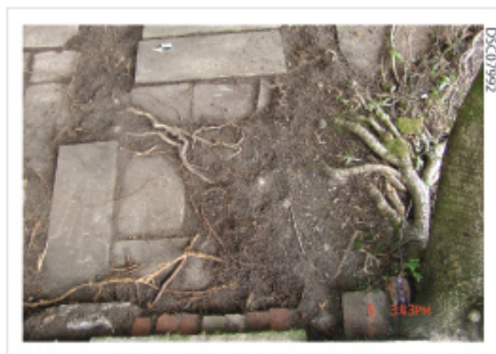
Plate 20: Mid terrace showing tree root damage
