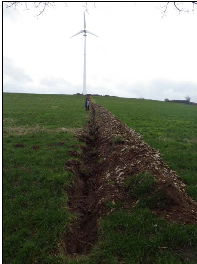
Plate 3: PGI2014_103, the northern part of the cable trench running north from the eastern turbine, looking south southeast. This part of the cable trench was open, but revealed no archaeological contexts or artefacts.
