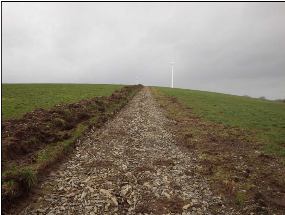
Plate 4: PGI2014_104, the eastern cable trench running east from the eastern turbine, looking southwest. The area stripped of topsoil was visible but no archaeological contexts or artefacts were revealed.
