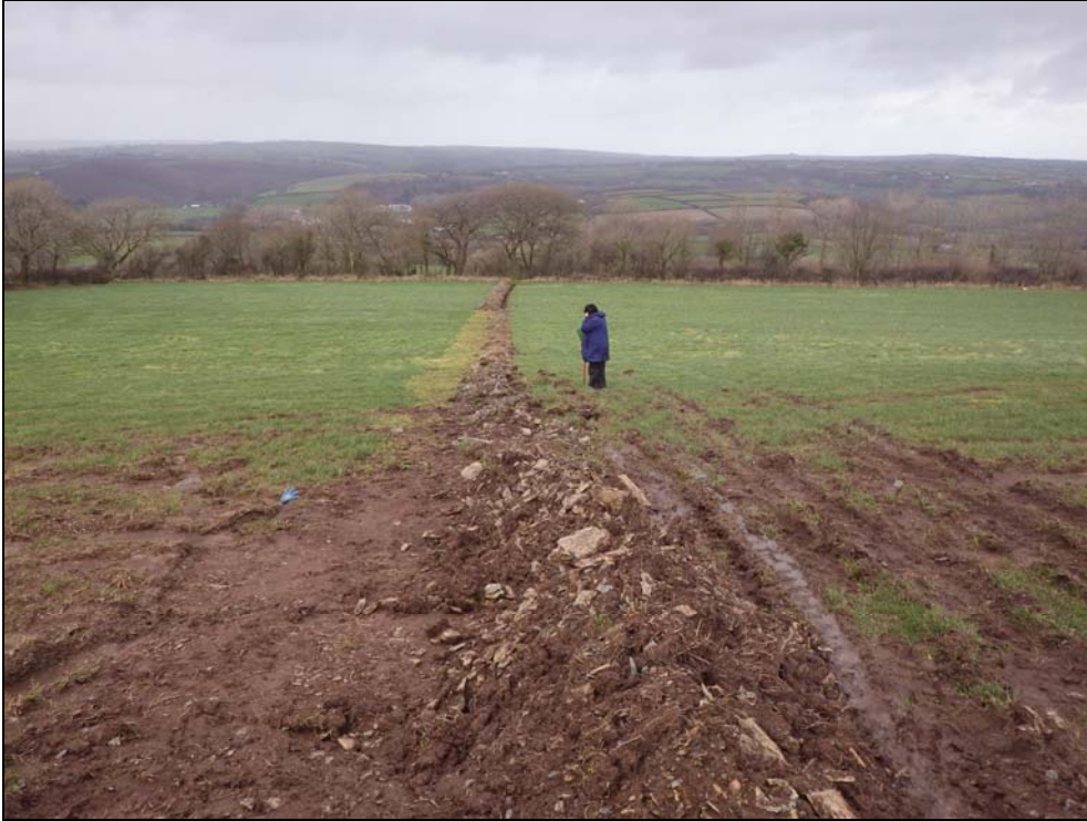
Plate 1: PGI2014_101, the southern part of the cable trench running north from the eastern turbine, looking north northwest. This part of the cable trench had been re-covered.
