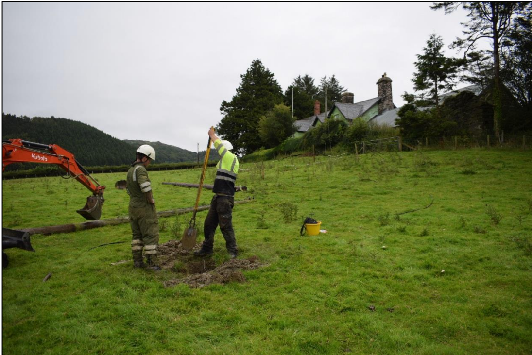
Fig. 5: Widening of the hole to allow the new pole to be inserted at the westernmost location (NGR SH 70380 00118), from the west-south-west. Photo CPAT 4386-0007.
