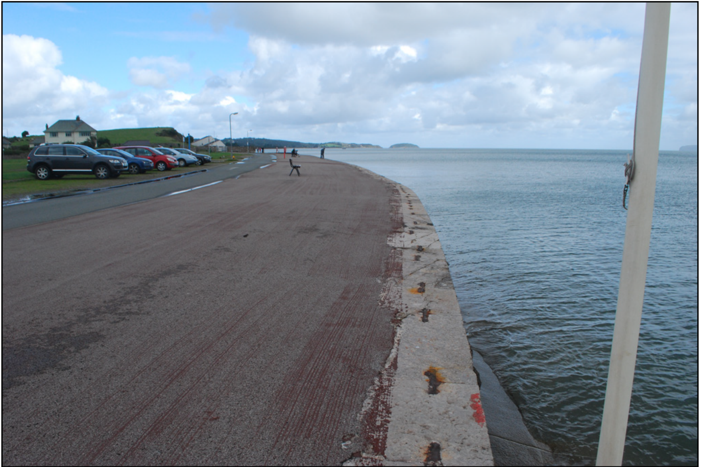
Plate 05 - View of the flood defence wall at the Green (Area 3, Feature 1). View from the south
