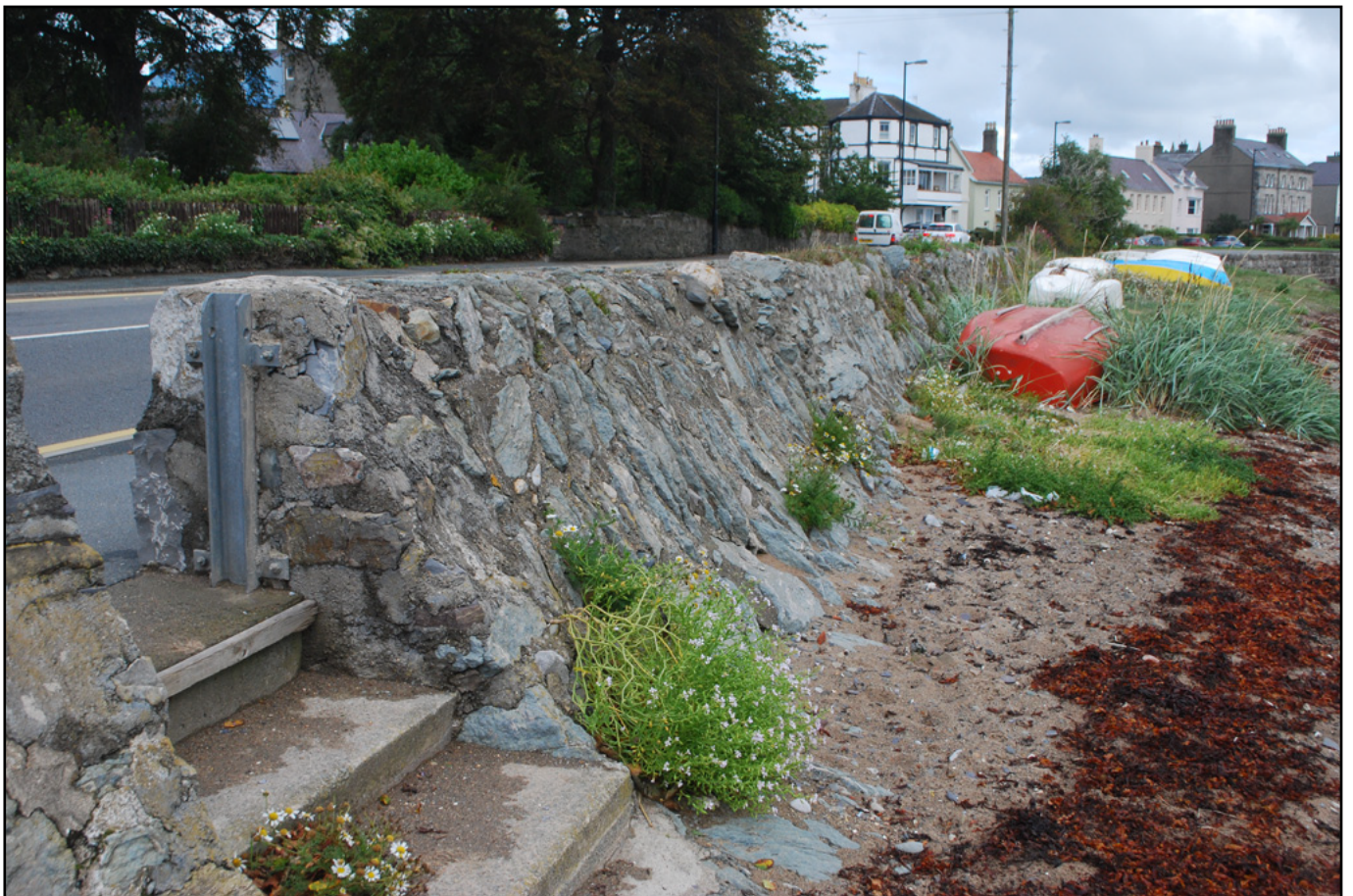
Plate 04 - Detail showing the batter on the flood defence wall in Area 4 (Feature 1). View from the north east
