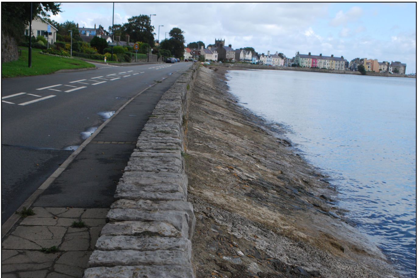
Plate 02 - View of the flood defence wall near Townend (Area 4, Feature 1). View from the south-east
