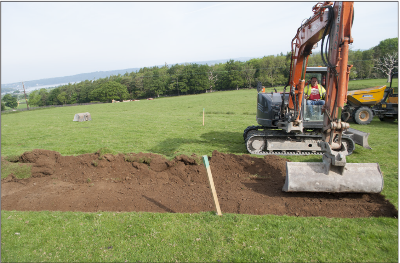
Plate 3: Working shot of topsoil strip; View from SE- scale: Not used. (archive reference: G2617_003).
