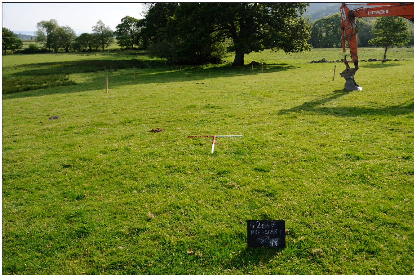
Plate 1: Pre-commencement shot of area to be topsoil stripped; View from SW - scale: 2x1m. (archive reference: G2617_001).
