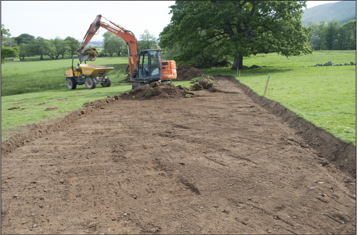
Plate 7: Working shot of turf/topsoil strip; View from SW - scale: Not used. (archive reference: G2617_007).
