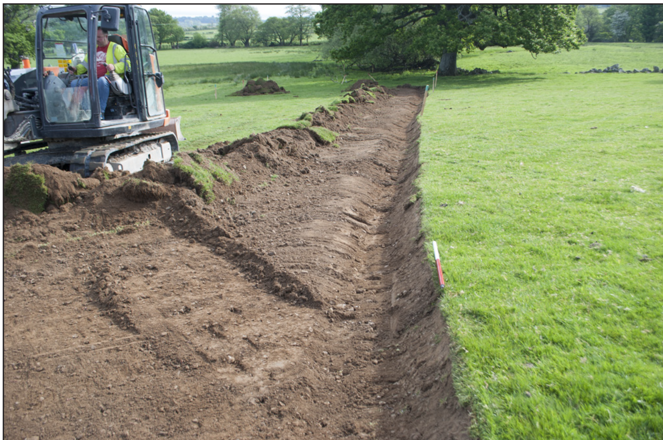
Plate 5: Shot of small drainage channel/v-ditch running length of track; View from SW - scale: 1x1m. (archive reference: G2617_005).
