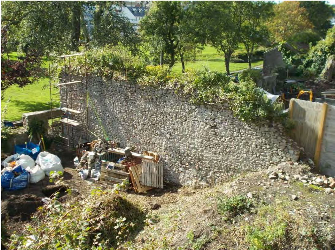
Photo 29: General shot facing SW, showing spoil heap in lower right-hand corner prior to removal.
