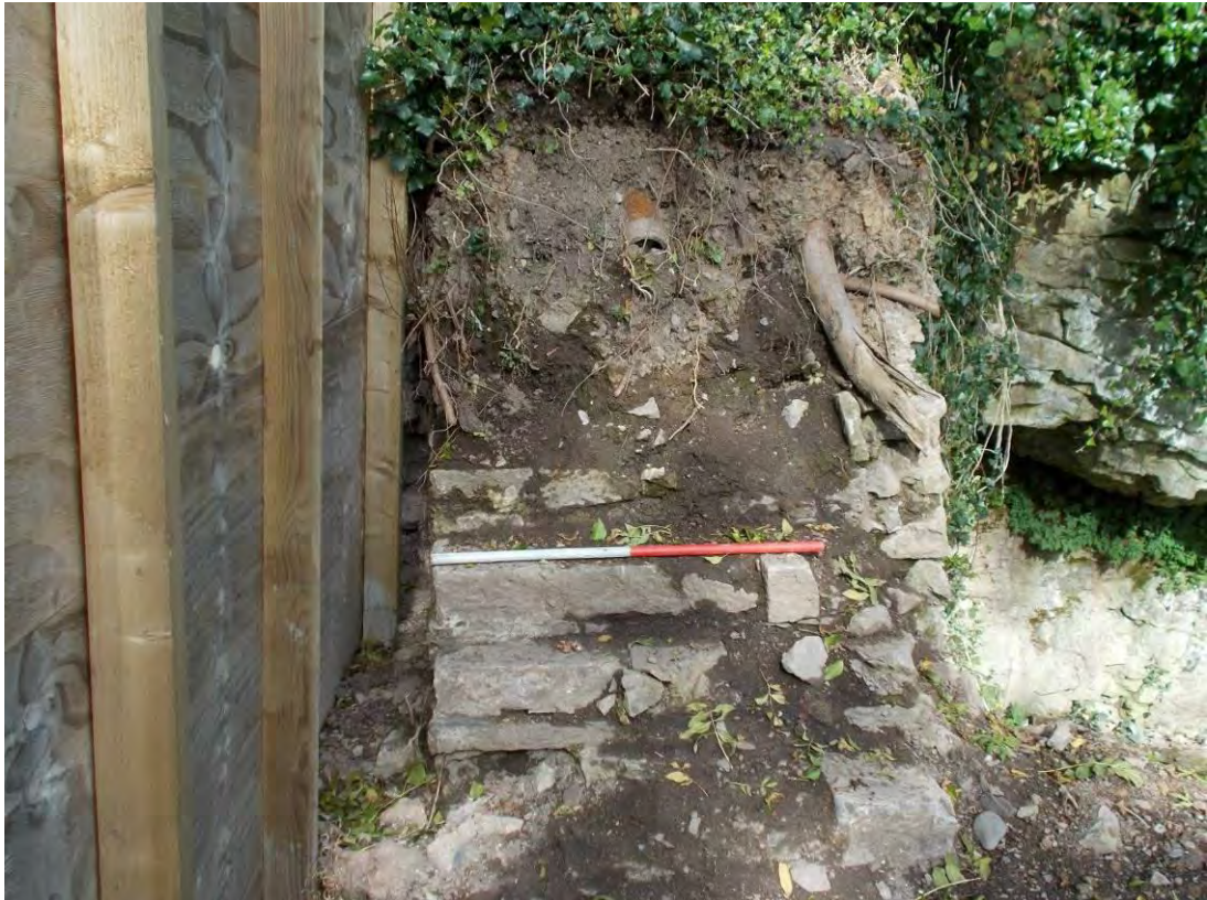
Photo 33: A series of steps between the two main levels on the site, built against the western boundary wall and partly uncovered. 1m scale.
