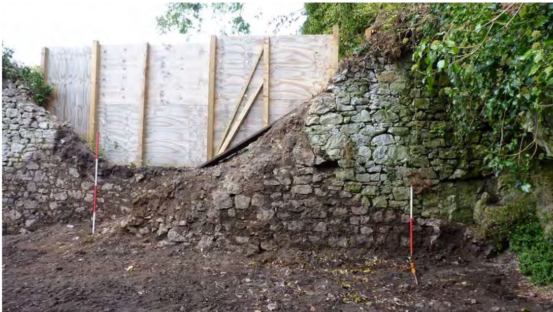
Photo 32: West facing shot showing western boundary wall after spoil tip was removed and spread. 2m & 1m scale.
