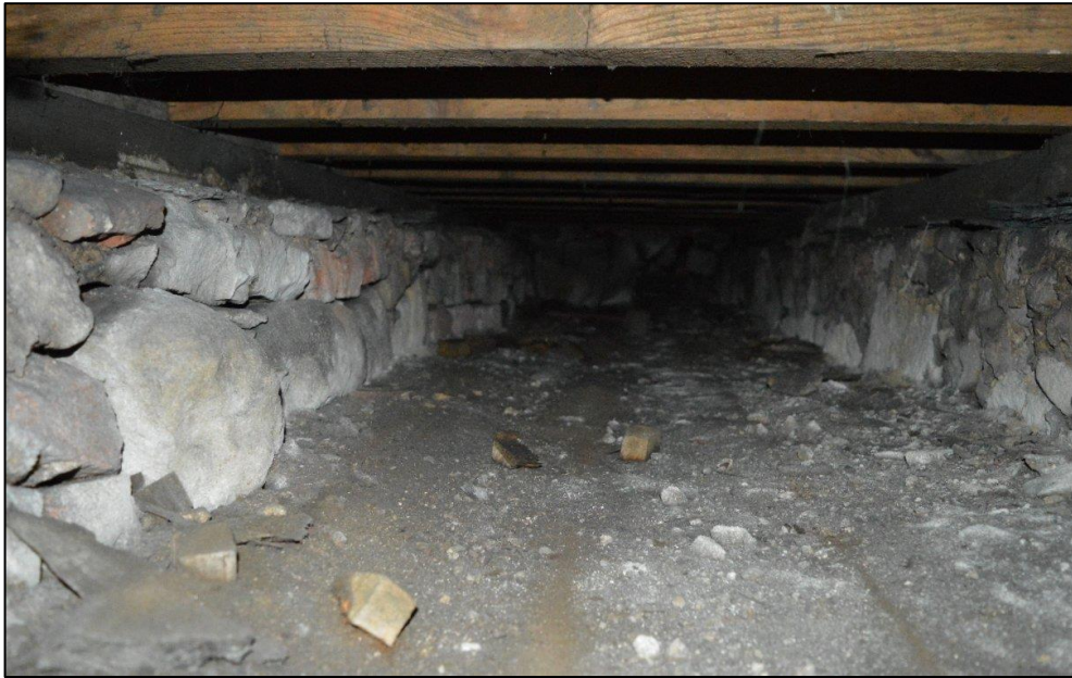
Fig. 3: The structure below the wooden flooring on the south side of the church, showing the possible earlier floor between the sleeper walls. CPAT 4283-0008
