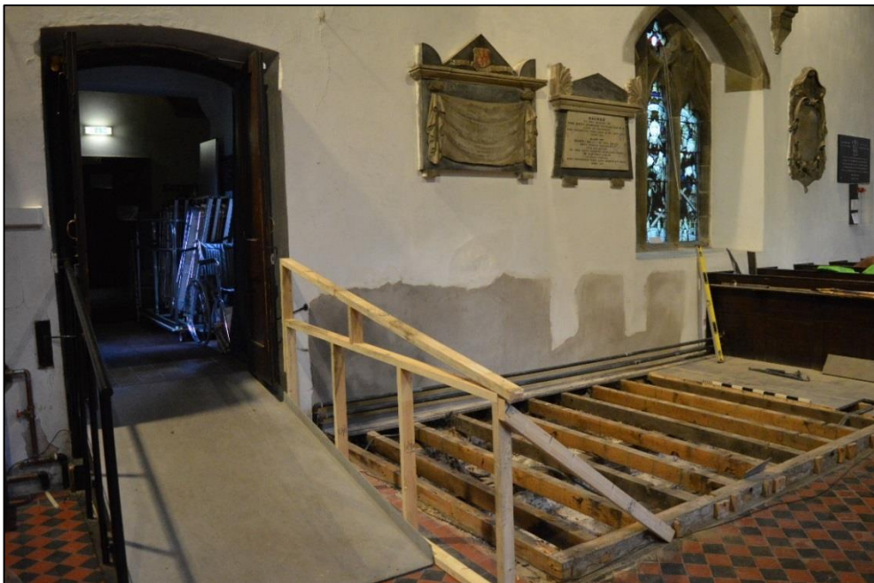
Fig. 4: The location of the new disabled access ramp after the pews and existing floor were removed, showing the adjoining tiled walkways. CPAT 4283-0010
