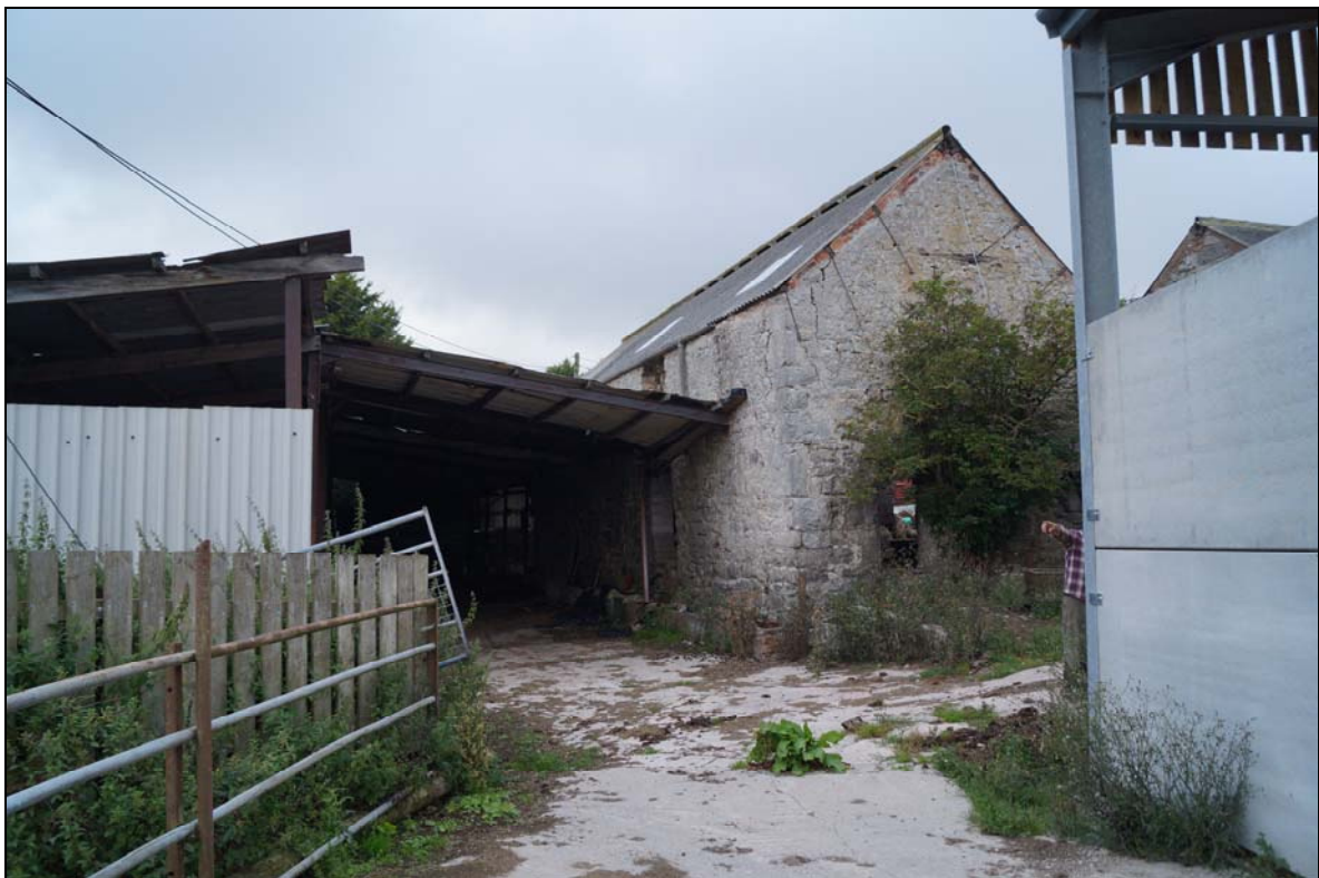
Plate 6: The eastern end of the listed barn (ID number 26), looking west northwest.
