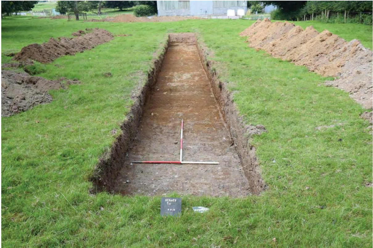
Photo 31: Trench 10, after machine excavation and initial cleaning. View Northwest. 2m & 1m scales.
