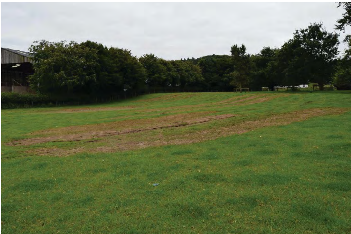
Photo 38: The Central Area after backfilling, looking Southeast. Showing the change of slope within the field.
