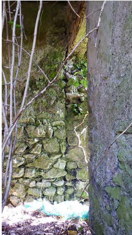
Photo 20: Interior of the outbuilding in the northeast corner of the site, showing both the inserted opening through the eastern boundary wall, and the northern boundary wall, which forms the rear of the outbuilding, butting against the eastern boundary wall.
