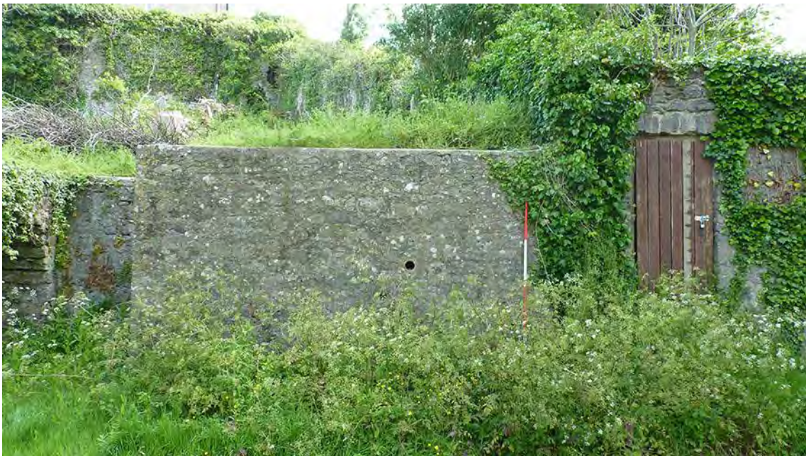
Photo 11: View NNE of the external face of the southern boundary wall, to the east of the limekiln. 2m scale.
