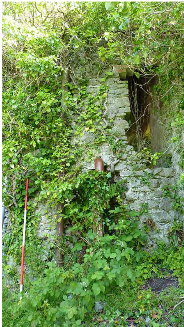
Photo 19: View NNE of the stone-built outbuilding in the northeast corner of the site, formerly used as a toilet as evidenced by the sewage pipe outlet. 2m scale.
