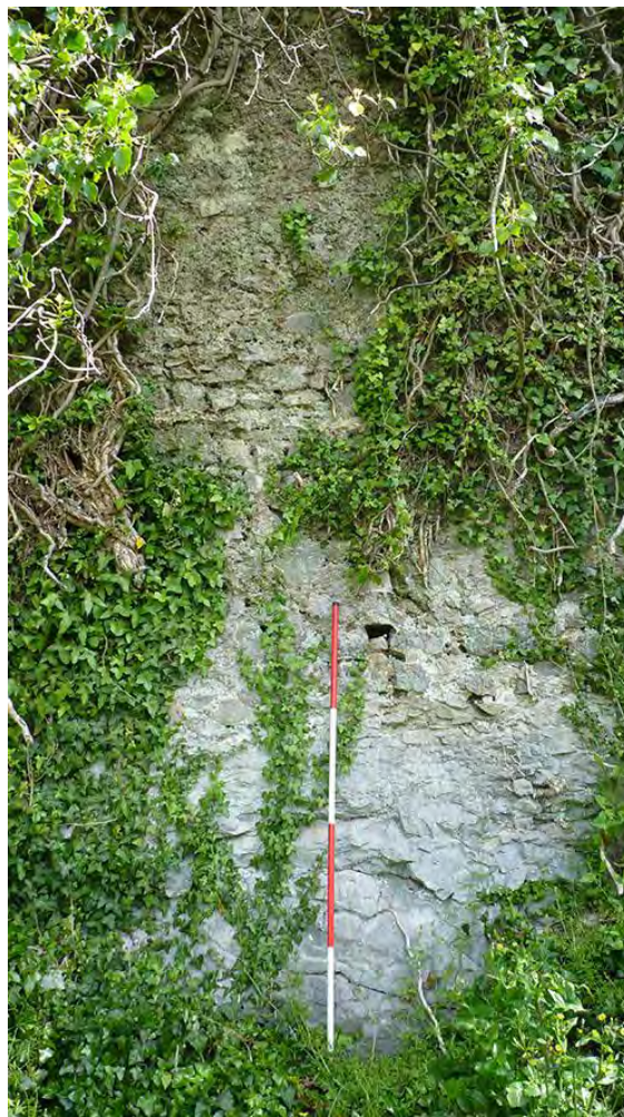
Photo 17: Central section of the northern boundary wall, showing the construction of the wall directly onto natural bedrock. 2m scale.
