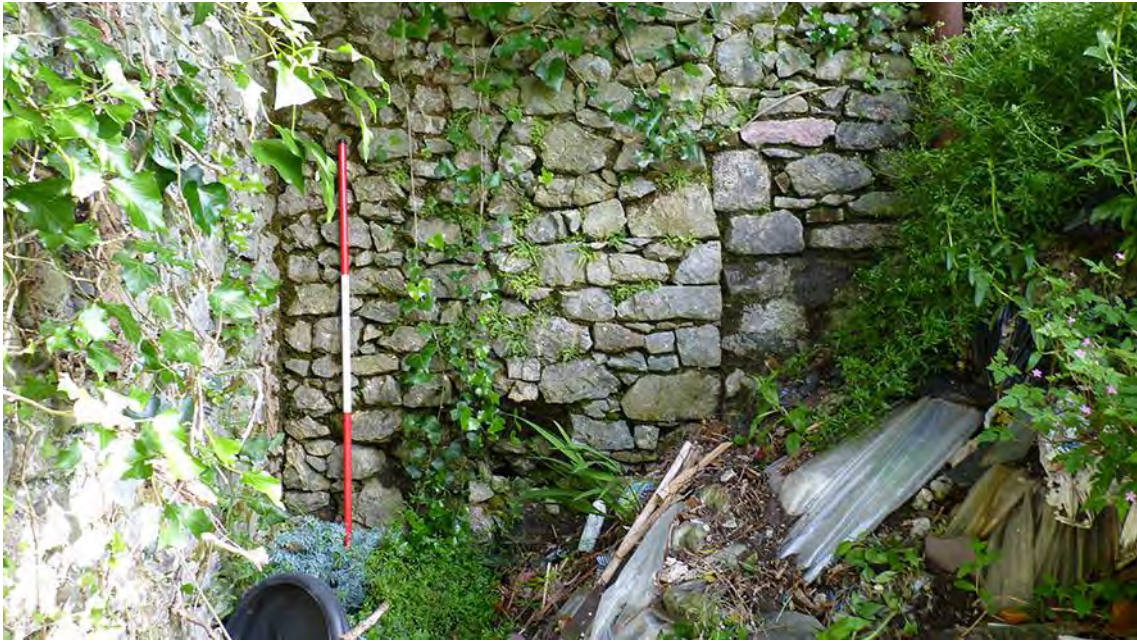
Photo 16: The western end of the northern boundary wall, showing both the butt-joint with the western boundary wall on the left, and potential blocking of an earlier opening seen in the vertical joint in the masonry on the right. 2m scale.
