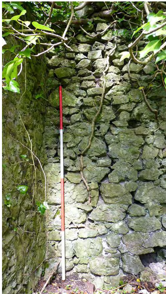
Photo 13: Inner face of the western boundary wall at the upper (northern) end of the site. 2m scale.
