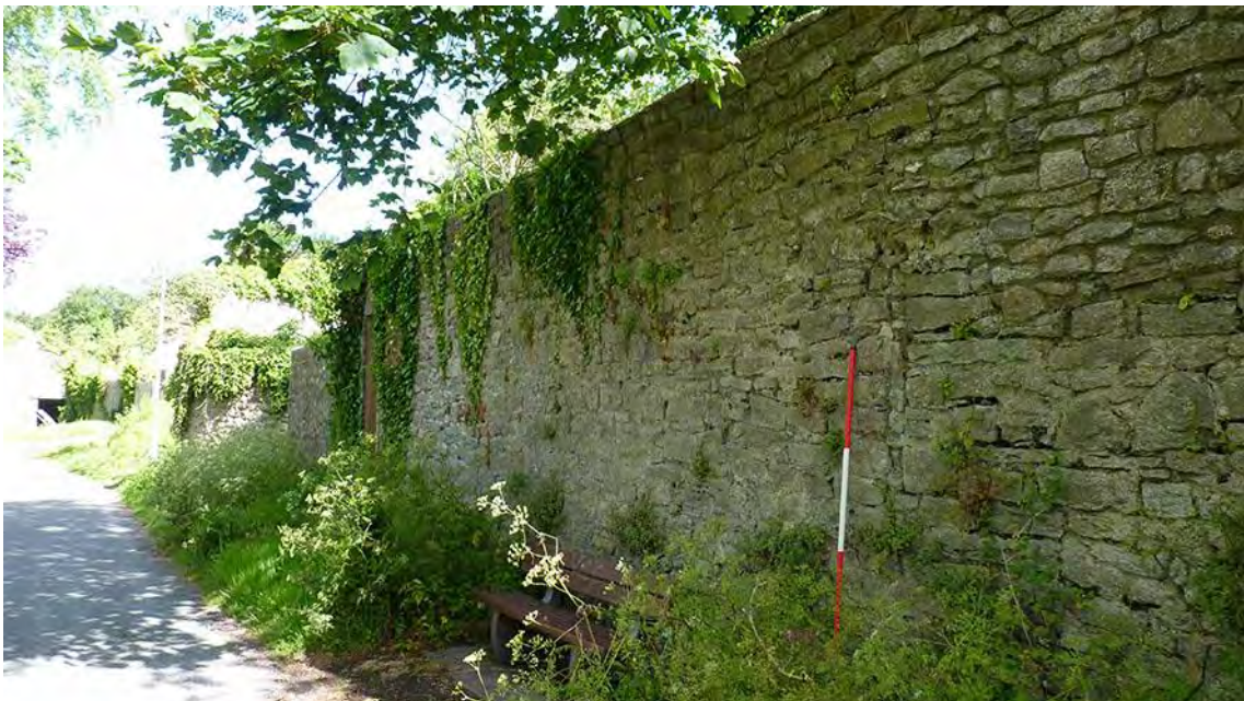
Photo 9: View WNW from the blocked arrow loop towards the site boundary wall (the projecting limekiln is visible). 2m scale.
