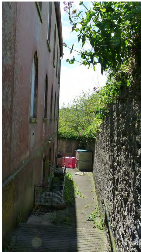
Photo 21: View SSW down the side of the Tabernacle Church showing the northern face of the upper reaches of the northern boundary wall (centre of photo).
