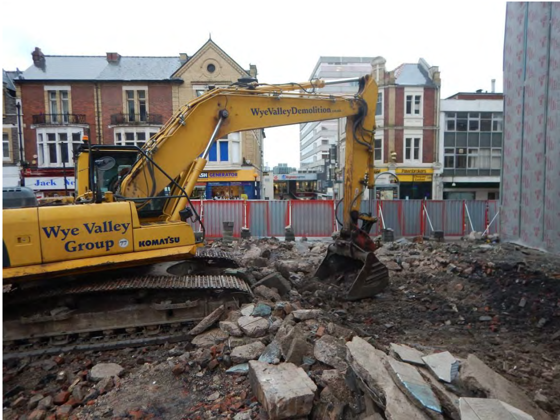
Photo 1: Initial clearance and excavation work in the area of Trench 1. View facing NE.
