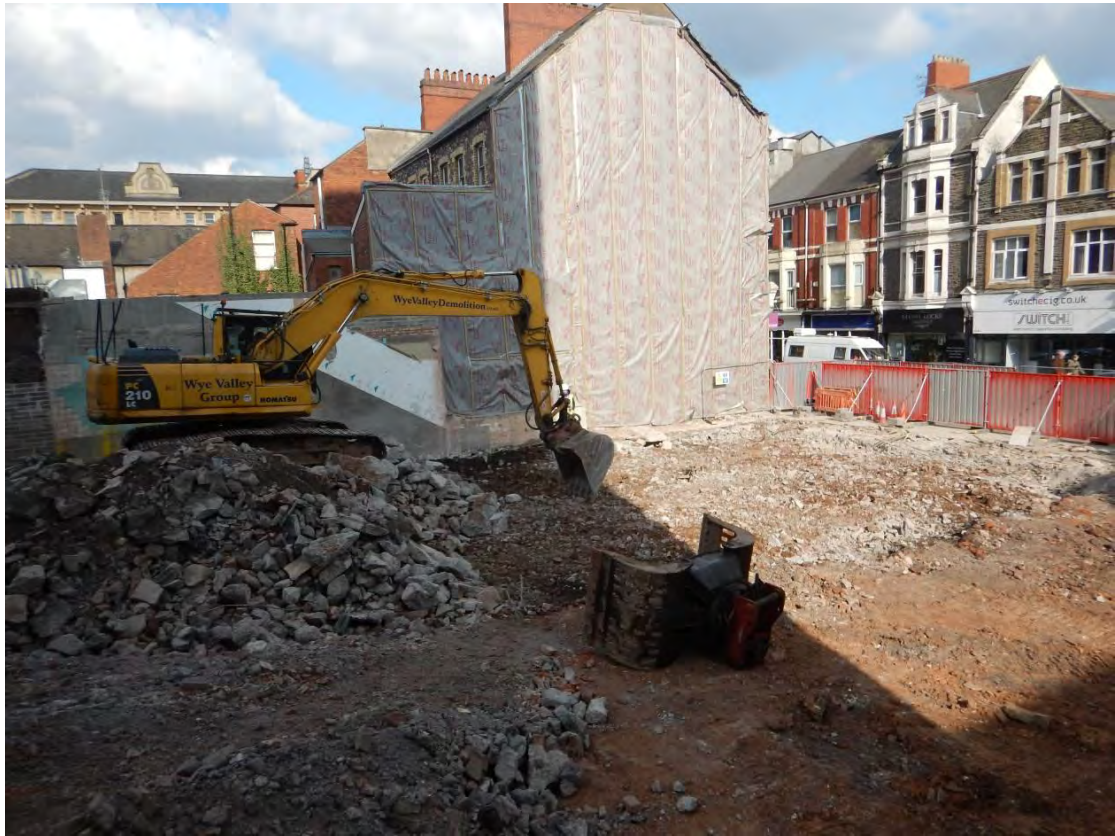
Photo 3: Initial excavation and clearance work in the area of Trench 2. View facing north.
