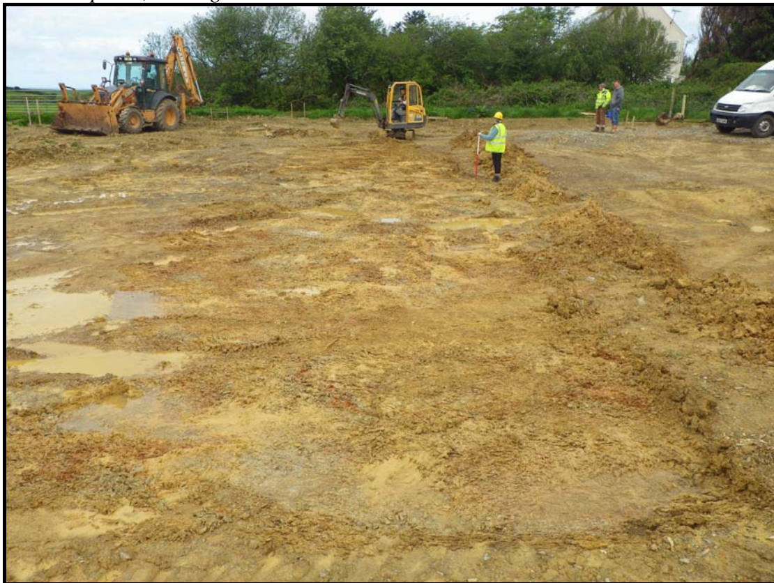
Plate 4: PZC2014_104, Mechanical cleaning of area in which foundation trenches would be excavated, looking west southwest.
