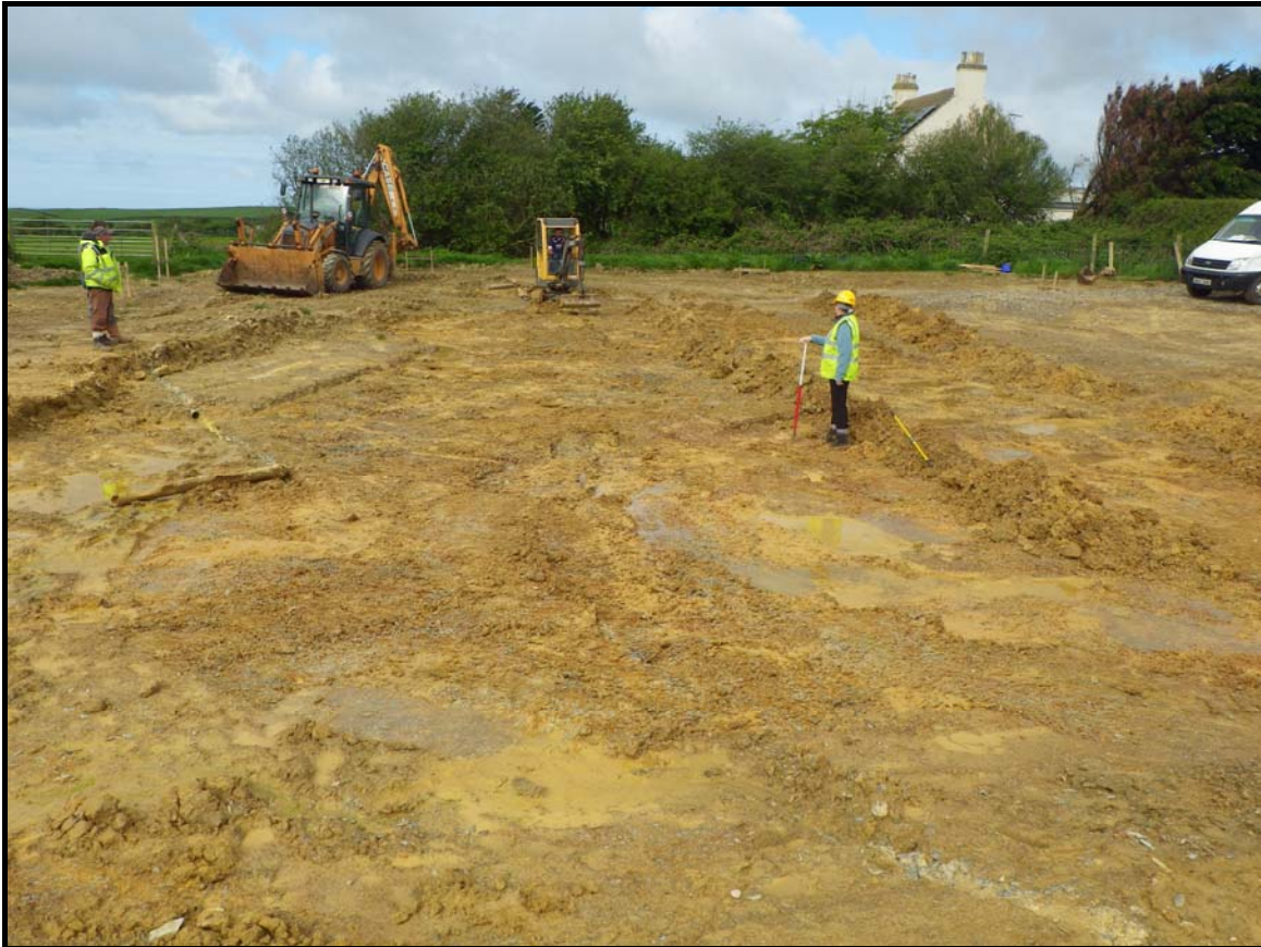
Plate 5: PZC2014_105, Mechanical cleaning of area in which foundation trenches would be excavated, looking west southwest.
