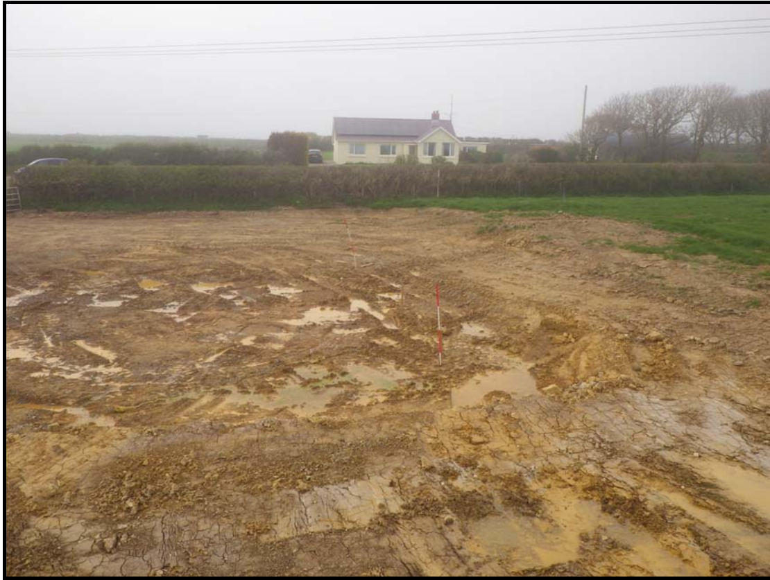
Plate 3: PZC2014_103, Area from which topsoil was removed prior to the watching brief with subsoil exposed, looking north northeast..
